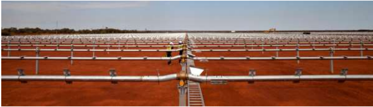
Figure 3-2 Example of a single-axis mounting system before panel installation.
