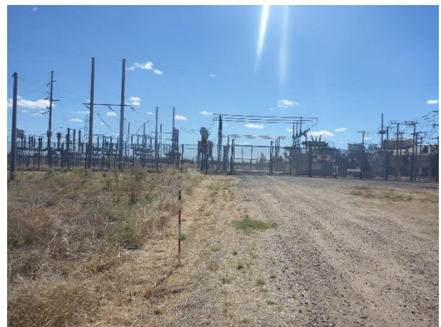
Plate 10 View east to existing substation structure.
