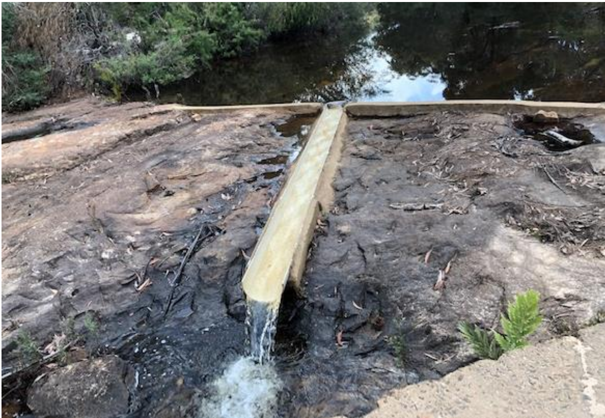
Plate 1 – Example of half-pipe weir structures installed at surface flow monitoring sites in Areas 5 and 6
