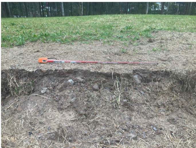
Figure 5-6: The sinkhole located to the southeast of the data centre building. Located within SU-01, facing west.
