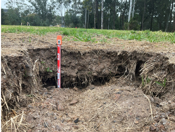
Figure 5-7: Section of the sinkhole to the southeast of the data centre building, showing the soil profile. Located within SU-01, facing southeast.
