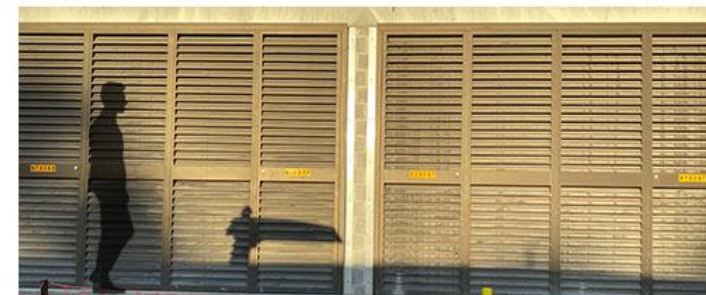
Ventilation louvres on the front of a chamber substation
