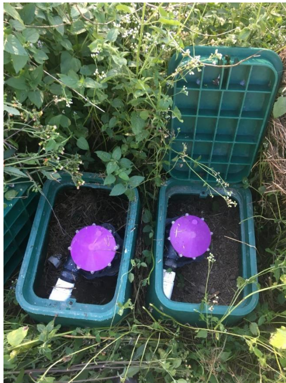
Photograph 8: Indexing valves in irrigation boxes.
