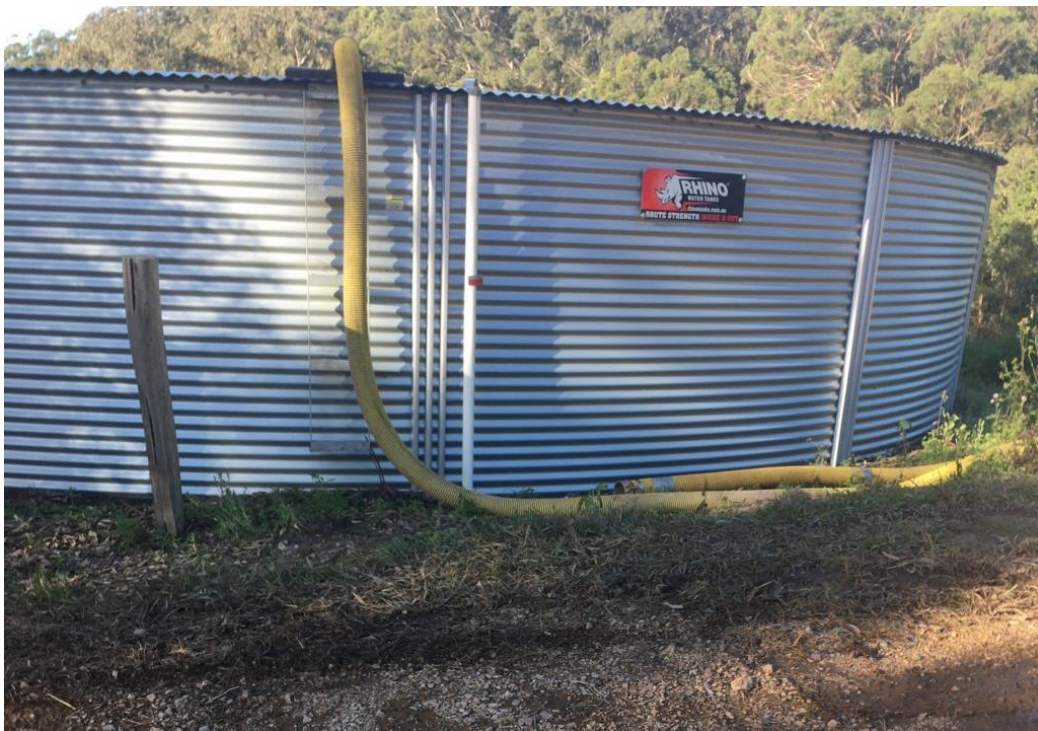
Photograph 6: Wastewater long-term 230kL holding tanks with transfer hose connected.
