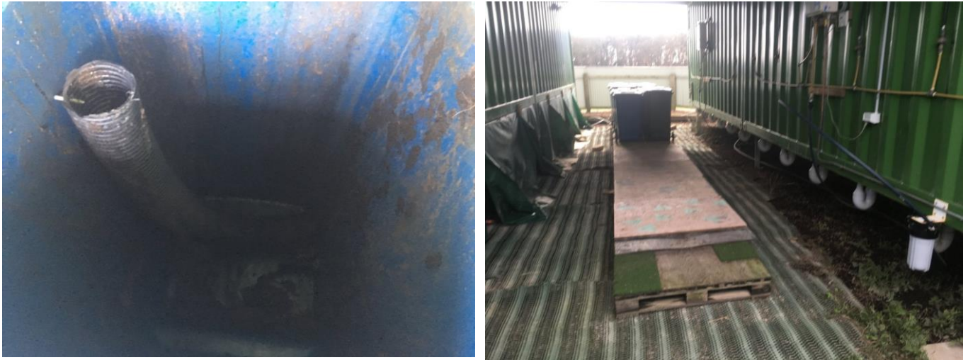
Photograph 3: Wheelie bins internal venting pipe, and storage area.
