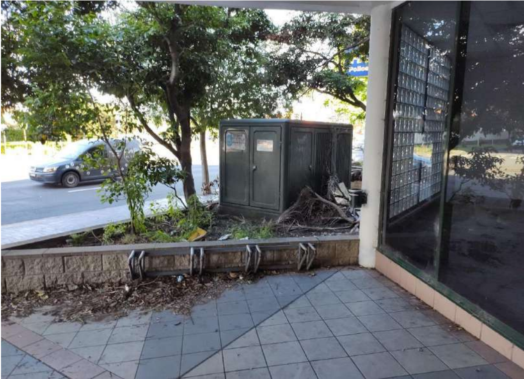
Photo 5: Transformer near southern boundary of site
