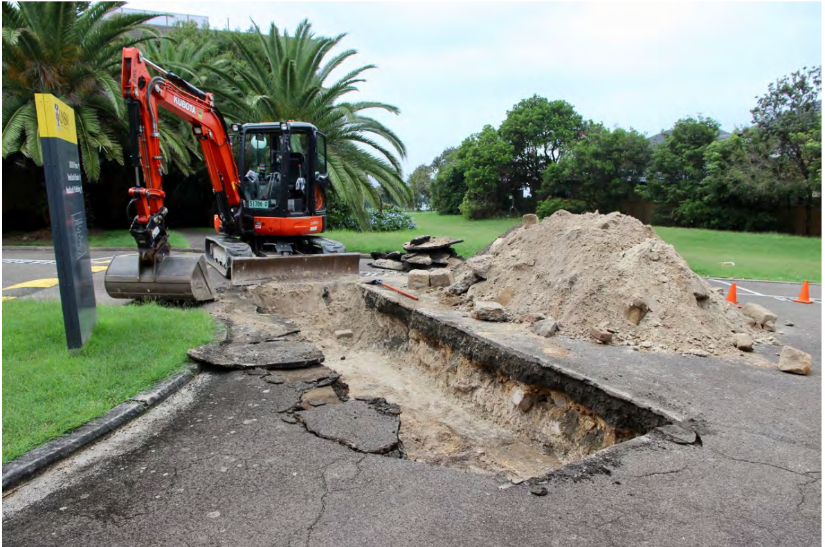
Figure 99: TT4 - Removal of construction & demolition deposit (with in situ footings exposed at base)
