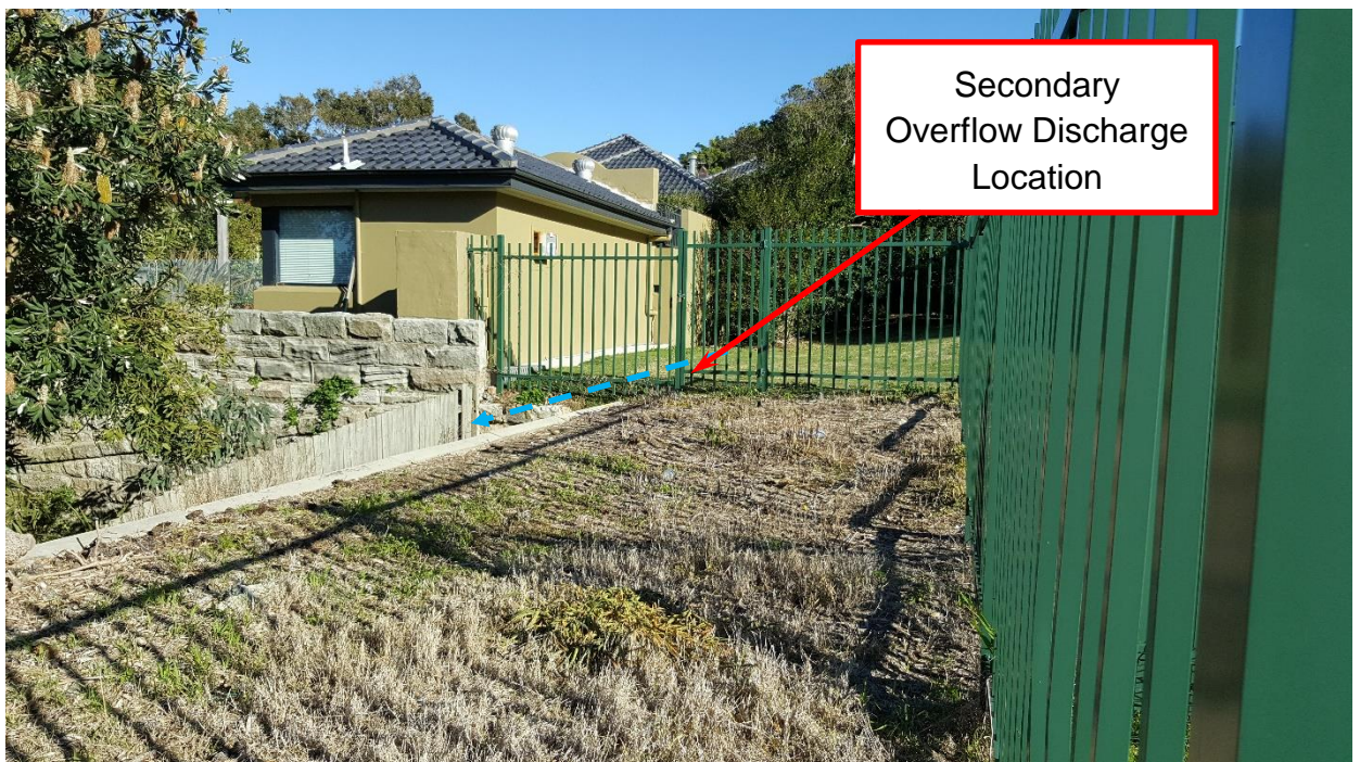
Figure 22 – Western view of secondary overflow path discharge point from Site, along southern boundary crib wall
