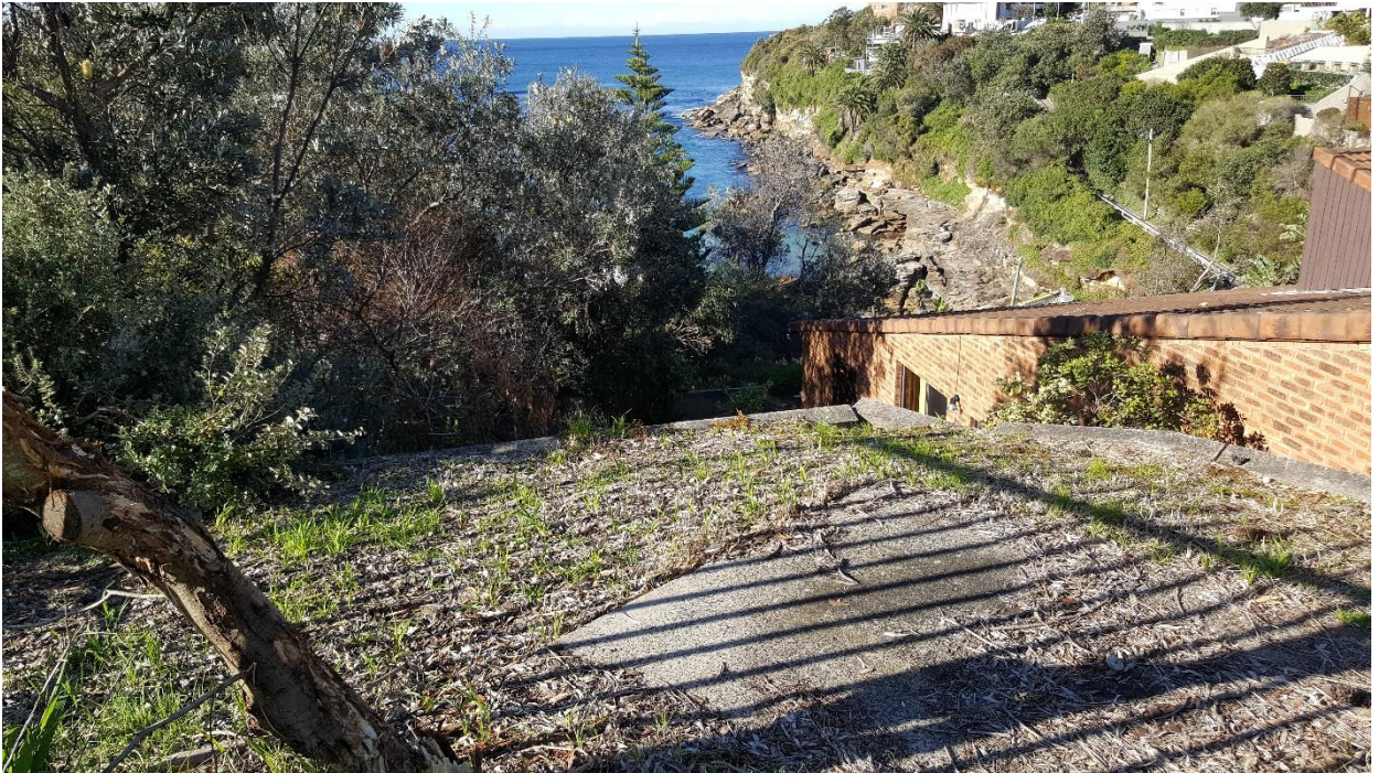
Figure 23 – Eastern view near secondary overflow path discharge point from Site, along southern boundary crib wall
