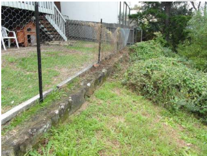
Figure 13. Property edging and footings are likely to have been carved from outcropping sandstone in the eastern third of the property.
