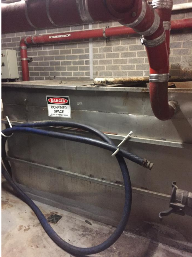
Photo 6: 1 of 3 grease traps located in basement level 1
