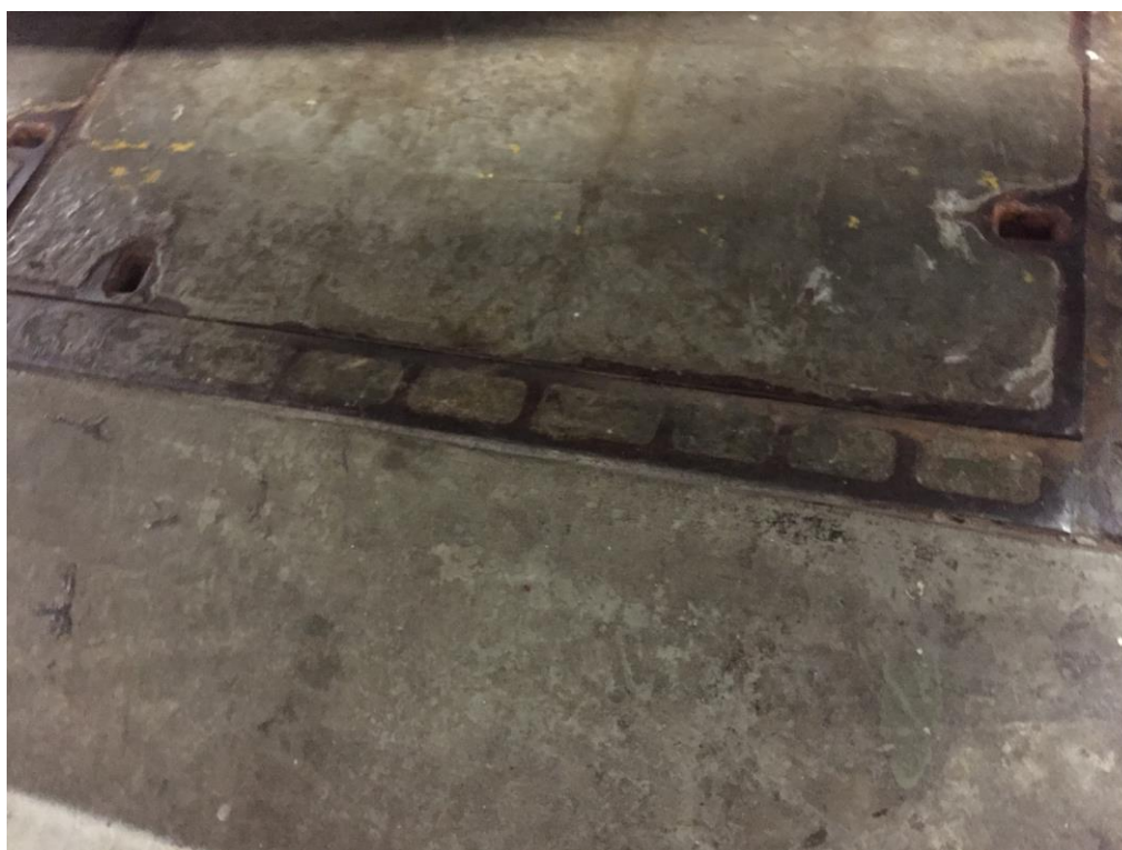
Photo 2: Underground Storage Tank 2 - Basement Level 2
