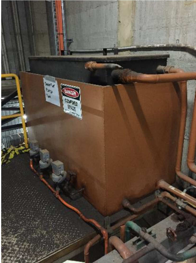
Photo 8: Day tanks holding diesel from underground storage tanks for back up generators on level 40
