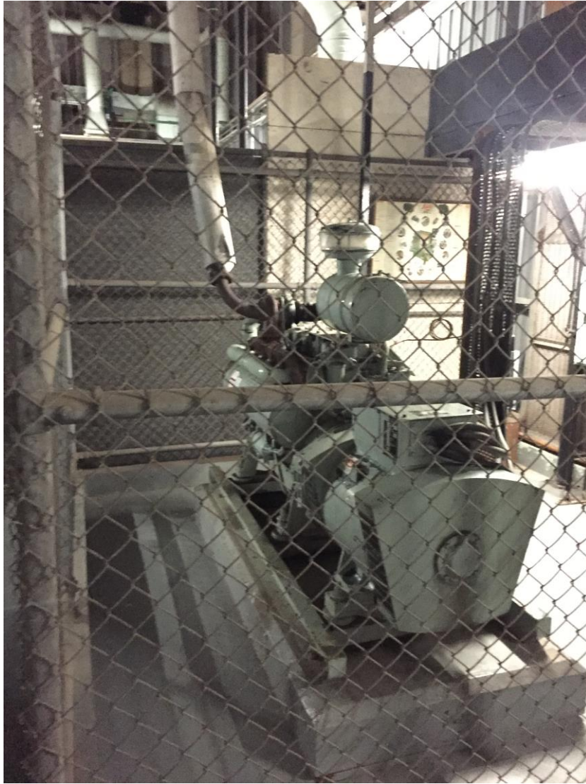
Photo 9: Back up generator on level 40
