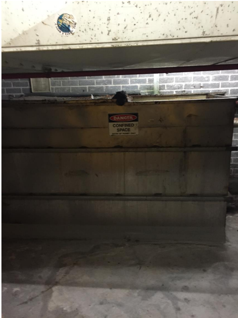
Photo 7: 1 of 3 grease traps located in basement level 1
