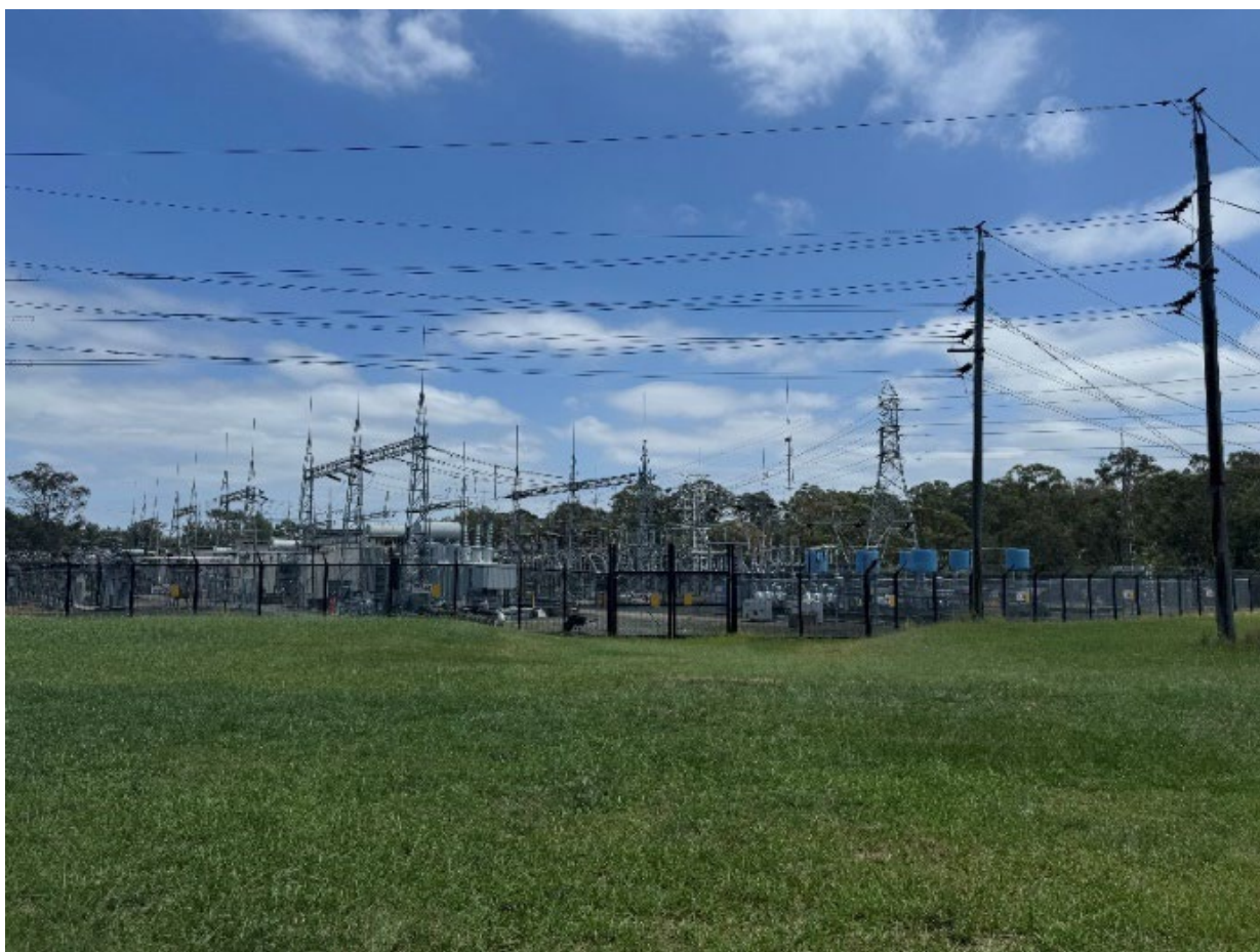
Photo 2-6: Looking west onto Baulkham Hills Transmission Substation
