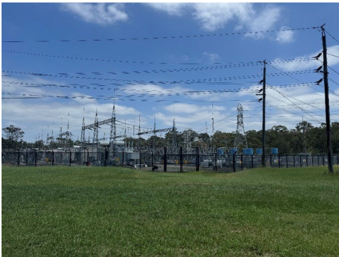
Photo 2-2: Looking west onto Baulkham Hills Transmission Substation
