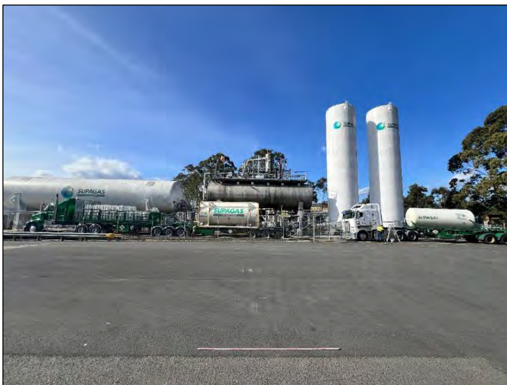
Plate 10: Existing CO2 facility within Manildra similar to the proposed new CO2 facility.
