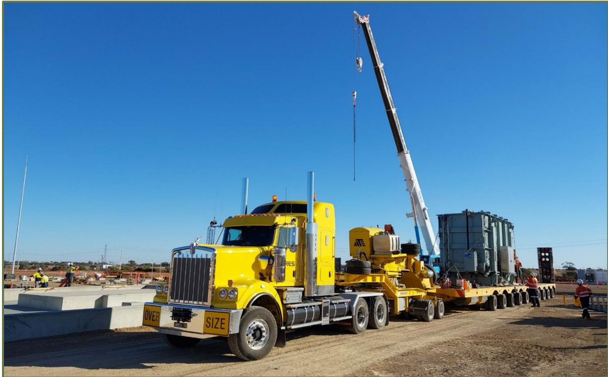
Figure 1 Anticipated Transformer and the Nominated OSOM Vehicle
