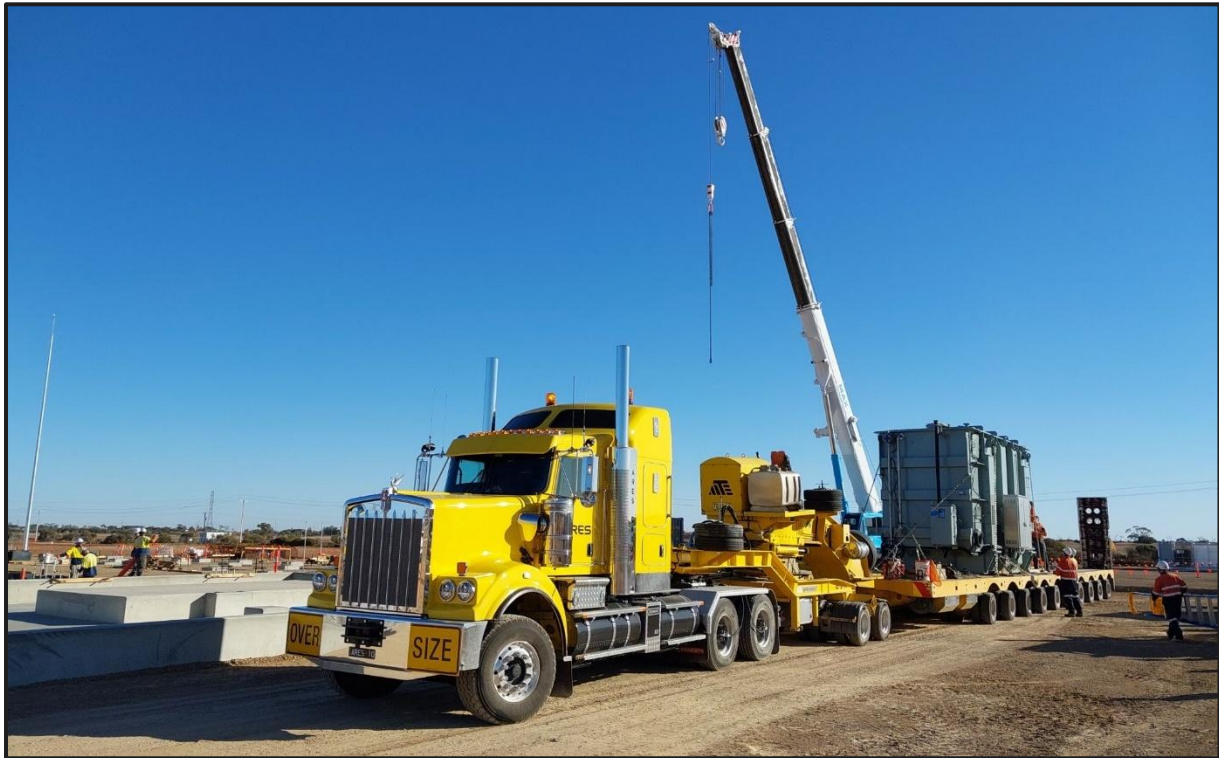
Figure 5 Anticipated Transformer and OSOM Vehicle (Similar)
