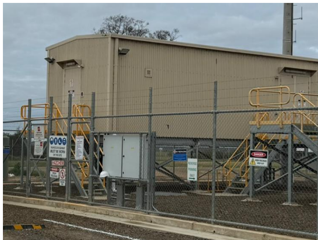
Figure 7 Image of switchroom (source: Stor)
