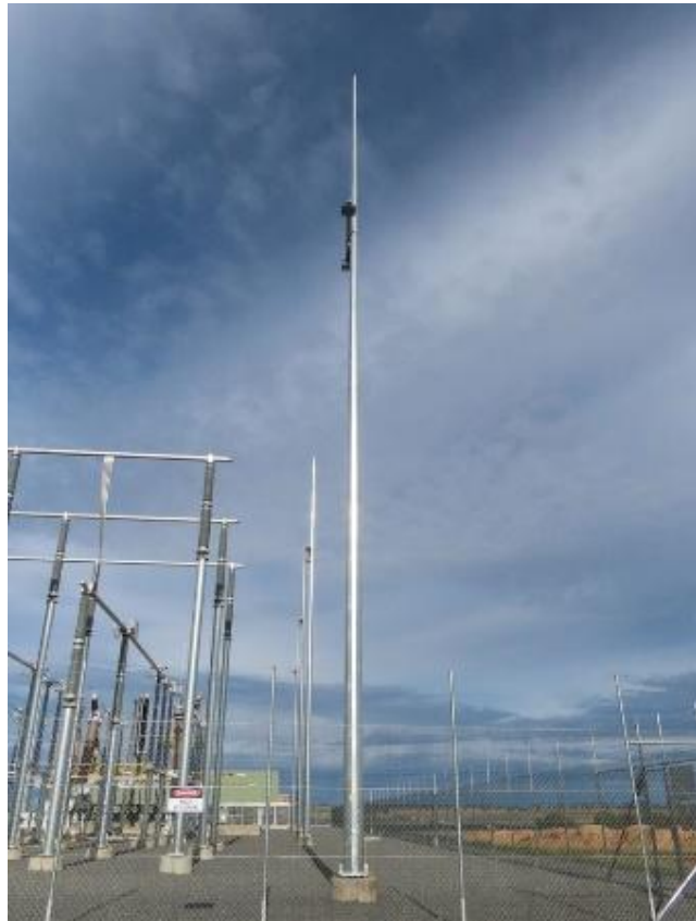
Figure 6 Image of lightning masts (source: Stor)
