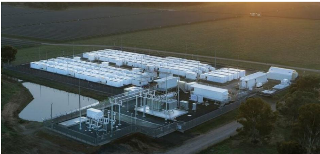
Figure 3 Indicative Image of BESS Modules
