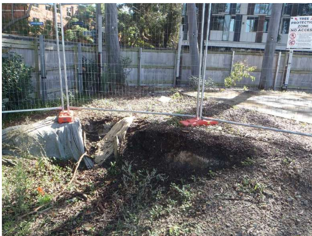
Figure 41. Close up views (both photos) of the trunk and ground condition of trees T43, T42 and T41 (from left to right). Note: T44 just out of the photo on the far left. Photo looking north (Danks St straight ahead). Note retained slab (semi-circle) and understood to have the underground arrangement described in Figure 5 (Chapter 6). Retain TPZ fencing in place for the Main Works DA / construction phase and for tree stability (utilising the slabs for stability)
