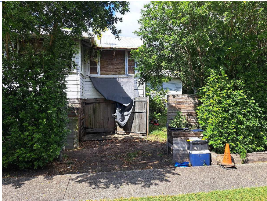
Photo No. 1 Date 17.10.2024 Description: View south overlooking existing weatherboard dwelling to be demolished on 12 Florence Street.
