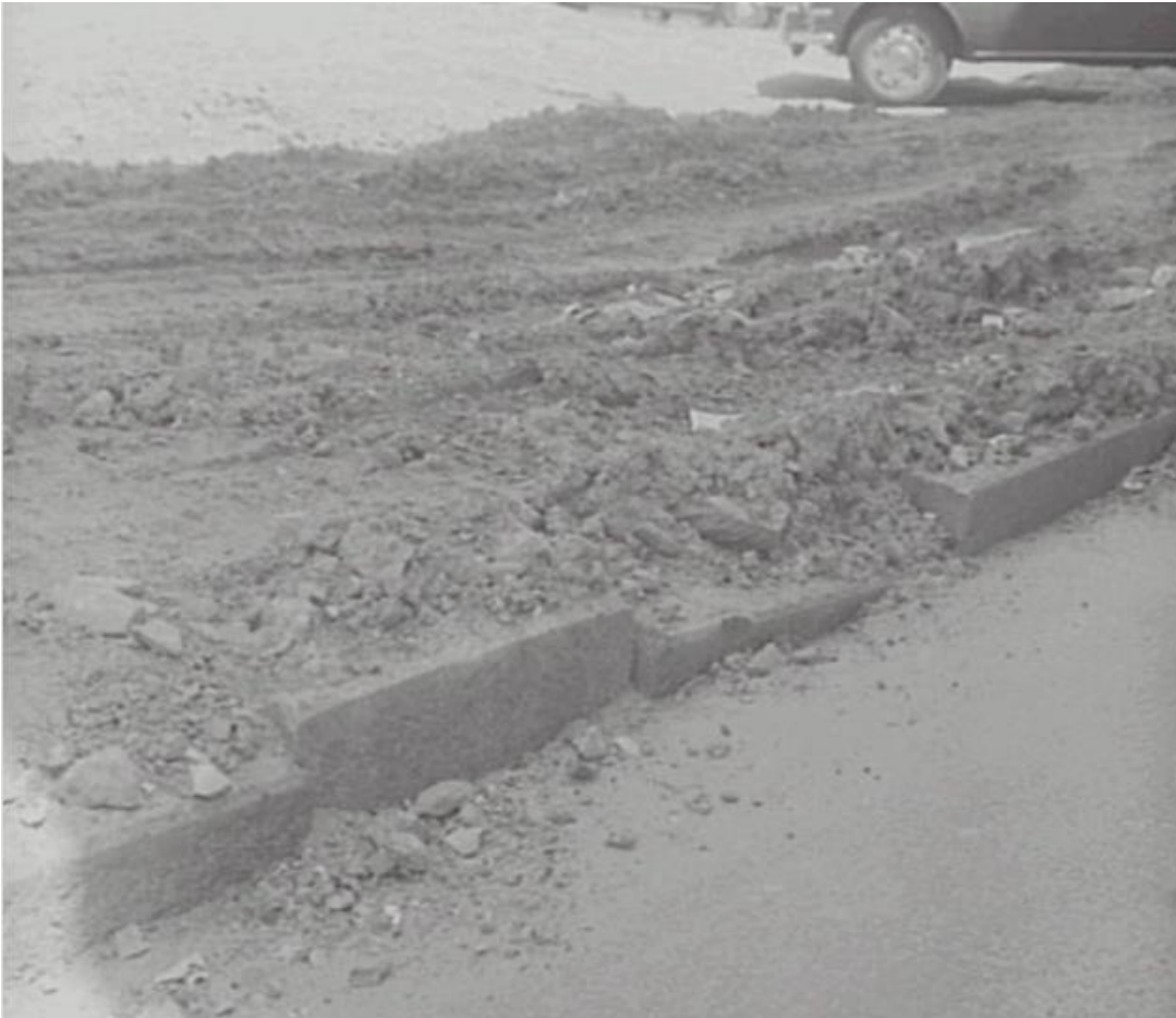
Figure 24 – Footpath damage in Judge Lane, Woolloomooloo, 1971. Detail of possible remains of former terraces either in situ or as reused materials.
