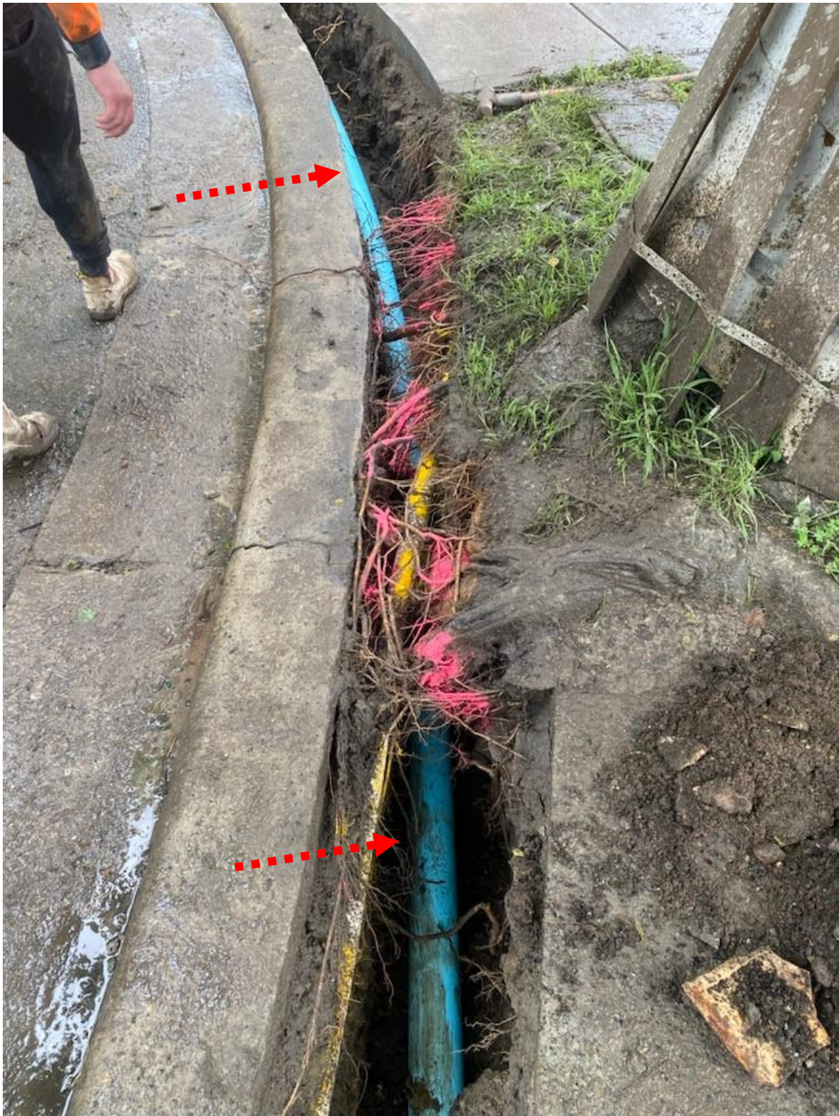
Roots have been exposed and painted to highlight location so that services can be placed underneath tree roots without impact to tree roots
