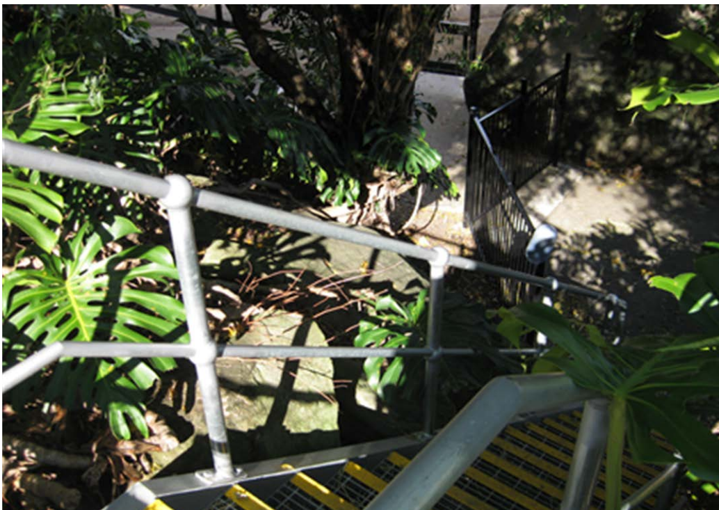
Photo 10 – Floater exposed near stairs
