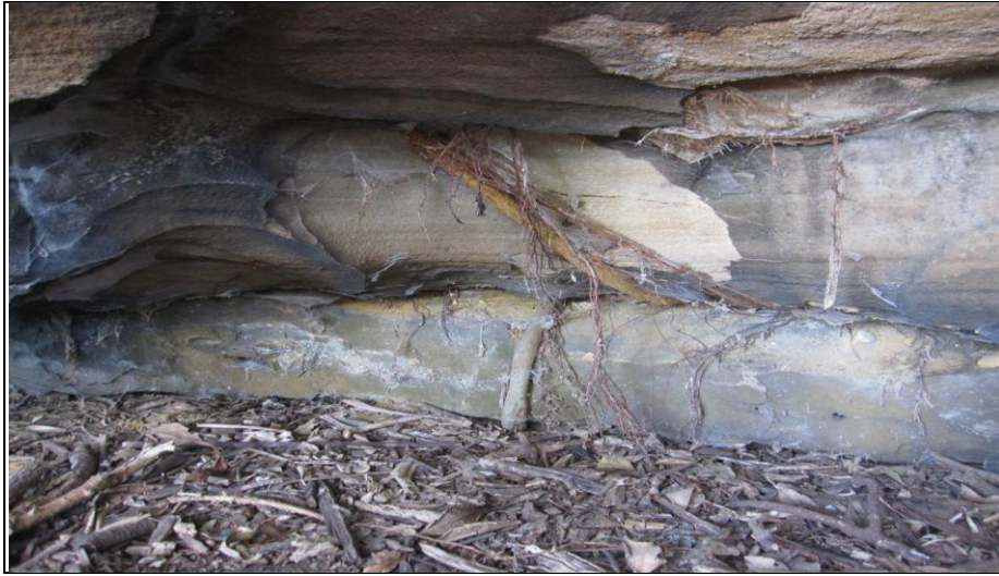
Figure 2.8: The probable location of the above photo; this area of stone below the tree roots is deteriorated (Rice 2016)
