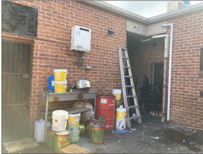
Photograph 5 – Rear View: Waste Drums and Containers of Food Supplies
