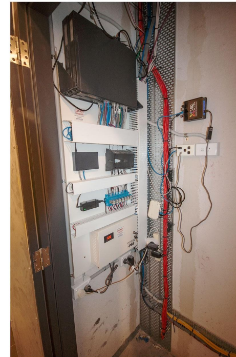
A typical on-floor communication cupboard
