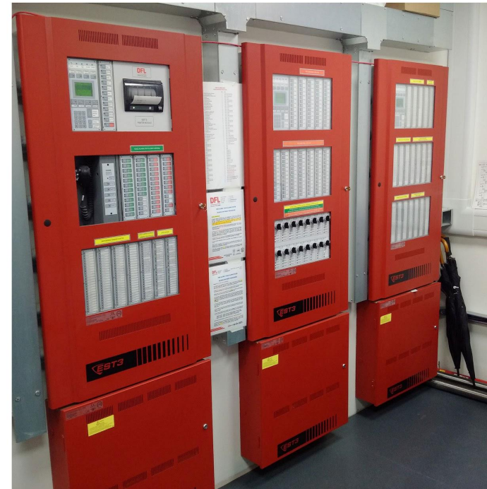
Fire alarm control panel
