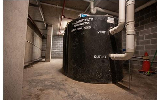
An image of an installed grease arrester
