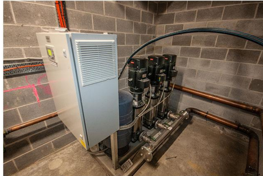
Cold water booster pump room image.
