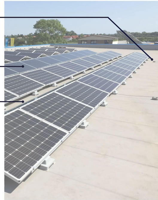
A typical solar panel arrangement (image source https://www.sika.com/ )
