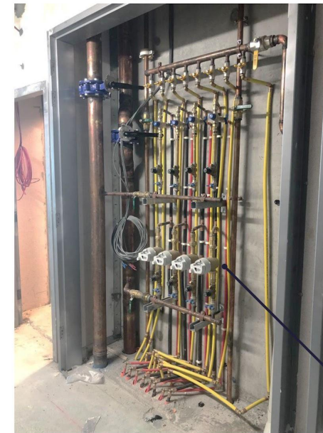
A typical on-floor hydraulic cupboard
