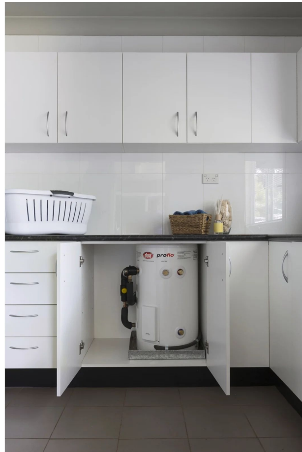
Electric storage unit
