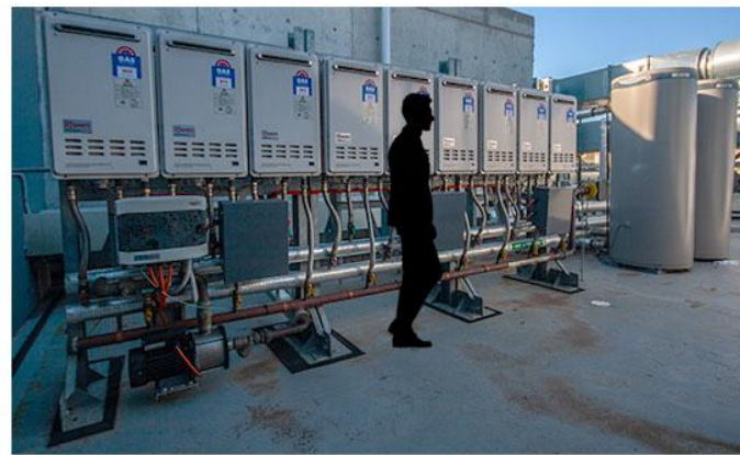
An Image of hot water heaters located outside on a roof
