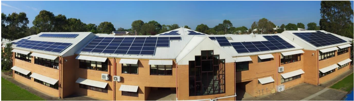
Example of a large 99.5kW solar system at Menai High School.
