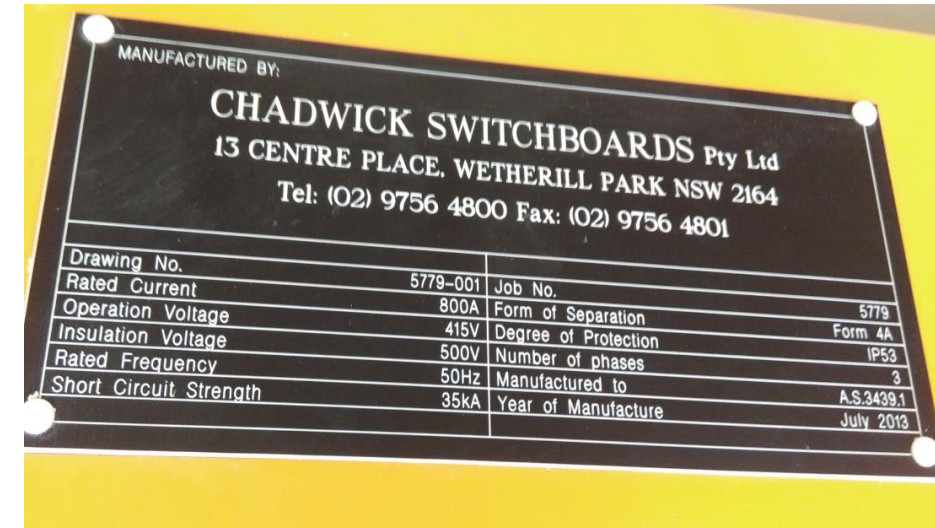
Figure 3: Existing Site MSB
