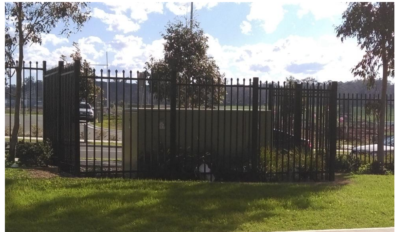
Figure 1: Existing Kiosk Substation S.32635
