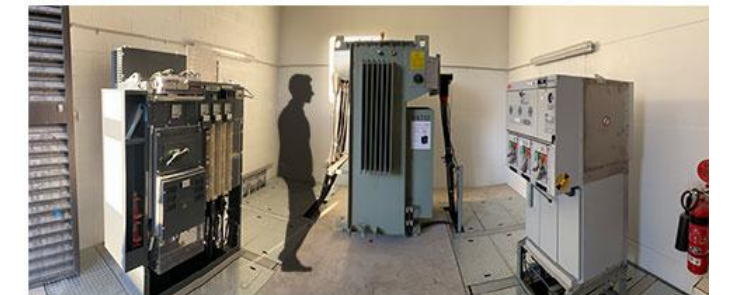
Inside a chamber substation
