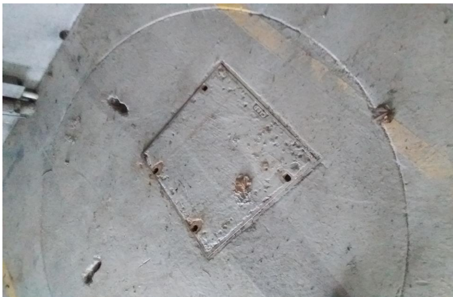
Photograph 8 – The water sump observed in the basement of premises 270
