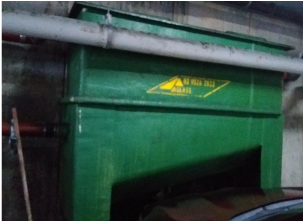
Photograph 7 – Aboveground grease trap located in the basement of premises 270
