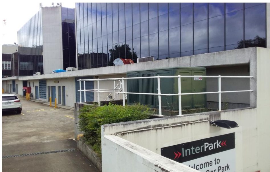
Photograph 5 – Green electrical transformer located at the rear of premises 270.
