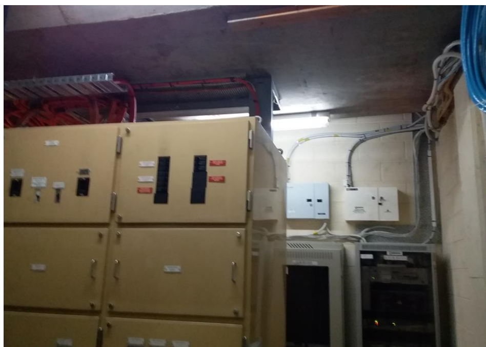
Photograph 6 – The plant room observed in a shared basement.
