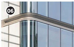
06 Podium Glazing Clear Low E Igu With Spandrels Panel In Light Bronze Finish
