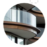
06. TOWER BALCONY CLEAR GLASS BALUSTRADE, SLAB EDGE TOP AND BOTTOM PROFILE TO MATCH LIGHT BRONZE METAL CLADDING
