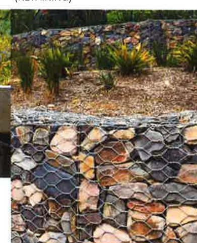
BLUE STONE GABION WALL (RETAINING)
