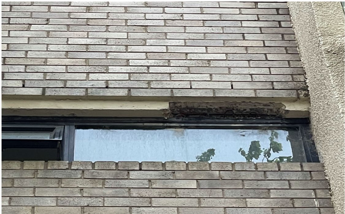
Figure 7 - Spalling concrete at façade / primary structure interface. Primary structure is supporting brick façade. Poses a very significant safety risk due to concrete pieces falling without notice to ground.
