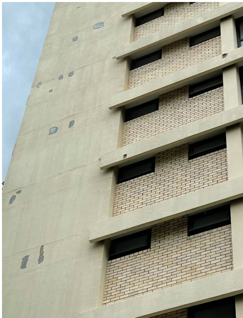
Figure 10 - Elevation of façade showing previous repair of concrete elements. If this building was to remain, it would require constant repair and maintenance of the external building fabric. This maintenance would not stop safety concern, but rather be required for the building to remain serviceable. This repair would require concrete and steel removal and reinstatement. These works would likely require scaffolding to be erected around the perimeter for long periods and cause significant disruption to the residents and public.
