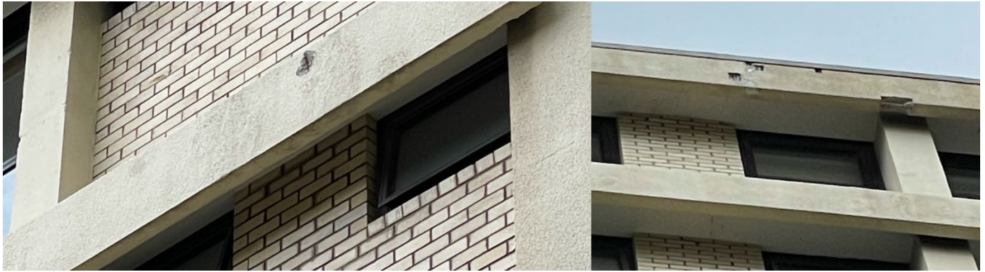
Figure 9 - Additional locations of spalling of external concrete façade elements. Poses a very significant safety risk due to concrete pieces falling without notice to ground
