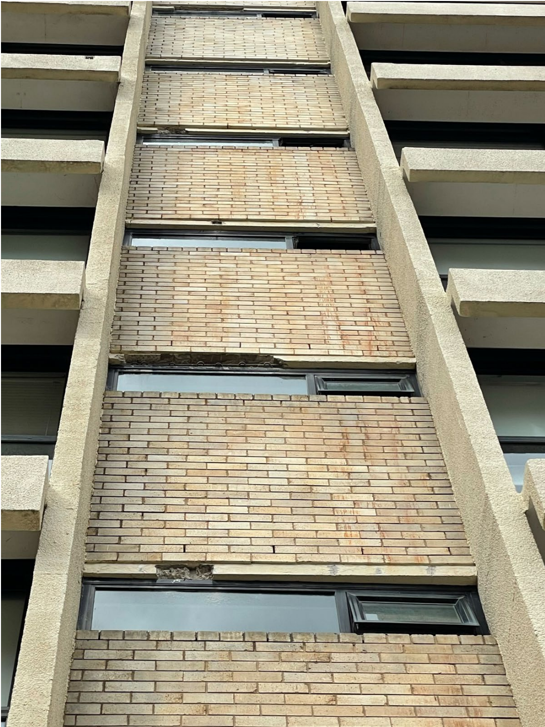
Figure 8 - Elevation shot showing extent of building damage. In this location all but one floor has been affected by concrete cancer (or evidence of it).
