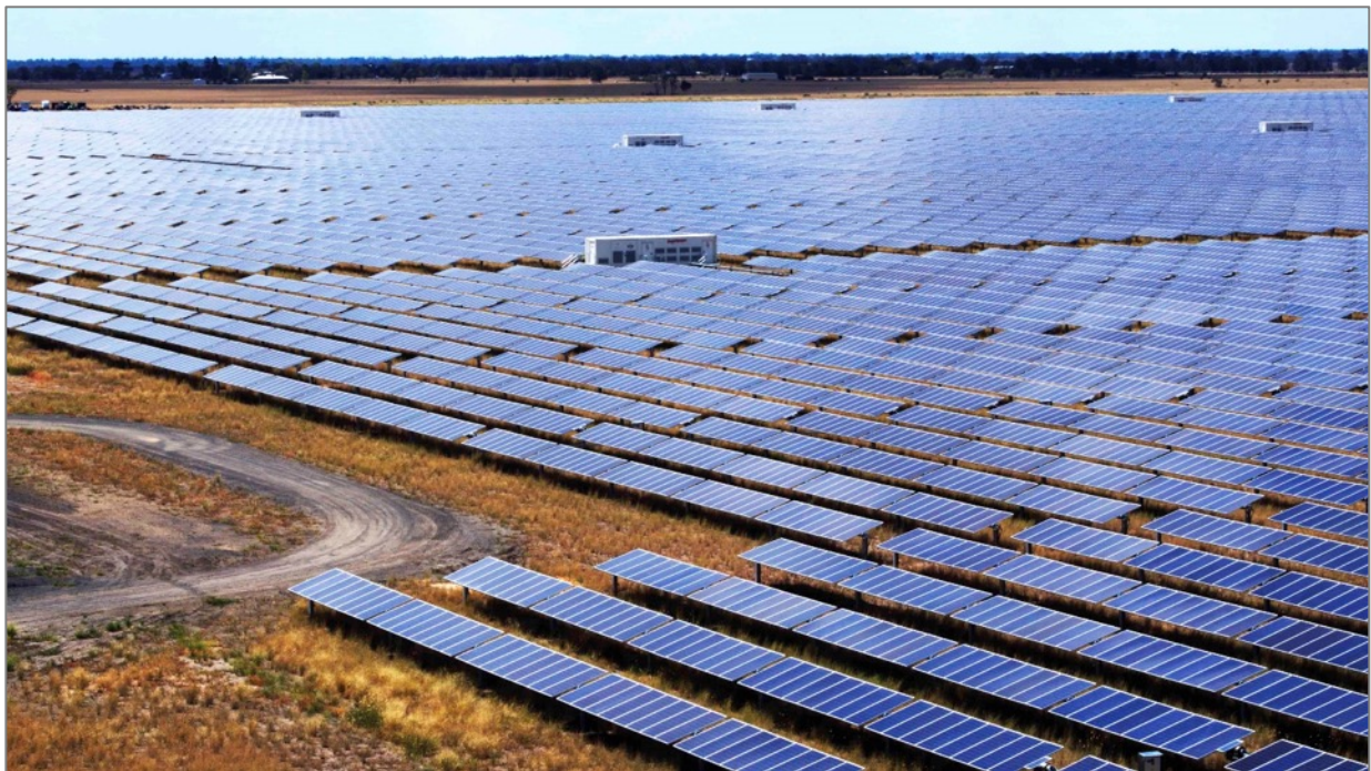
Figure 3-2: Fully assembled tracking array solar farm showing inverter housing (image courtesy Nextracker Australia, actual system may differ).
