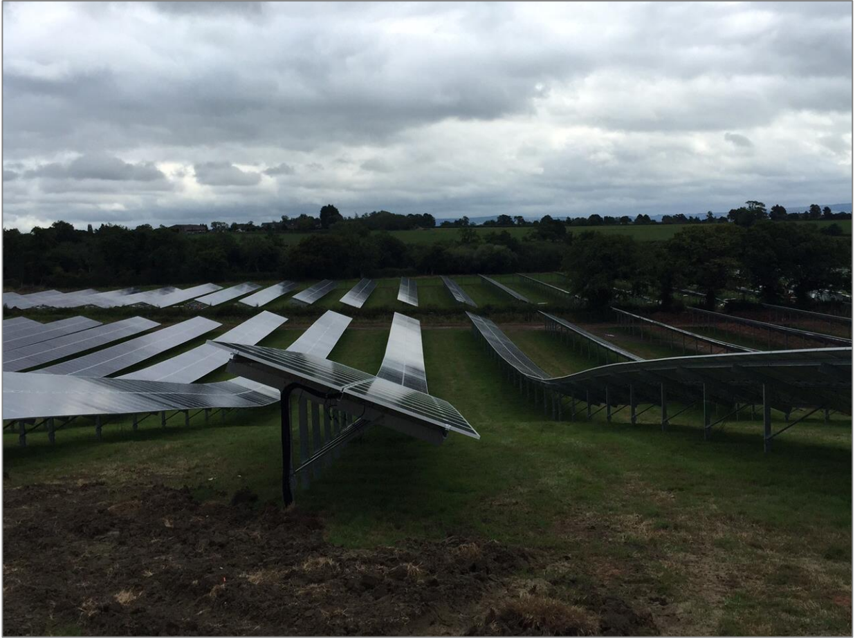
Figure 3: Fully assembled fixed array solar farm (image supplied by Infinergy UK).
