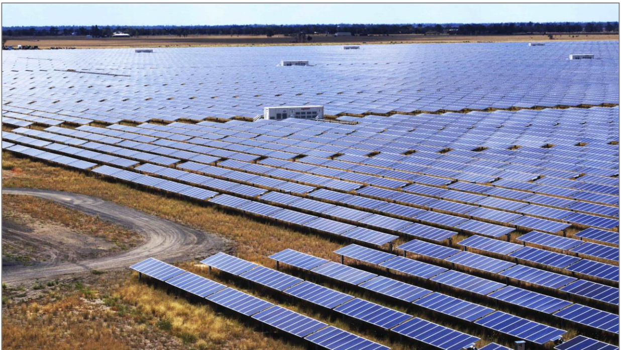
Figure 4: Fully assembled tracking array solar farm showing inverter housing (image courtesy Nextracker Australia, actual system may differ).
