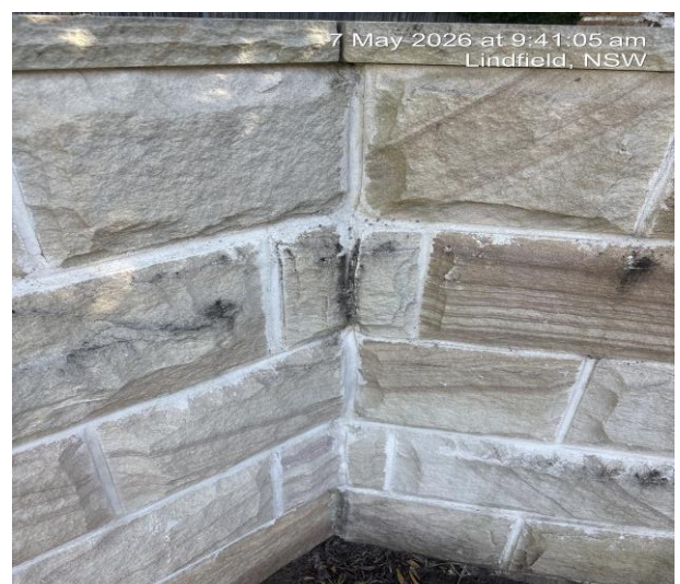
Photo 96 – Cracking observed to mortar
