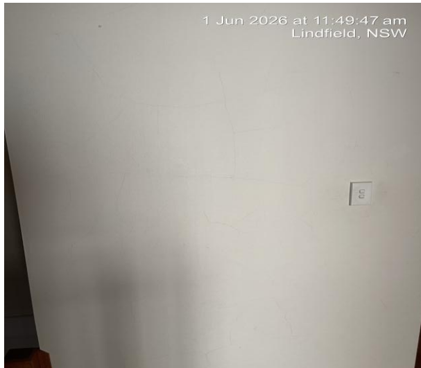
Photo 79 – Cracking observed to render
