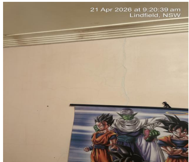
Photo 82 – Cracking observed to wall
