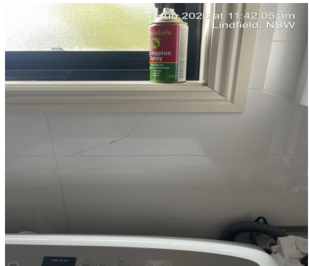
Photo 28 - Cracking observed to tiles
