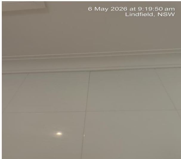
Photo 67 - Movement observed to coving
