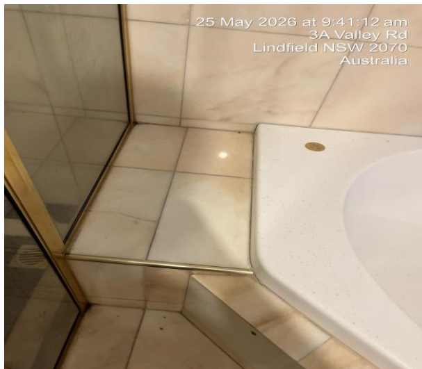
Photo 117 – Cracking observed to tiles
