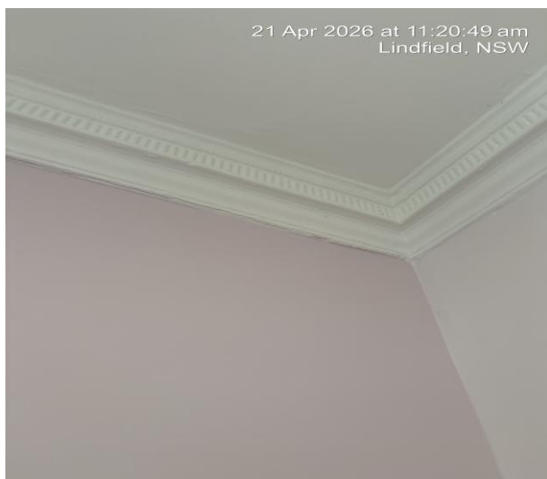
Photo 47 – Cracking observed to coving
