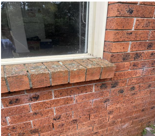
Photo 201 – Damage observed to mortar
