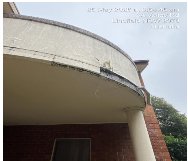
Photo 166 – Water ingress and damage observed to upturn
