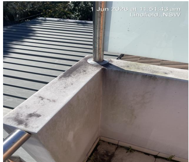
Photo 92 – Mould growth observed
