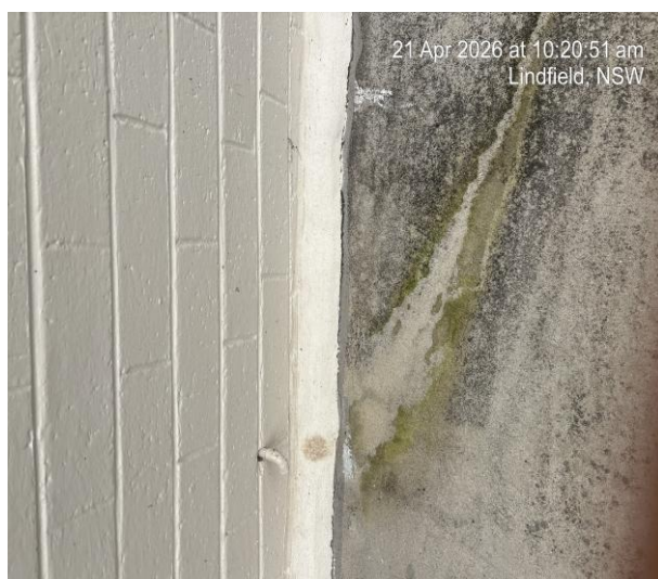
Photo 77 – Cracking observed to wall/floor junction
