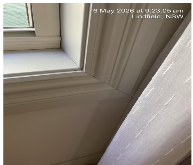
Photo 84 – Cracking observed to window frame
