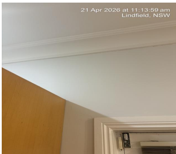
Photo 23 - Cracking observed to wall
