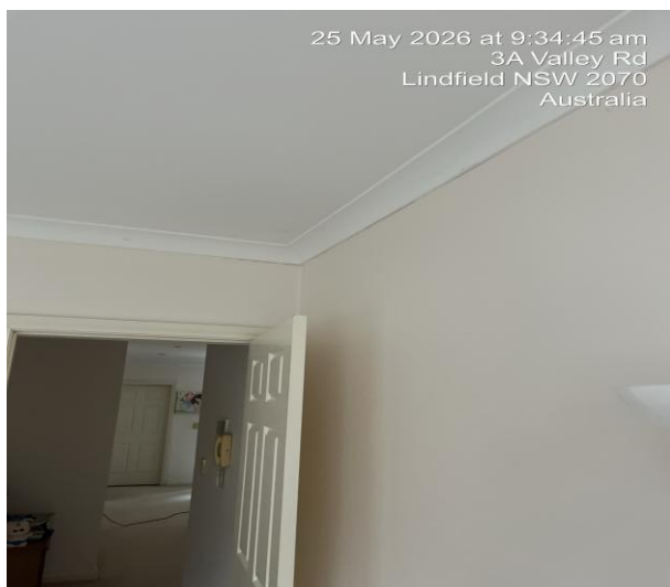
Photo 89 - Cracking observed to coving
