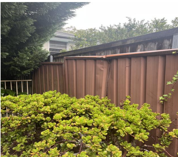
Photo 191 – Damage observed to fence
