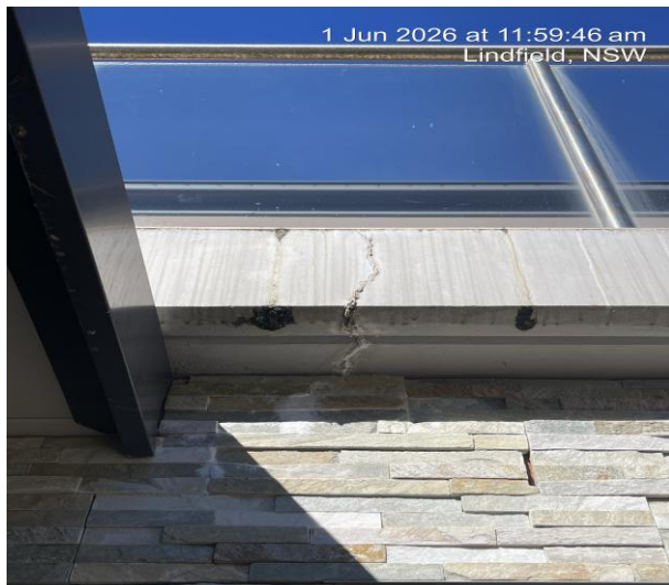
Photo 141 – Cracking and efflorescence observed to edge of balcony
