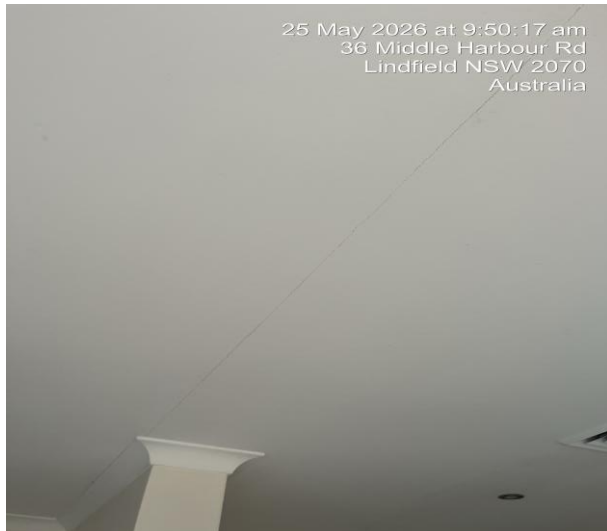
Photo 13 – Cracking observed to ceiling
