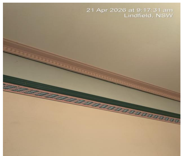
Photo 60 – Movement observed to coving
