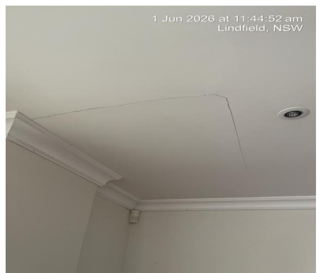
Photo 48 - Cracking observed to ceiling
