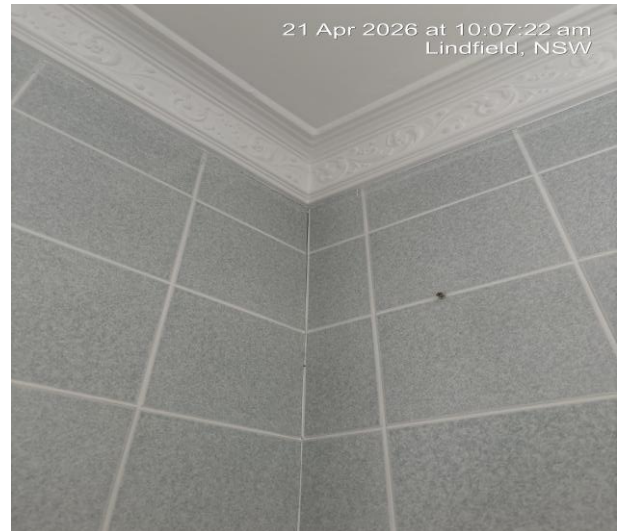
Photo 38 – Cracking observed to grout
