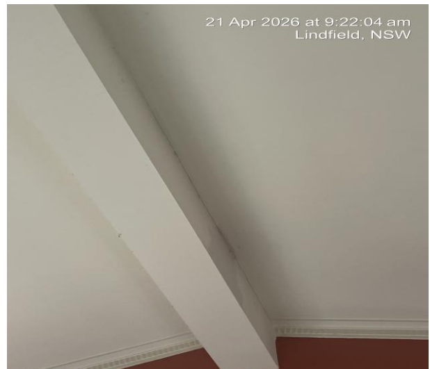
Photo 88 - Cracking observed to ceiling junction
