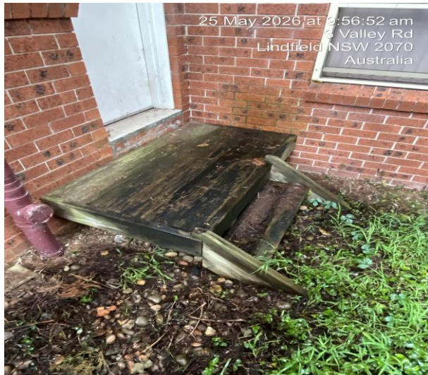
Photo 181 – Weathering observed to stairs
