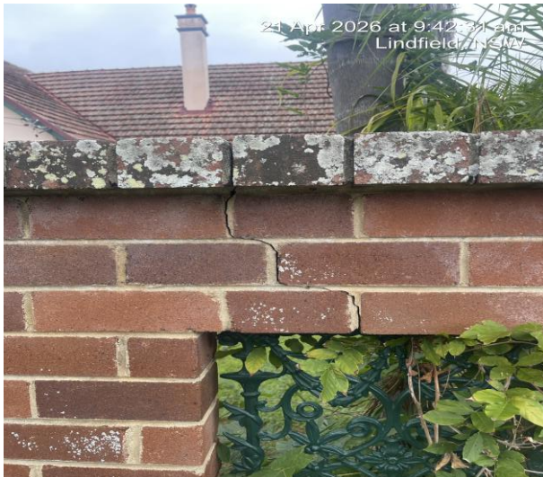
Photo 157 – Cracking observed to brick fence
