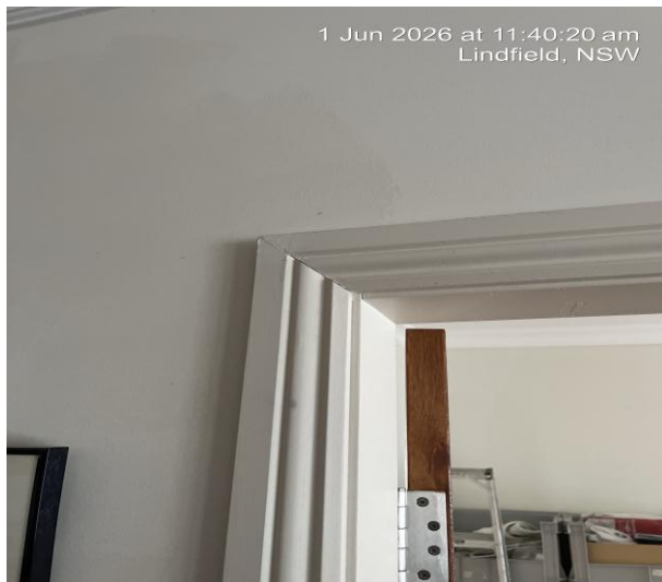
Photo 15 – Cracking observed to door frame
