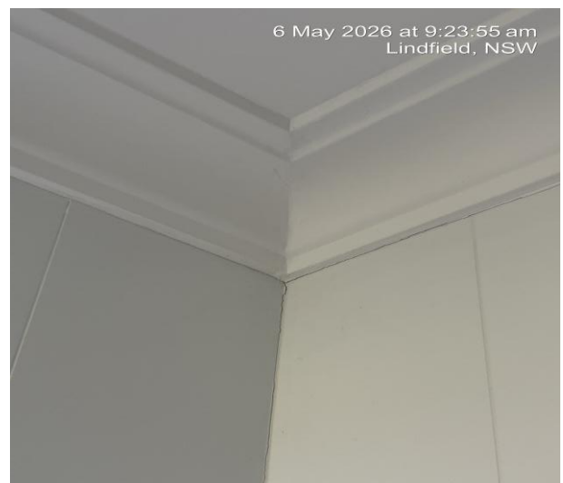
Photo 90 – Cracking observed to grout and coving
