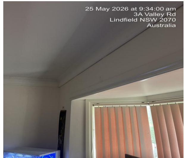
Photo 86 - Movement observed to coving
