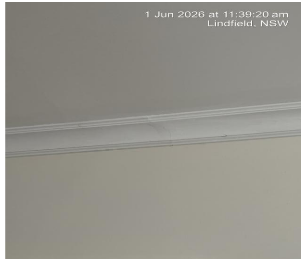
Photo 14 – Damaged observed to coving
