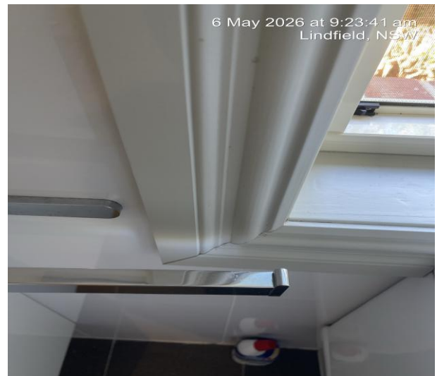
Photo 88 – Cracking observed to window frame
