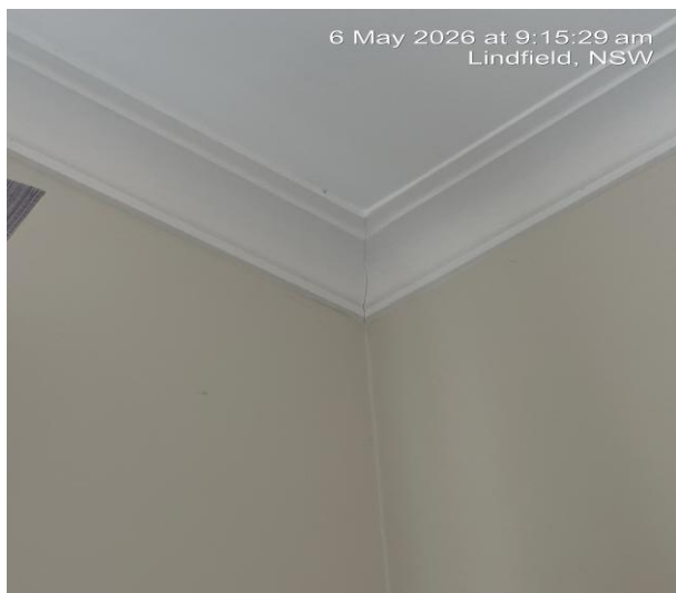
Photo 45 – Cracking observed to coving
