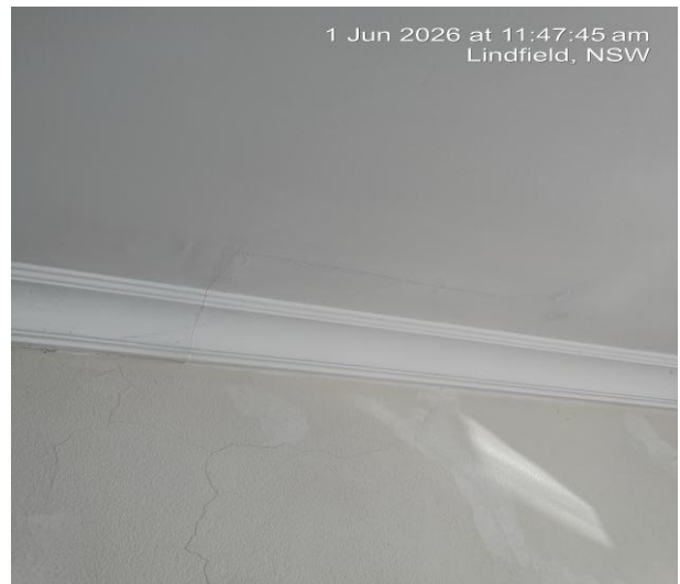
Photo 70 – Cracking observed to ceiling and render
