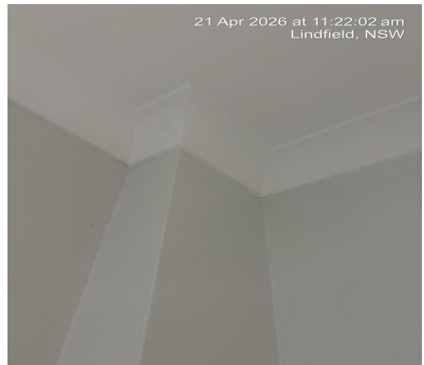
Photo 52 – Cracking observed to coving
