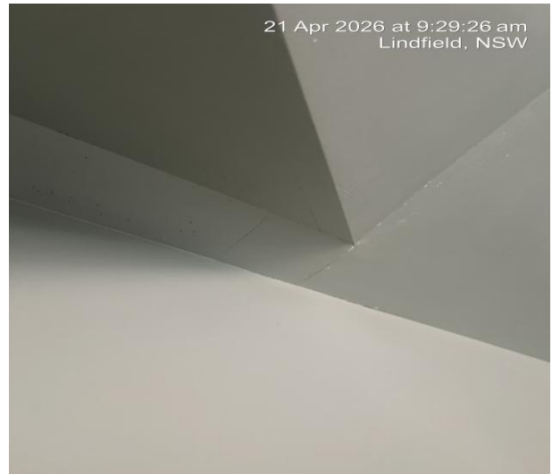
Photo 116 – Cracking observed to ceiling
