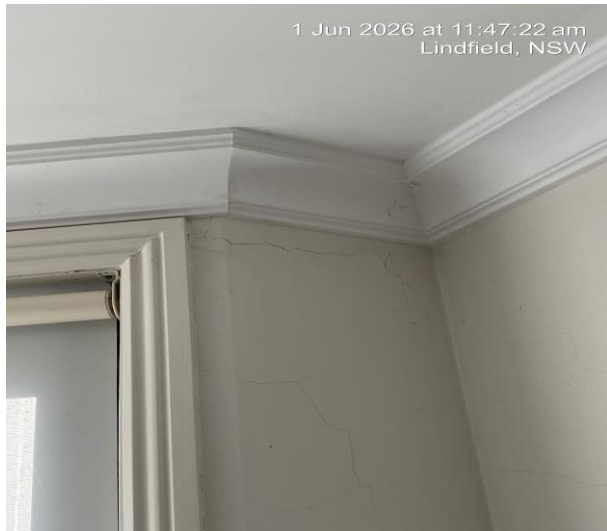
Photo 67 – Cracking observed to render
