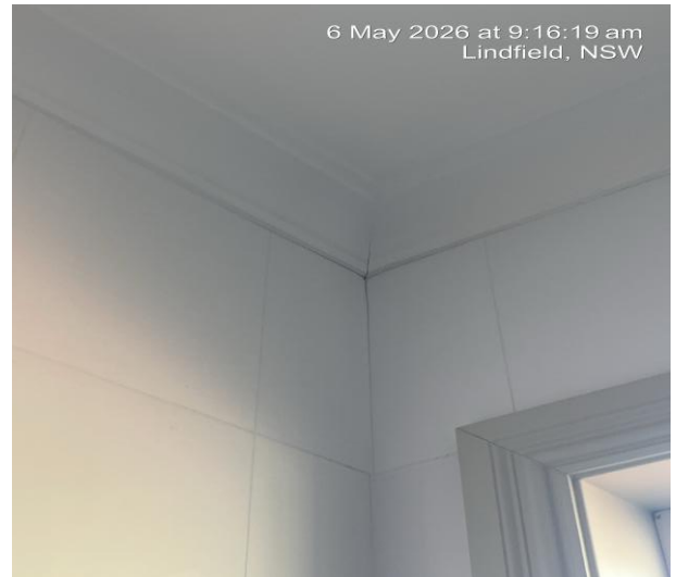
Photo 50 – Cracking observed to grout and coving
