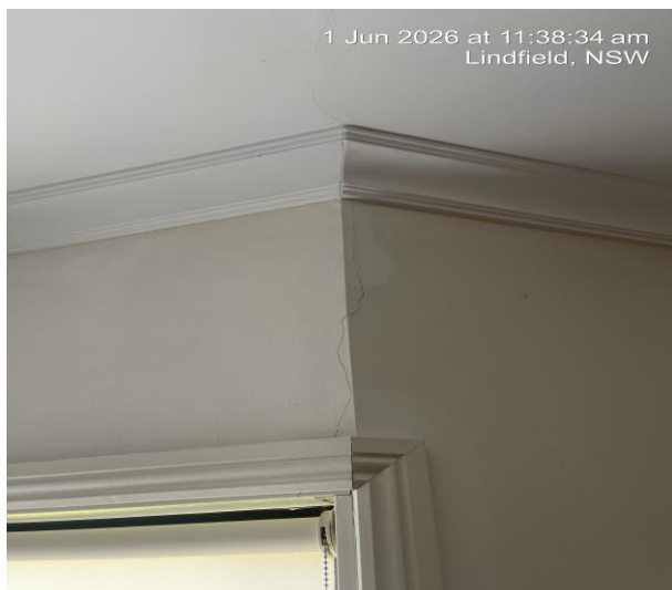
Photo 9 – Cracking observed to render
