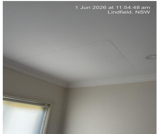
Photo 116 – Cracking observed to ceiling
