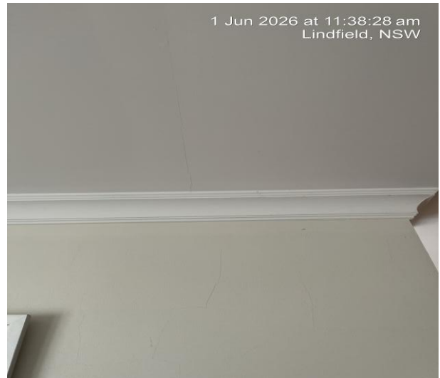
Photo 8 – Cracking observed to render and ceiling
