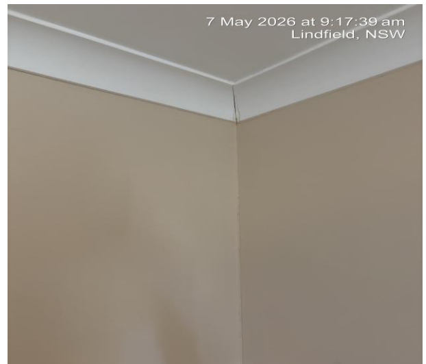
Photo 64 - Cracking observed to coving
