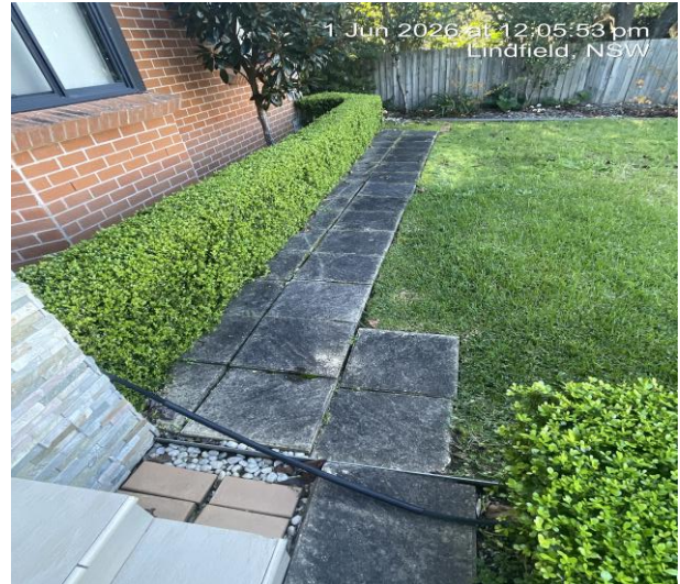
Photo 170 – Settlement observed to pavers
