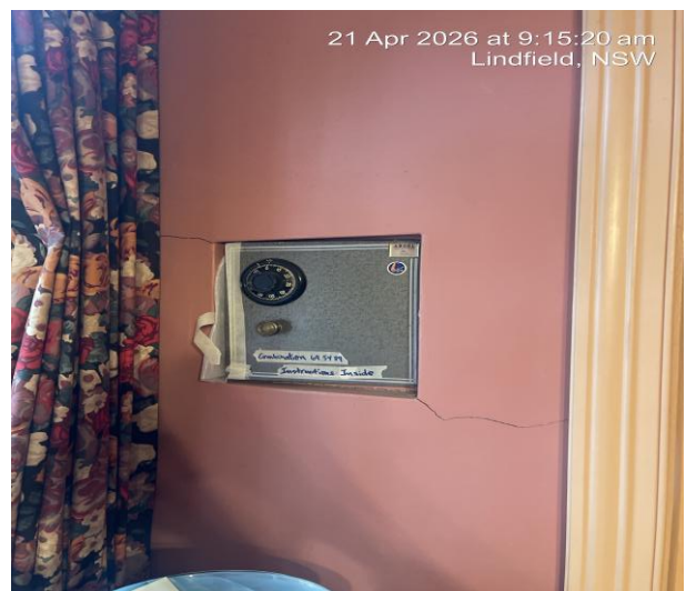
Photo 48 - Cracking observed to wall
