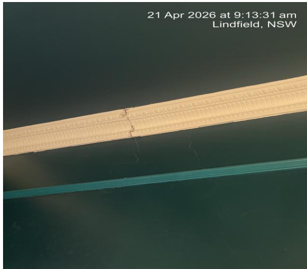
Photo 37 – Cracking observed to wall and coving
