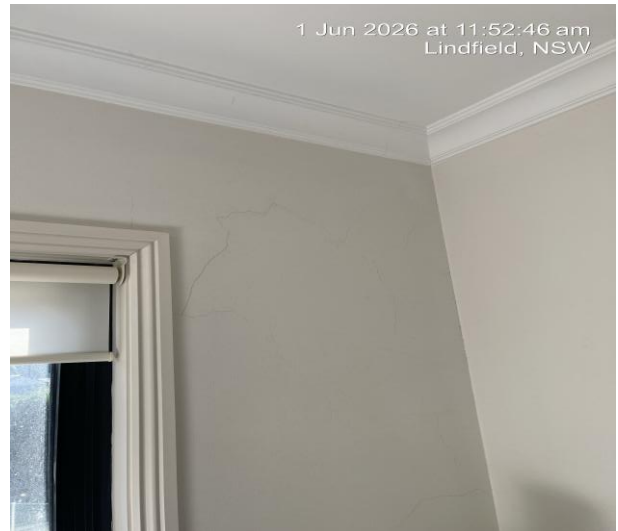
Photo 98 – Cracking observed to render
