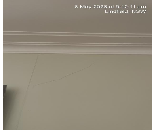
Photo 32 – 45° crack observed to gyprock
