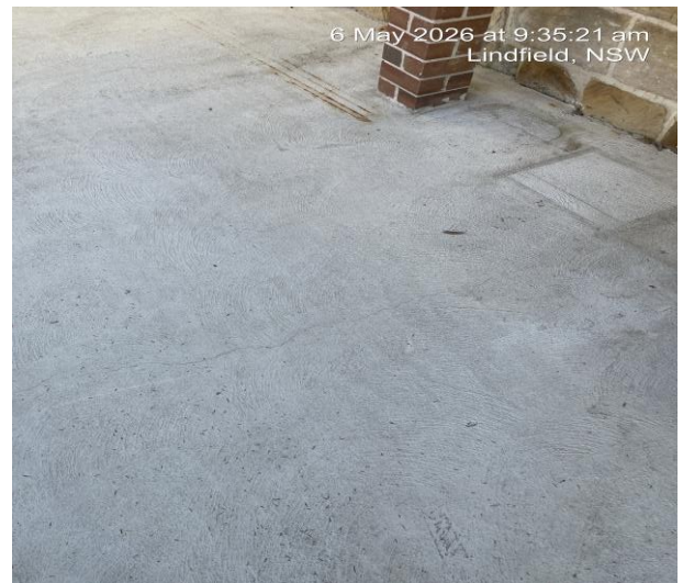
Photo 136 – Cracking observed to concrete
