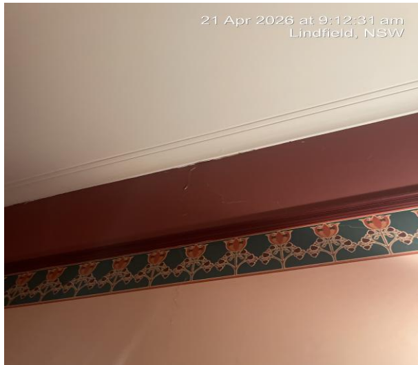
Photo 31 – Cracking observed to wall
