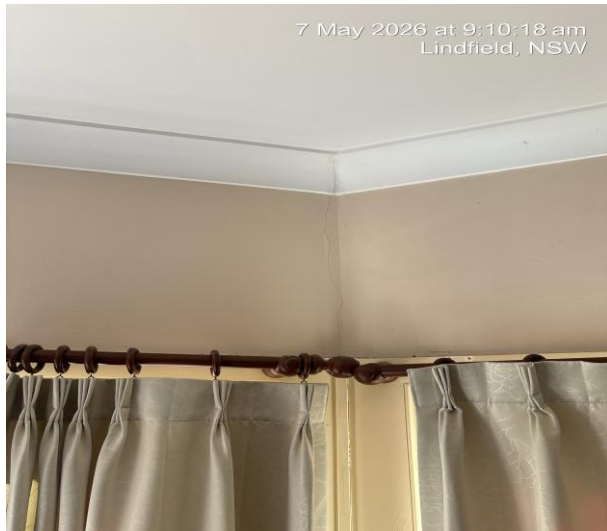
Photo 31 – Cracking observed to wall and coving
