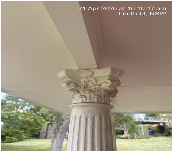
Photo 43 – Movement observed to top of column
