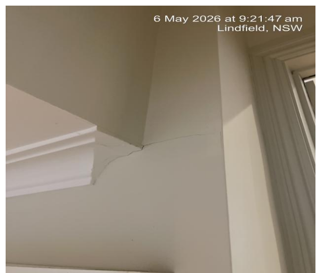
Photo 78 – Cracking observed to gyprock wall
