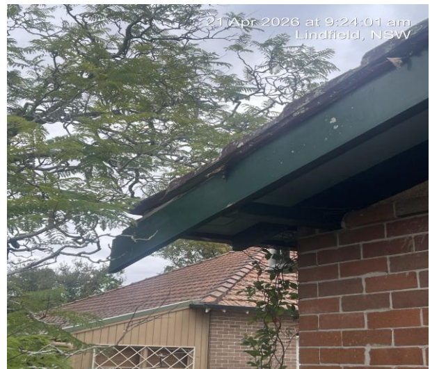
Photo 94 – Weathering observed to fascia
