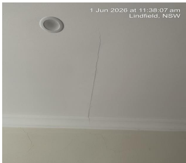
Photo 3 – Cracking observed to render and ceiling
