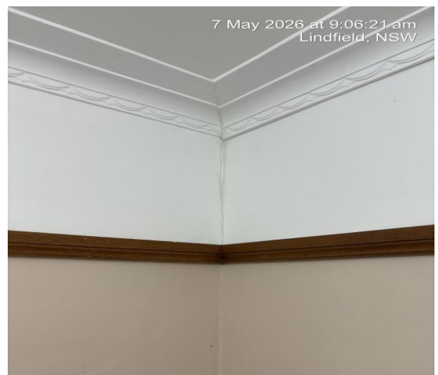
Photo 12 – Cracking and water damage observed to wall and coving
