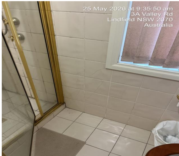
Photo 97 – Cracking observed to tiles
