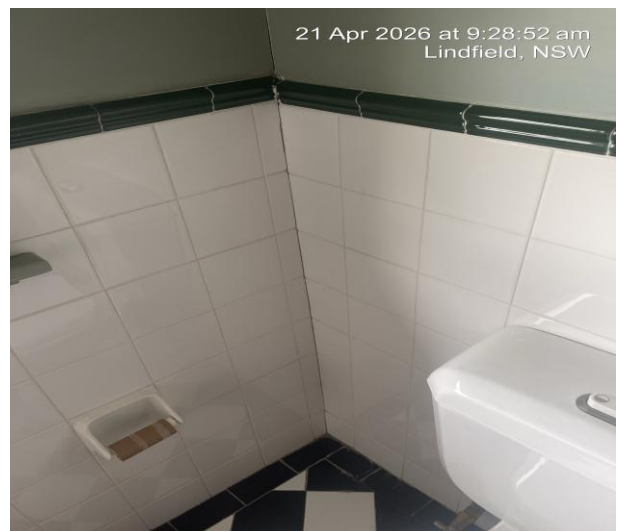
Photo 114 - Vertical crack observed to wall junction
