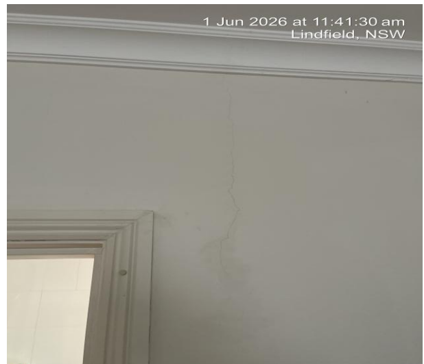
Photo 22 - Cracking observed to render
