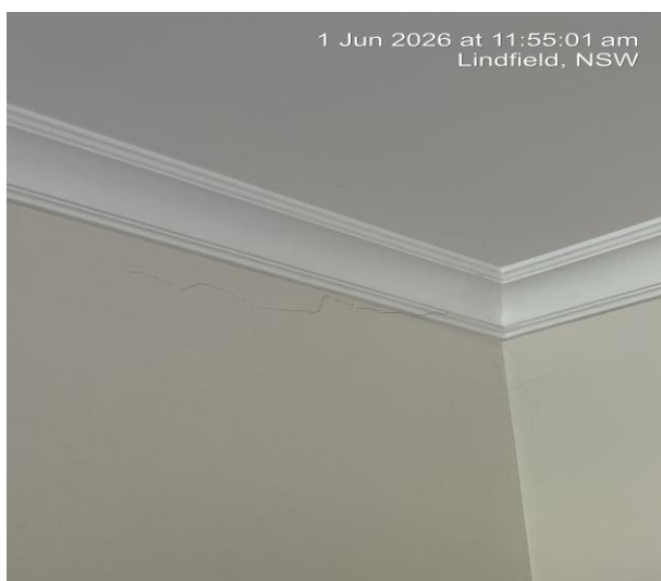
Photo 119 – Cracking observed to render
