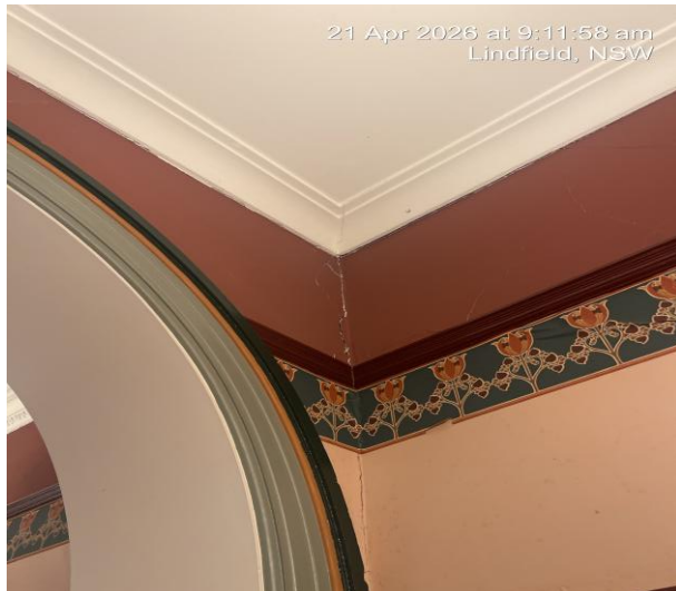
Photo 25 – Vertical cracking observed to wall
