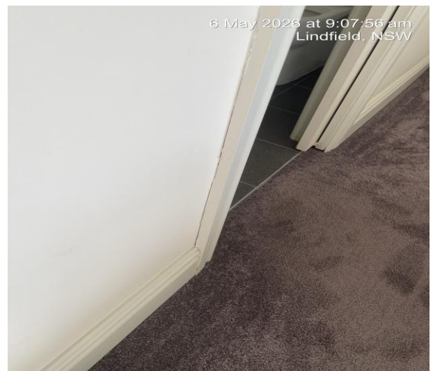
Photo 10 - Cracking observed to doorframe
