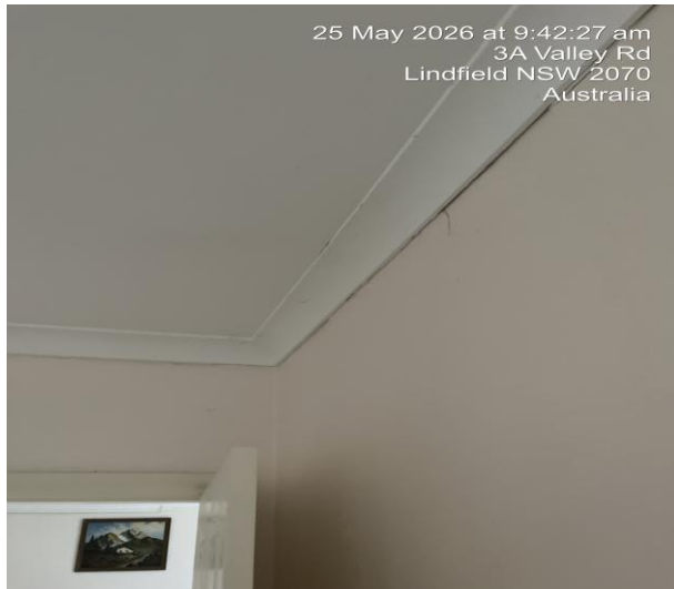
Photo 121 – Cracking observed to coving
