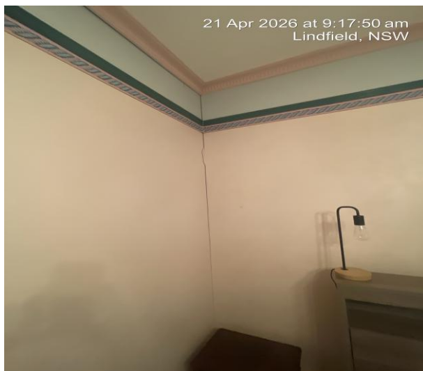
Photo 63 – Vertical crack observed at wall junction
