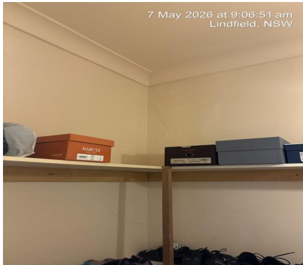
Photo 13 – Cracking observed to wall
