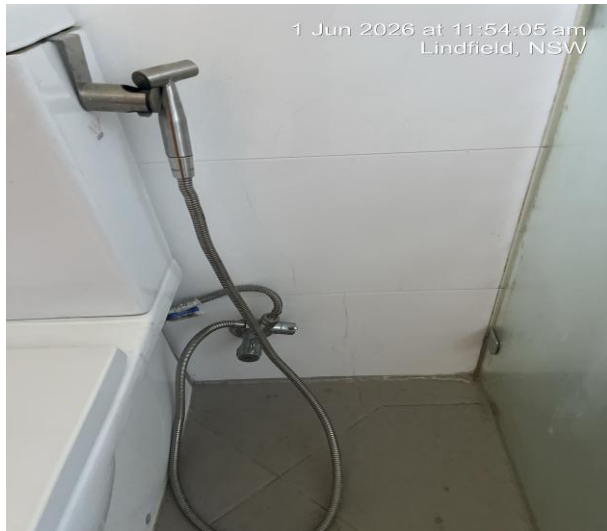
Photo 109 – Cracking observed to tiles
