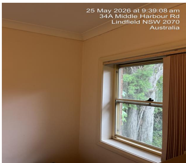
Photo 107 – Cracking observed to coving
