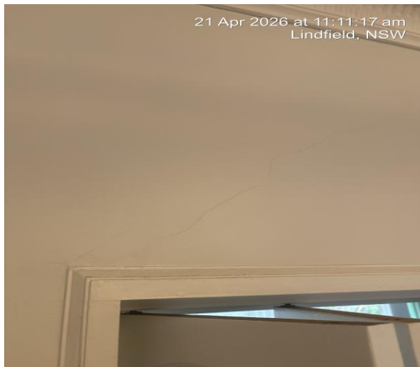
Photo 15 - 45° crack observed to wall
