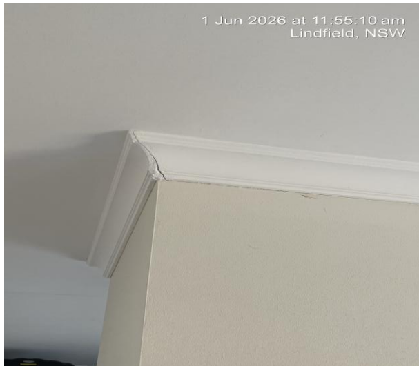
Photo 121 – Cracking observed to coving
