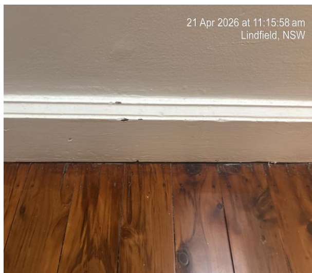
Photo 29 – Movement observed to floorboards
