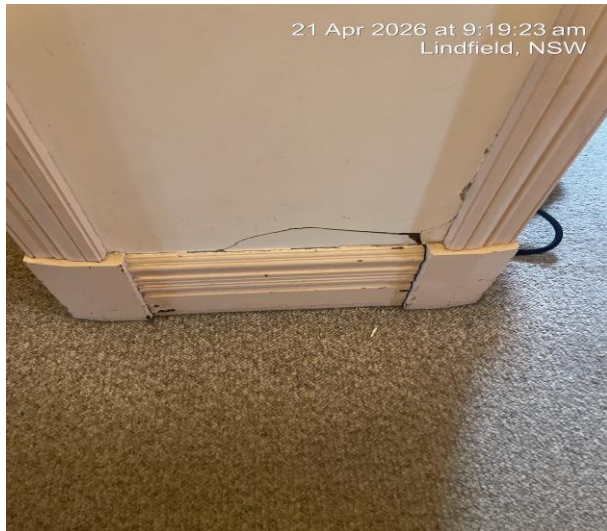
Photo 73 – Cracking observed to wall and skirting
