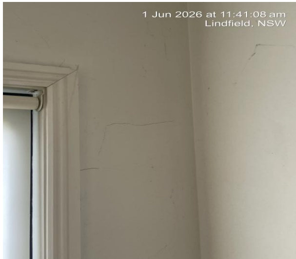
Photo 19 – Cracking observed to render
