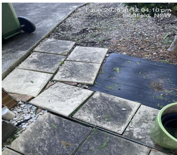
Photo 161 - Settlement observed to pavers
