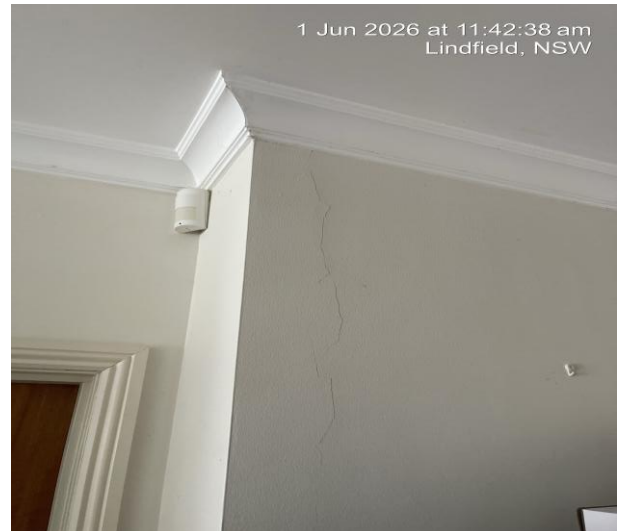
Photo 32 – Cracking observed to render
