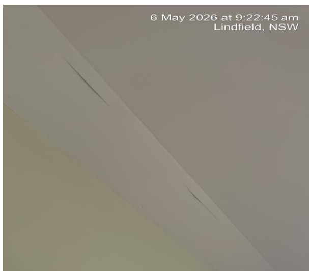
Photo 83 – Delamination observed to gyprock ceiling junction
