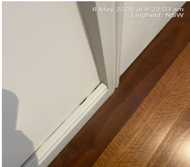
Photo 79 – Movement observed to skirting
