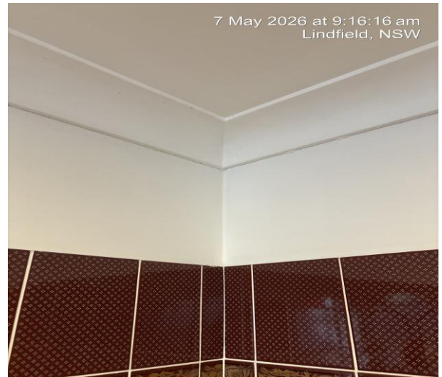
Photo 56 - Cracking observed to wall-coving join
