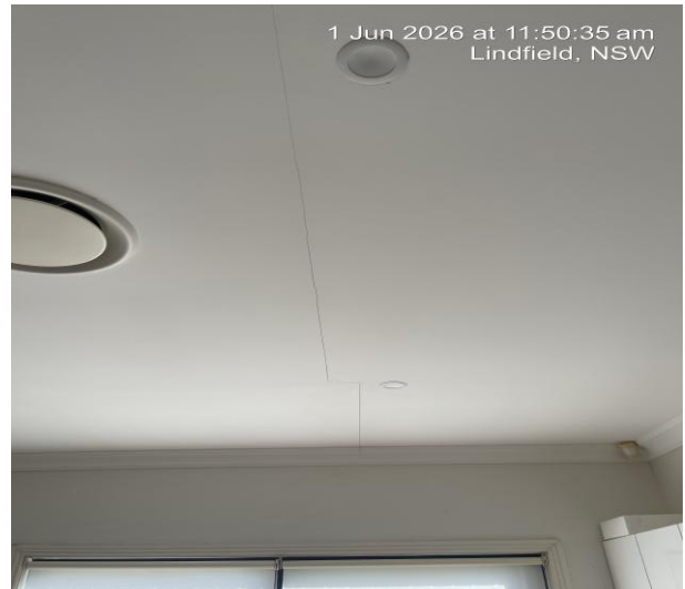
Photo 86 - Cracking observed to ceiling
