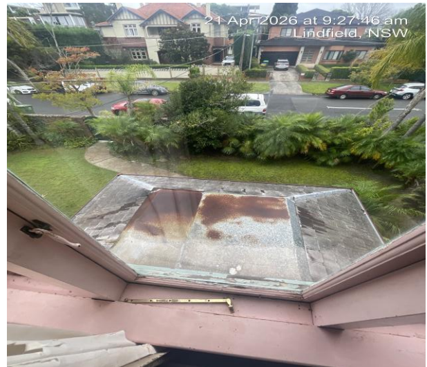
Photo 110 – Rust and age-related wear observed to front porch roof
