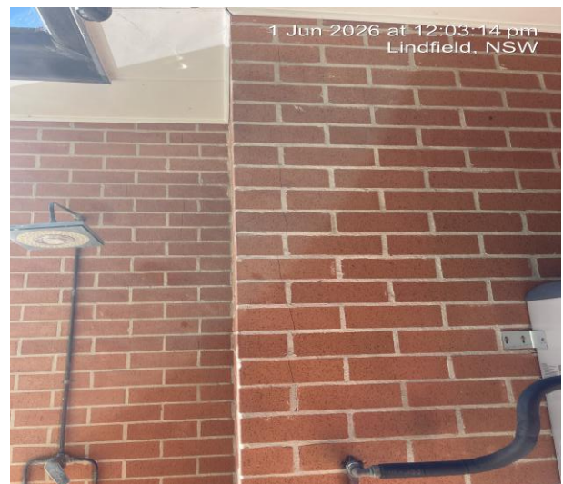
Photo 156 – Cracking observed to brick facade
