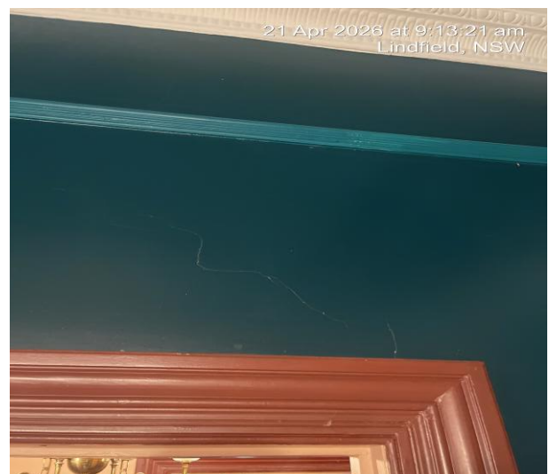
Photo 36 - Cracking observed to wall
