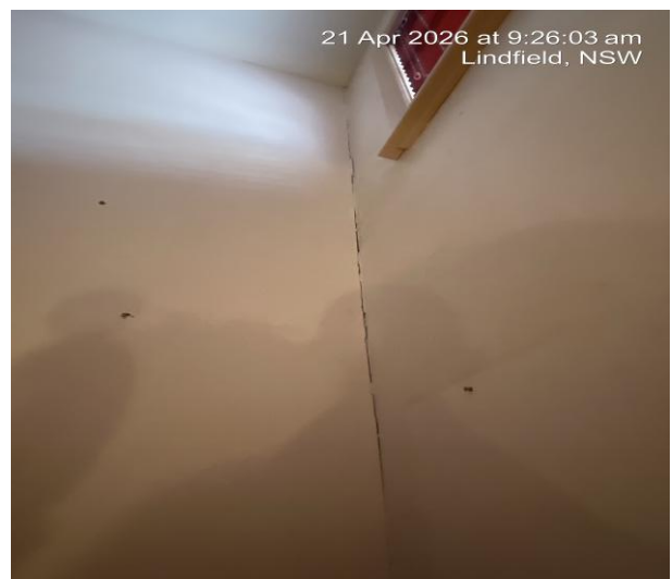
Photo 102 – Vertical crack observed to wall junction
