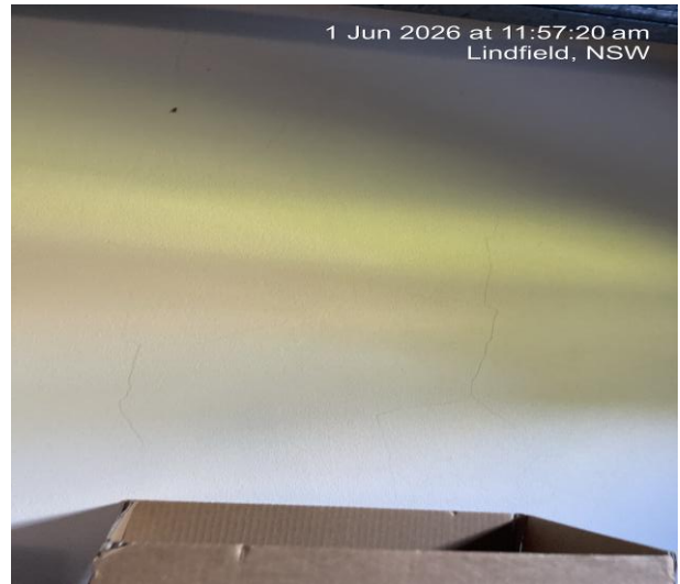
Photo 134 – Cracking observed to render
