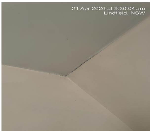
Photo 119 – Cracking observed to ceiling junction
