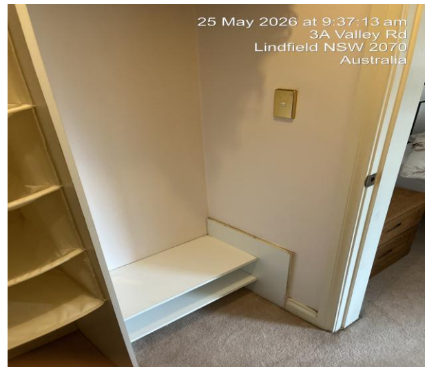
Photo 100 – Cracking observed to paint
