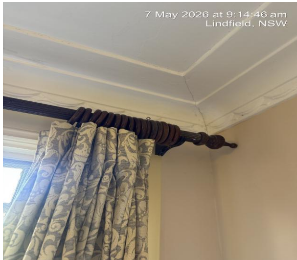
Photo 49 - Cracking observed to coving
