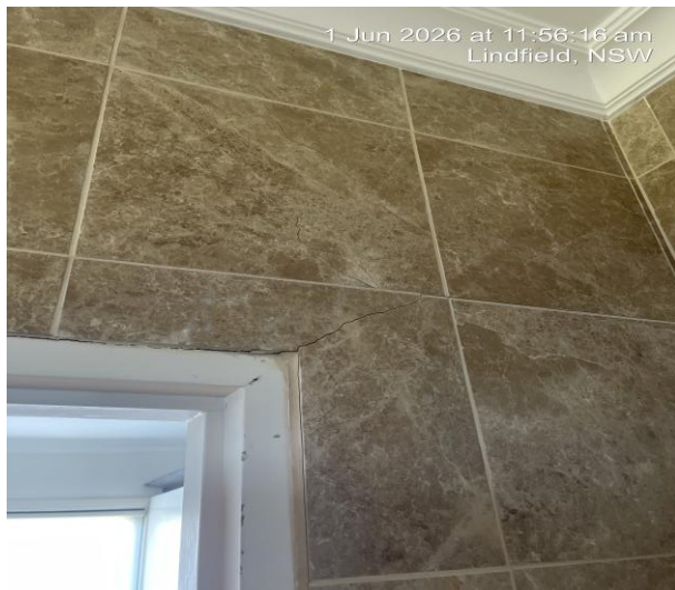
Photo 129 - Cracking observed to tiles
