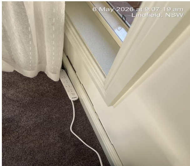
Photo 7 – Movement observed to skirting
