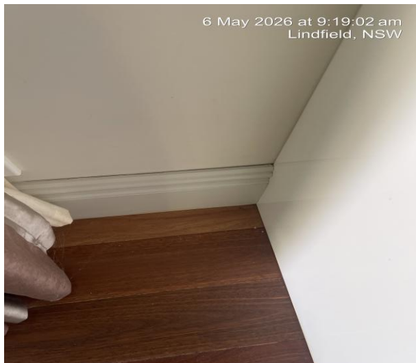
Photo 63 – Movement observed to skirting
