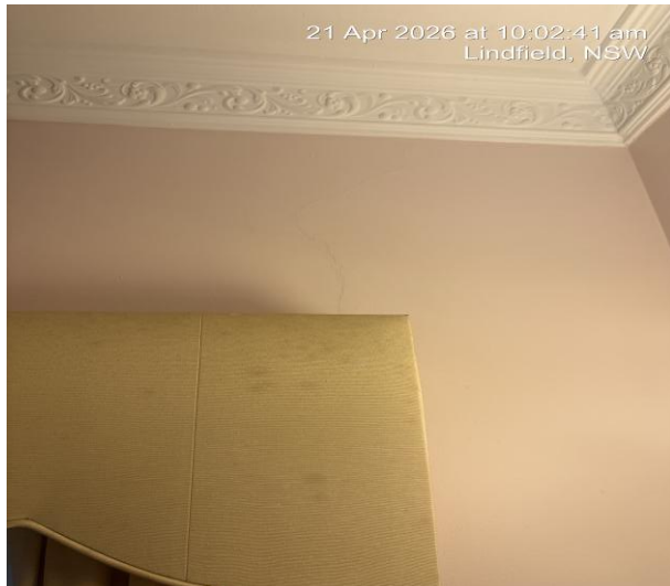
Photo 13 – Cracking observed to wall
