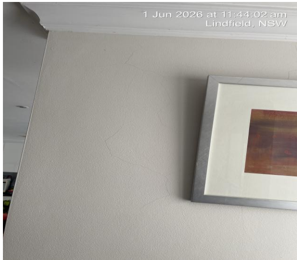
Photo 43 – Cracking observed to render
