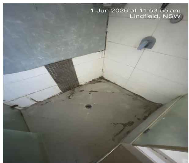
Photo 108 – Mould growth observed to shower area
