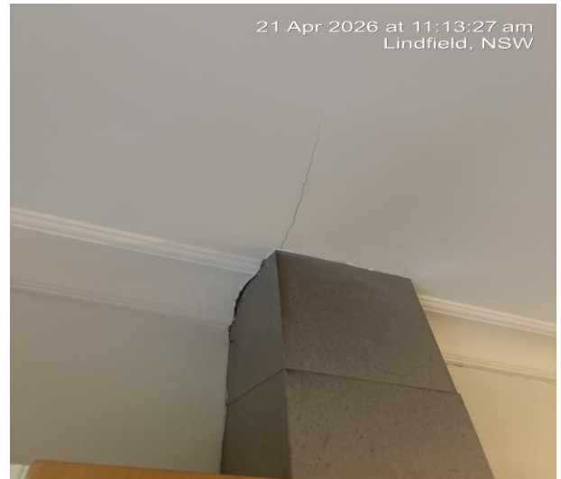
Photo 20 - Cracking observed to ceiling
