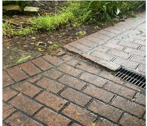
Photo 218 – Settlement observed to driveway pavers
