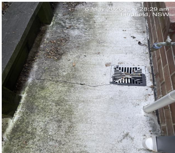
Photo 105 – Cracking observed to concrete
