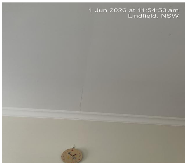
Photo 117 - Cracking observed to ceiling
