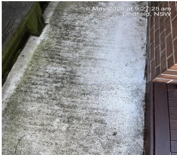
Photo 103 – Cracking observed to concrete
