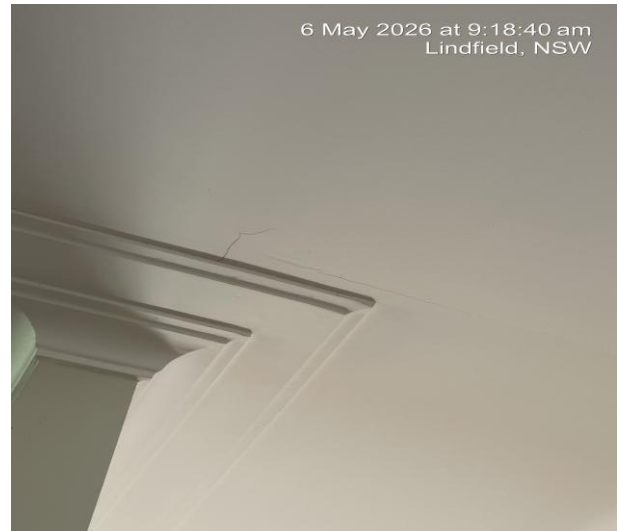
Photo 62 – Cracking observed to ceiling
