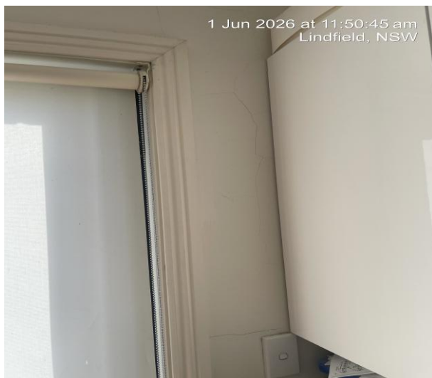
Photo 87 - Cracking observed to render
