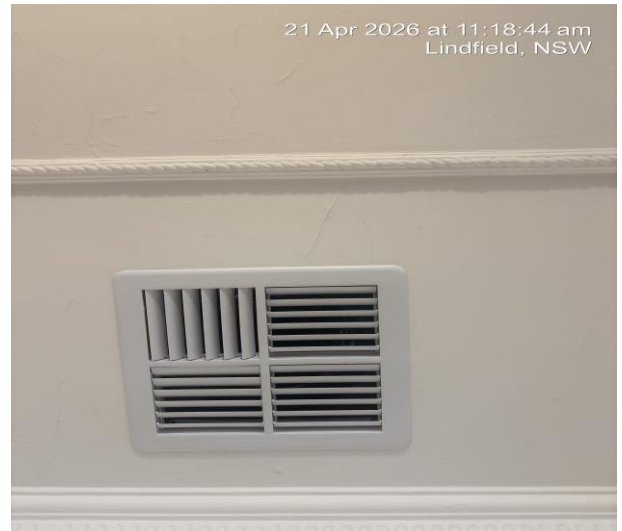
Photo 38 – Cracking observed to ceiling
