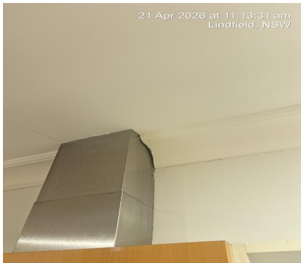
Photo 21 – Cracking observed to wall/coving junction
