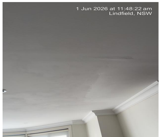
Photo 72 – Damage observed to ceiling consistent with water ingress
