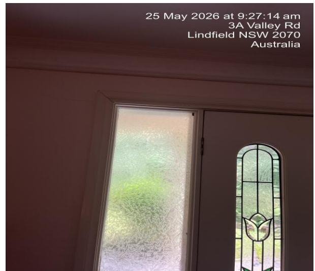
Photo 52 – Cracking observed to wall and frame
