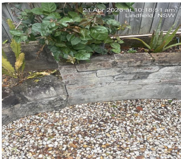
Photo 69 – Cracking observed to mortar
