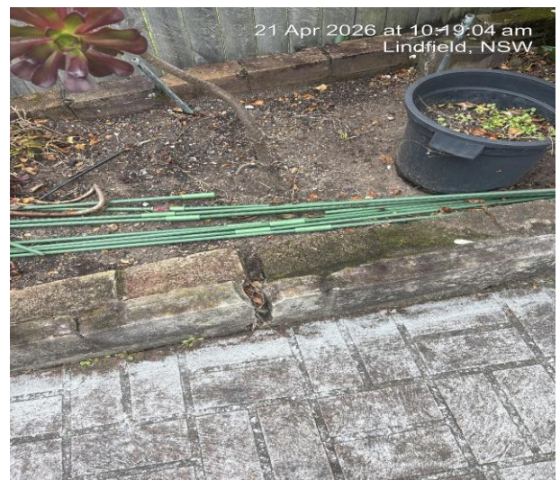
Photo 70 – Cracking observed to stone
