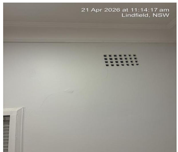
Photo 24 – 45° crack observed to wall
