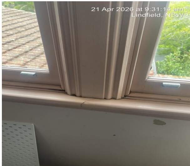
Photo 121 – Cracking observed to window frame
