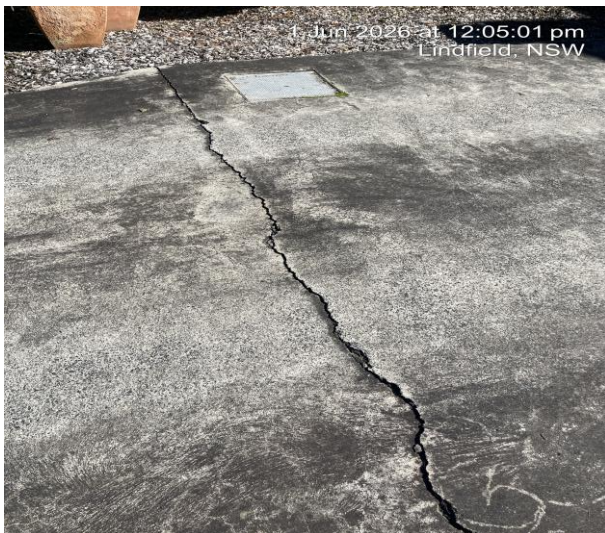
Photo 165 – Cracking observed to concrete
