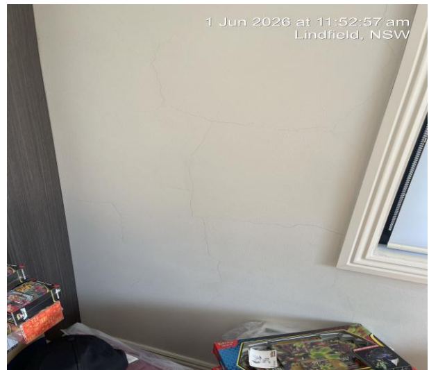
Photo 100 - Cracking observed to render
