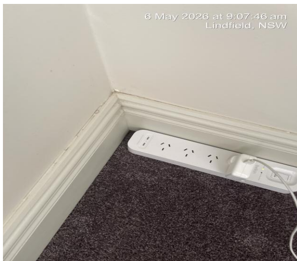
Photo 9 - Cracking observed to skirting
