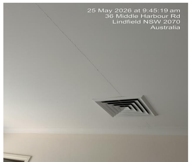
Photo 138 – Cracking observed to ceiling
