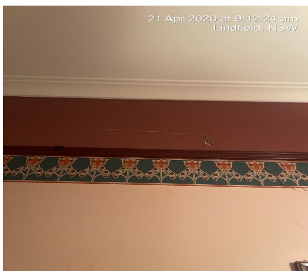
Photo 29 - Cracking observed to wall
