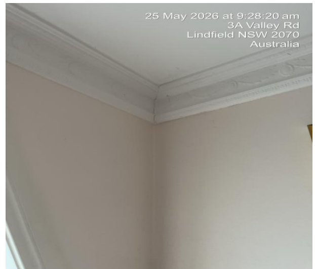
Photo 58 – Cracking observed to coving
