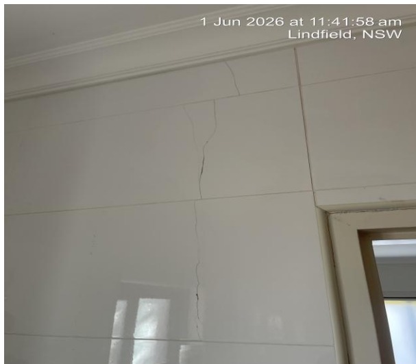
Photo 27 – Cracking observed to tiles
