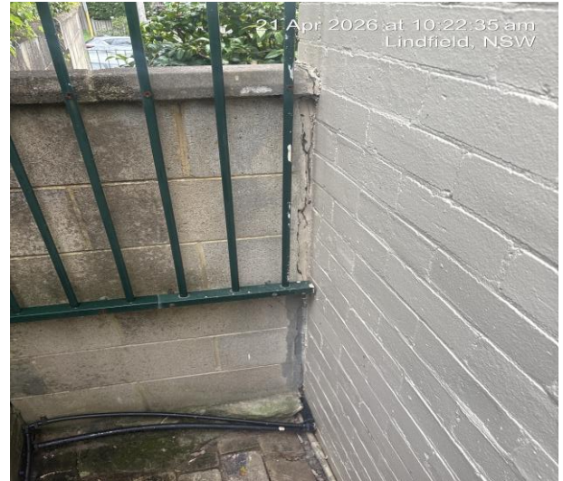
Photo 80 – Cracking observed to mortar
