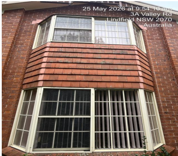
Photo 163 – Mold growth observed to tiling
