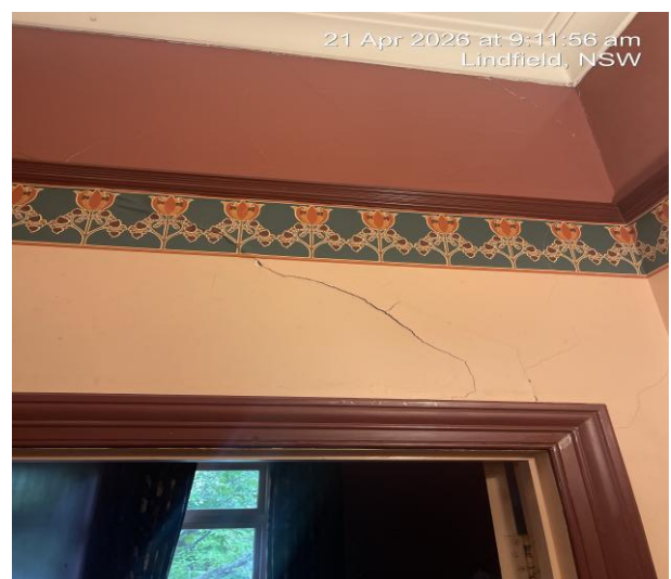
Photo 24 – 45° crack observed to wall
