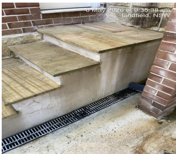
Photo 137 – Cracking observed to render
