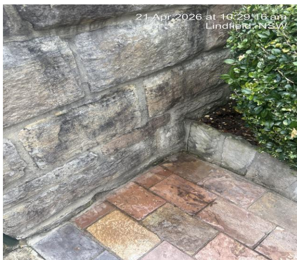
Photo 95 – Cracking observed to mortar
