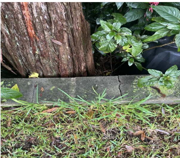
Photo 209 – Cracking observed to capping block
