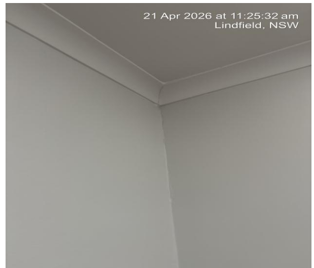
Photo 64 - Cracking observed to wall and coving
