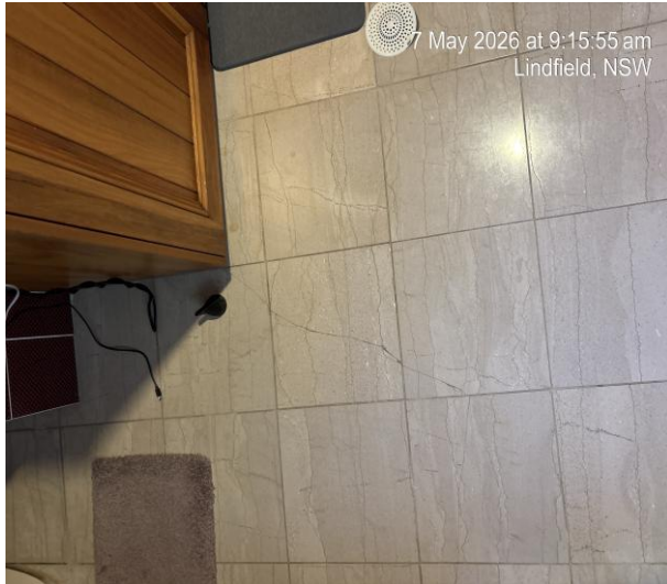
Photo 55 - Cracking observed to tiling
