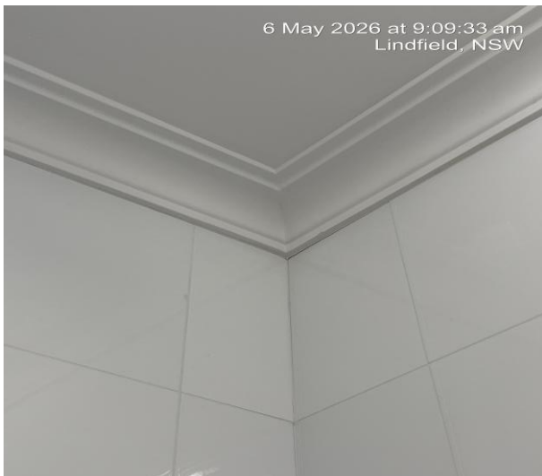
Photo 21 – Cracking observed to grout and coving
