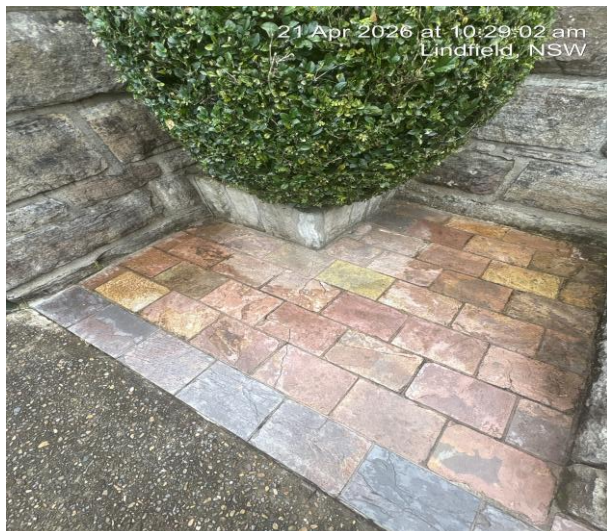
Photo 93 – Cracking observed to tiles
