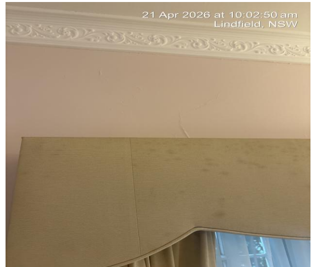
Photo 14 - Cracking observed to wall
