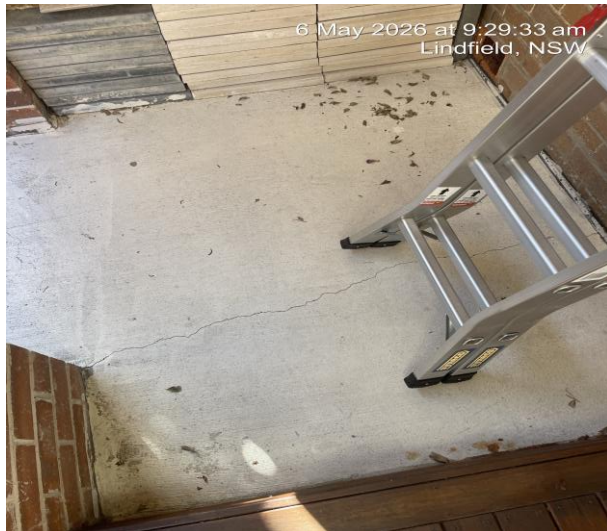
Photo 109 – Cracking observed to concrete
