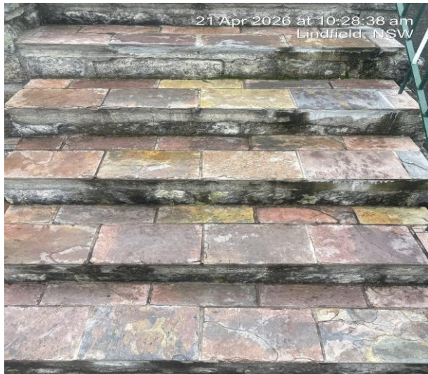
Photo 91 – Cracking observed to tiles
