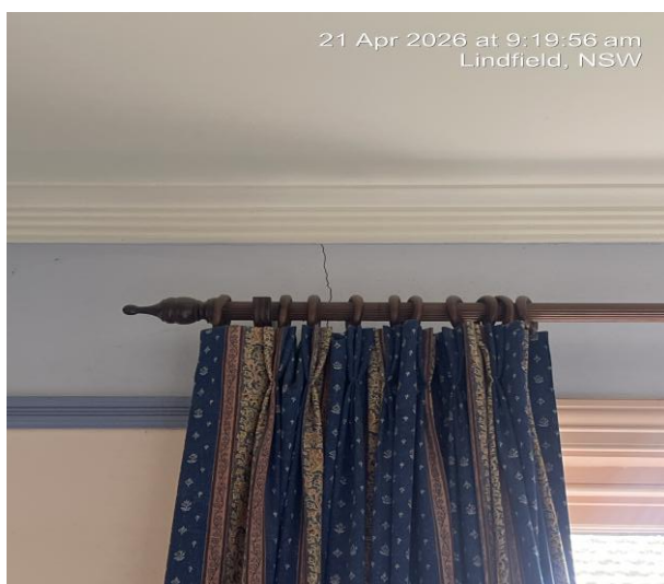
Photo 77 – Vertical crack observed to wall
