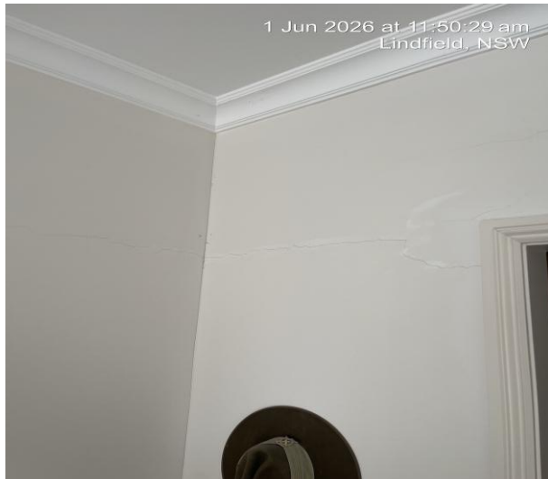
Photo 85 - Cracking observed to render with signs of attempts to repair
