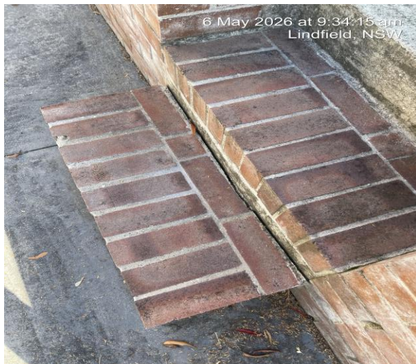
Photo 129 – Movement observed to stairs
