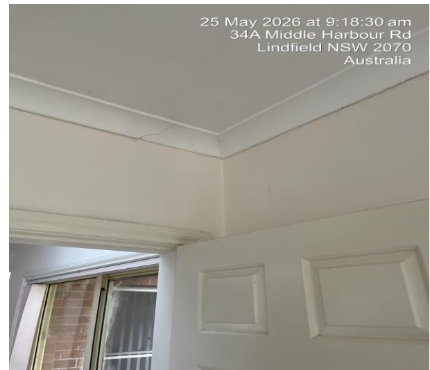
Photo 2 – Cracking observed to coving
