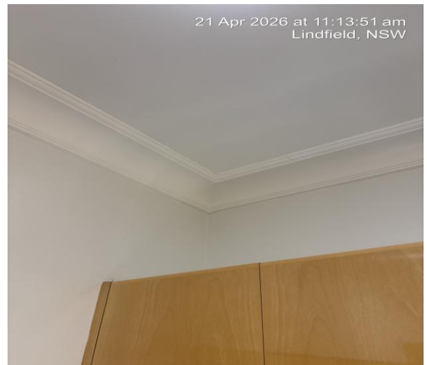
Photo 22 - Cracking observed to coving
