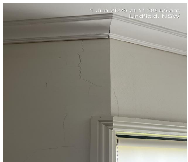
Photo 12 – Cracking observed to render
