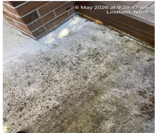
Photo 110 - Cracking observed to concrete
