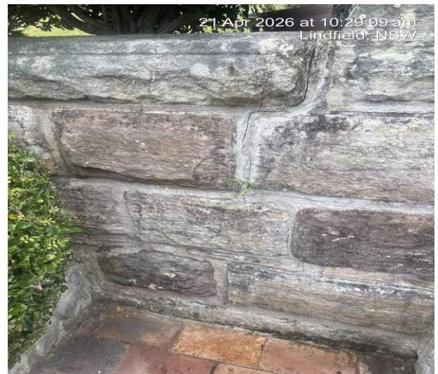
Photo 94 – Cracking observed to mortar
