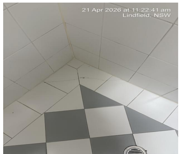
Photo 54 – Cracking observed to tiles
