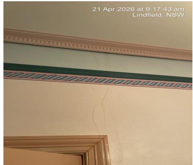
Photo 62 - Cracking observed to wall
