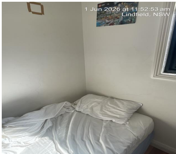
Photo 99 - Cracking observed to render
