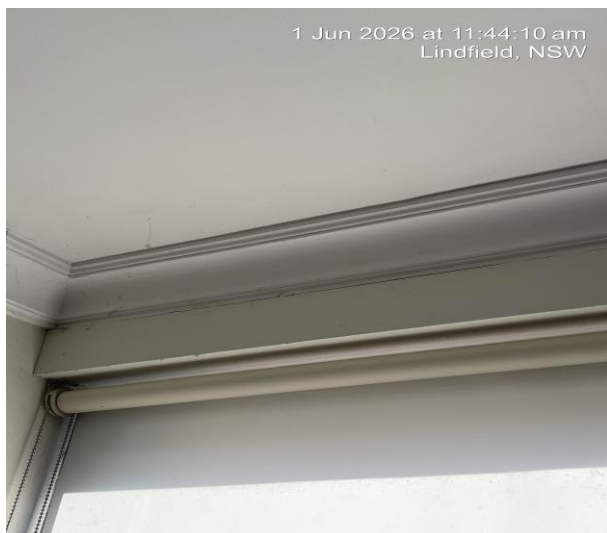
Photo 45 – Movement observed to coving
