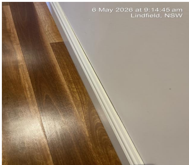
Photo 39 – Movement observed to skirting
