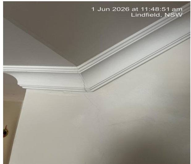
Photo 74 – Cracking observed to render and coving
