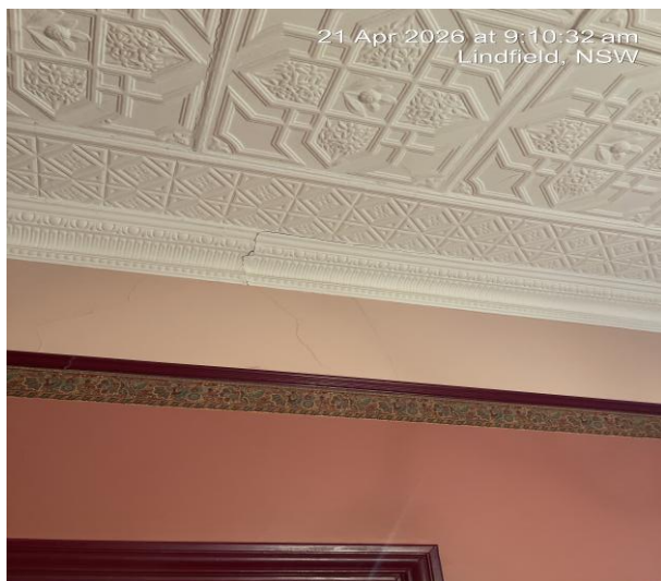
Photo 15 - Cracking observed to wall and coving
