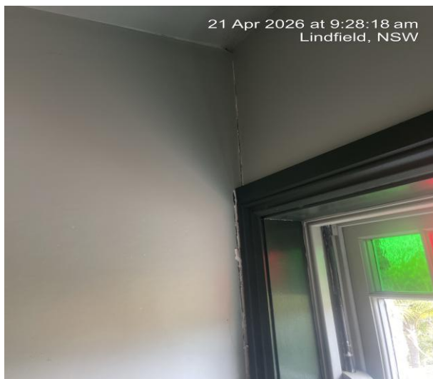
Photo 113 – Vertical crack observed to wall junction
