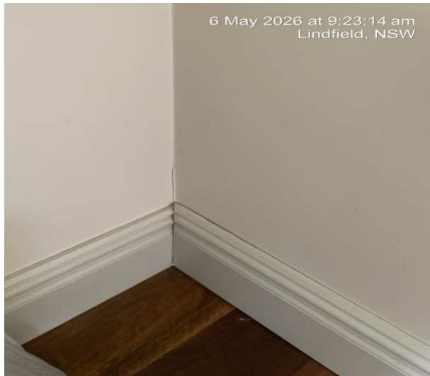
Photo 85 – Cracking observed to skirting and wall
