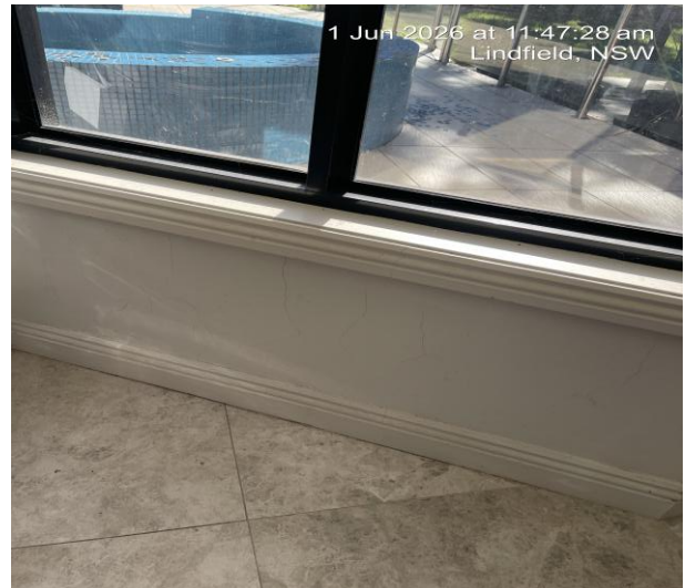
Photo 68 – Cracking observed to render
