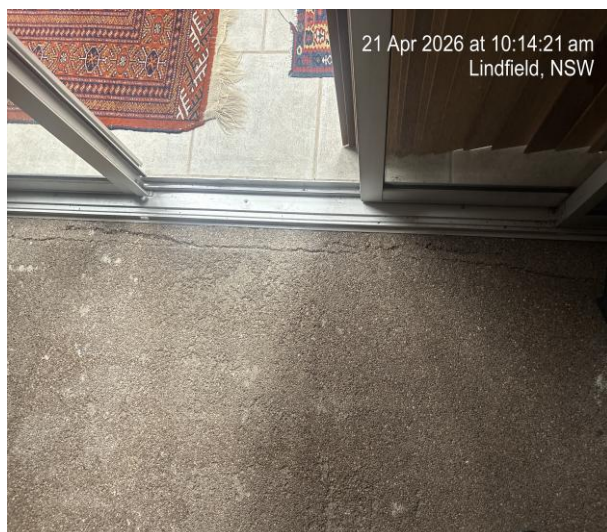
Photo 53 – Cracking observed to epoxy pebble flooring
