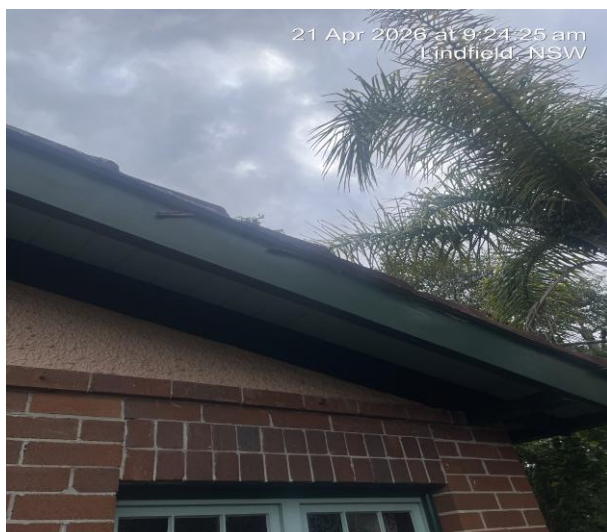
Photo 95 – Weathering observed to fascia
