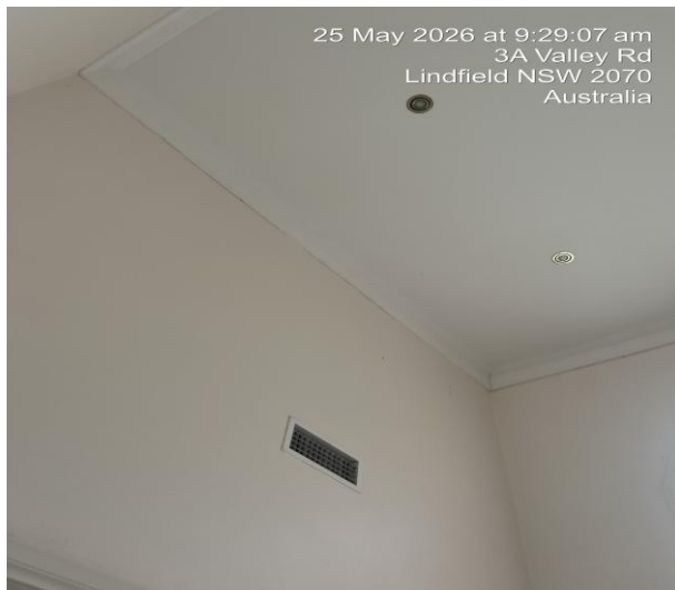
Photo 63 – Cracking observed to coving
