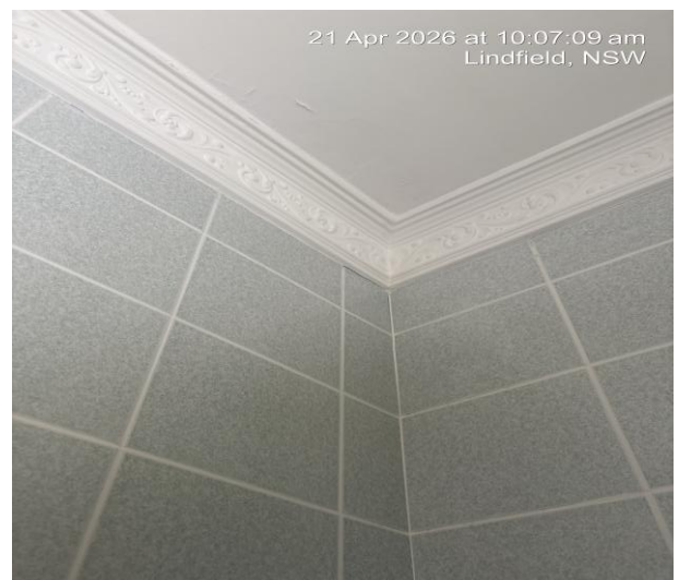
Photo 36 – Cracking observed to grout
