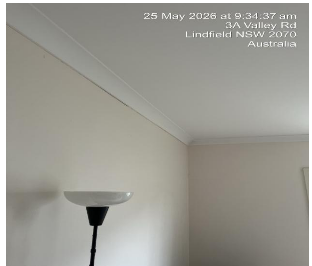
Photo 88 - Cracking observed to coving
