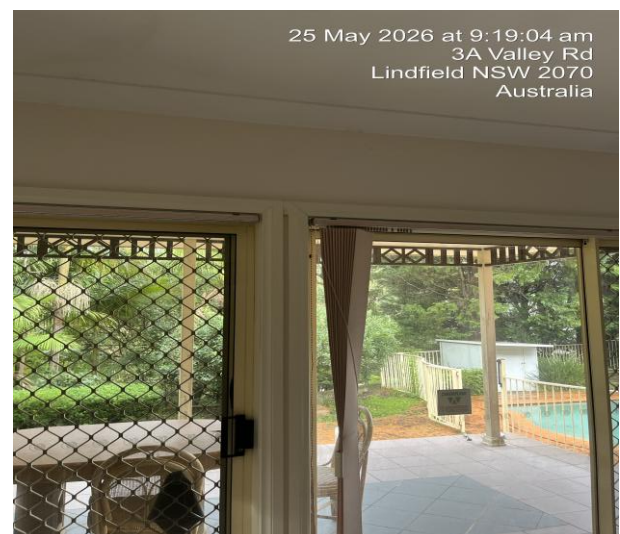
Photo 6 – Cracking observed to doorframe
