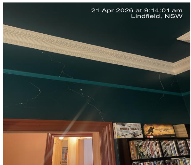
Photo 40 - Cracking observed to wall and coving
