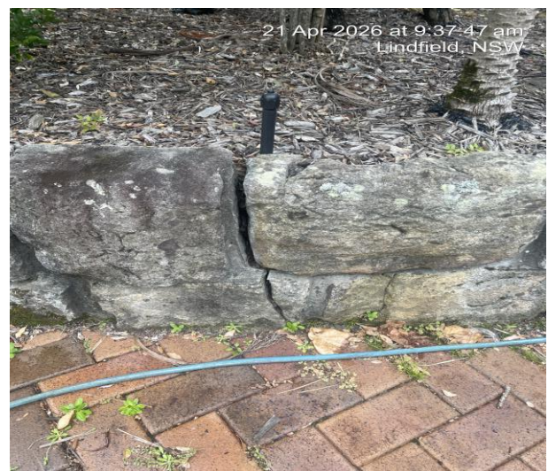
Photo 144 - Cracking observed to mortar
