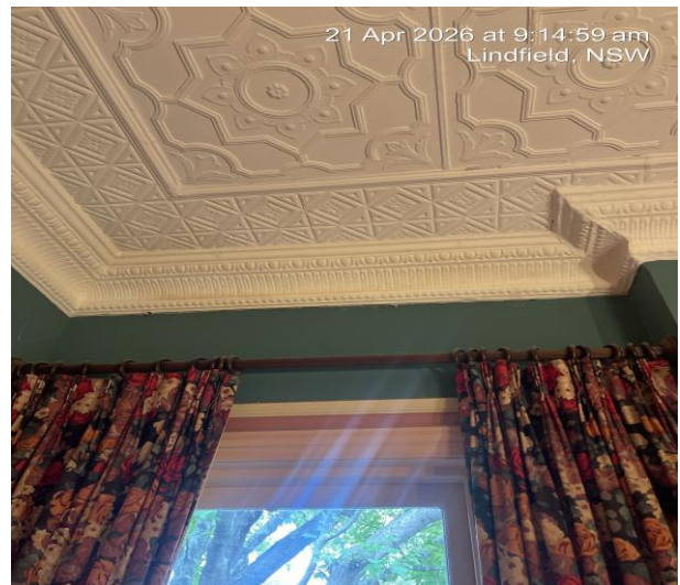
Photo 46 - Cracking observed to wall and coving
