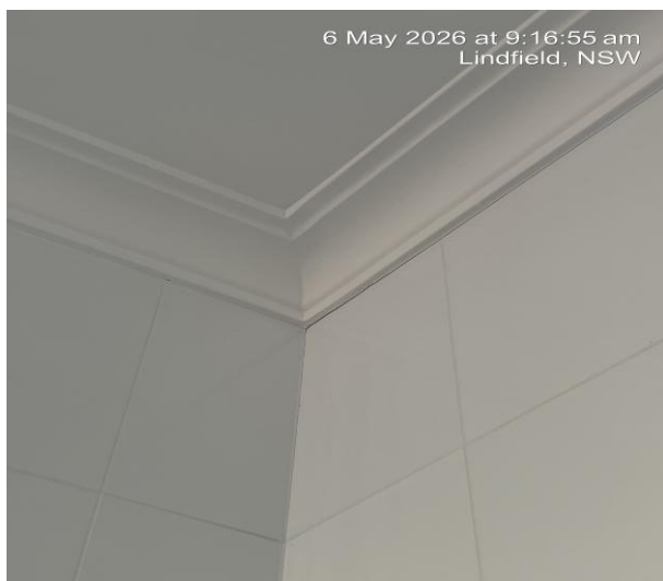
Photo 53 – Cracking observed to grout and coving
