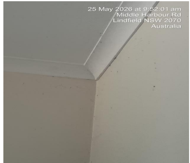
Photo 152 – Cracking observed to coving
