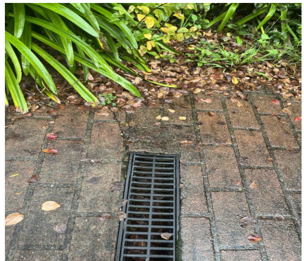
Photo 220 – Cracking observed to pavers
