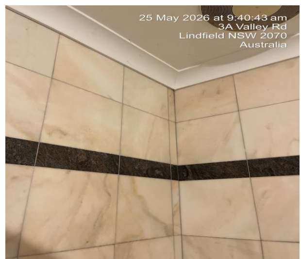
Photo 114 – Cracking observed to coving
