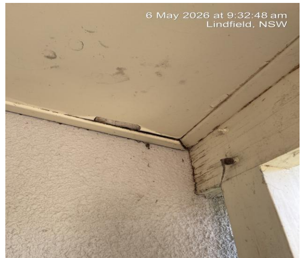
Photo 118 – Deterioration observed to ceiling and framing
