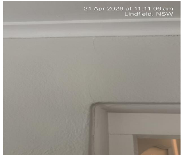
Photo 14 - Vertical cracking observed to wall
