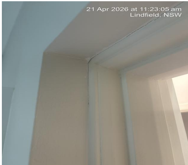
Photo 55 – Cracking observed to door frame
