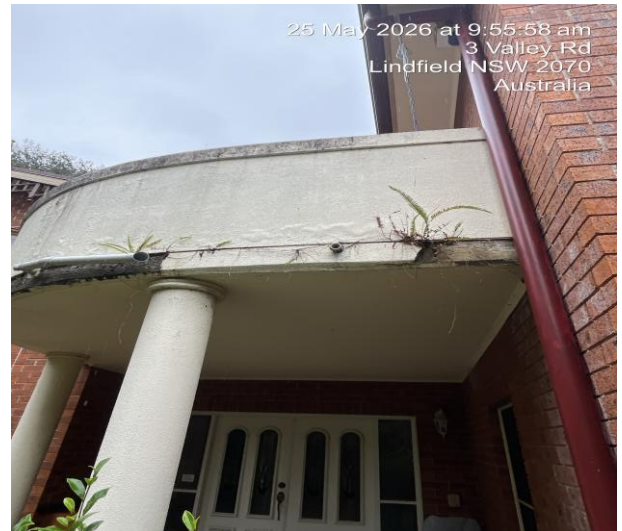
Photo 176 – Water ingress and damage observed to upturn
