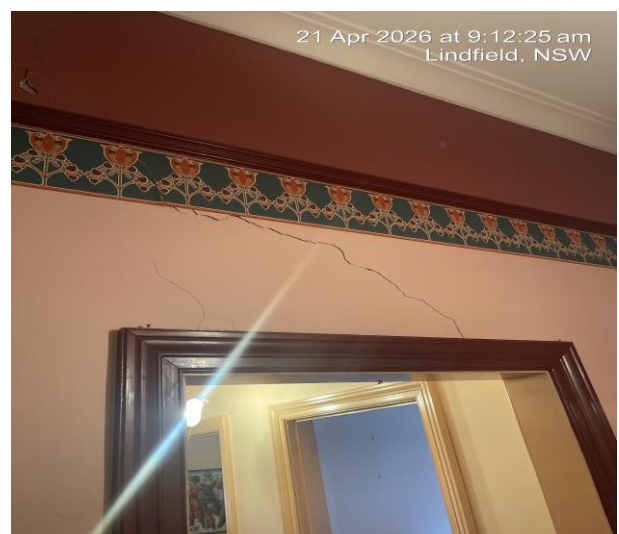
Photo 30 – 45° crack observed to wall
