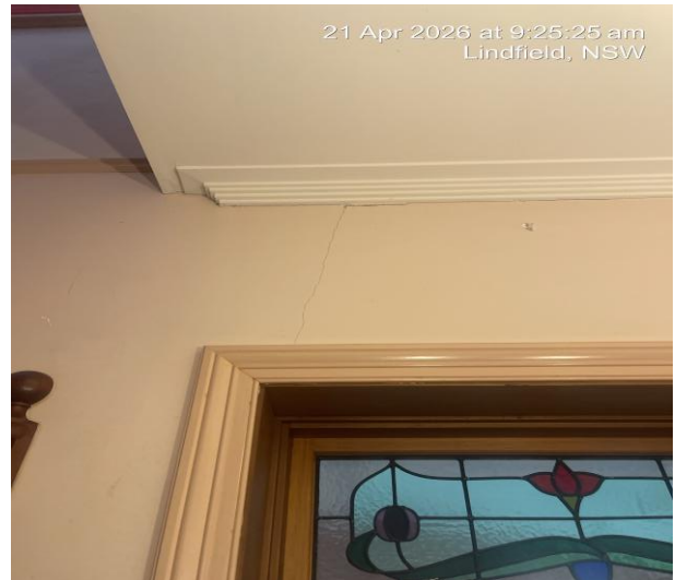
Photo 98 – Vertical crack observed to wall
