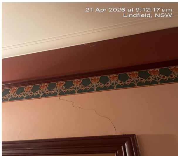
Photo 27 – 45° crack observed to wall
