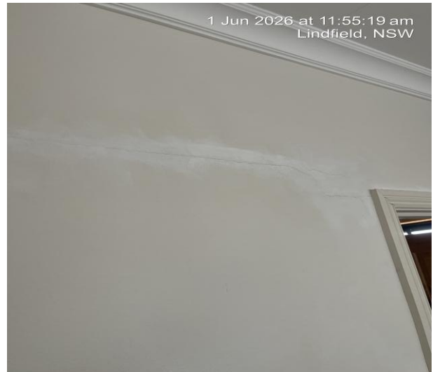
Photo 122 - Cracking observed to render with signs of attempts to repair
