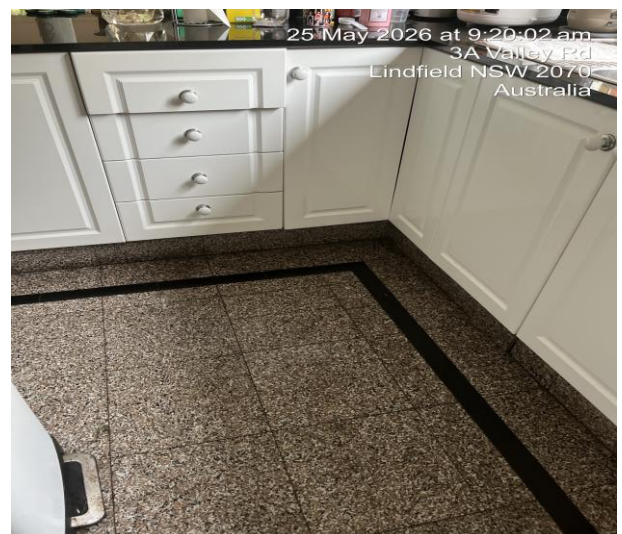
Photo 18 – Loose tiling observed
