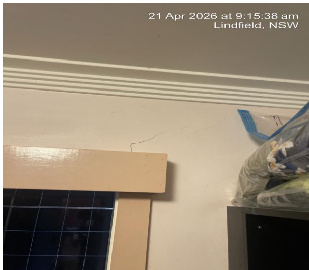
Photo 51 - Cracking observed to wall
