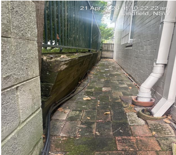
Photo 79 – Overturning of timber retaining wall observed
