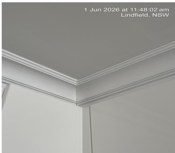
Photo 71 – Movement observed to coving
