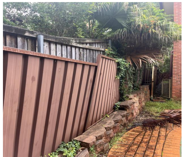
Photo 192 – Overturning of fence observed
