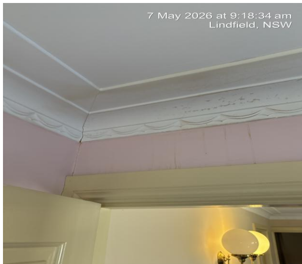
Photo 69 – Cracking and water damage observed to wall, coving and ceiling
