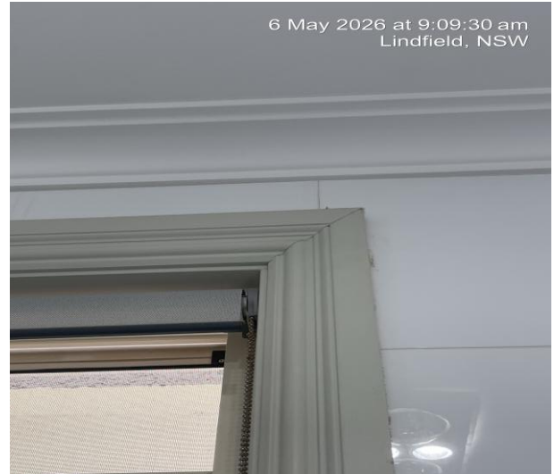
Photo 20 - Cracking observed to grout and window frame
