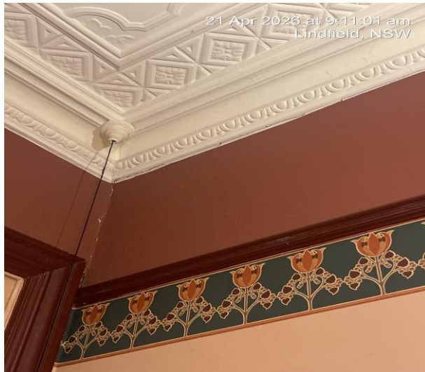
Photo 19 – Cracking observed to wall
