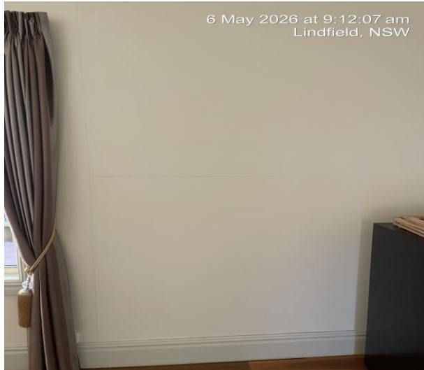
Photo 31 – Horizontal crack observed to gyprock
