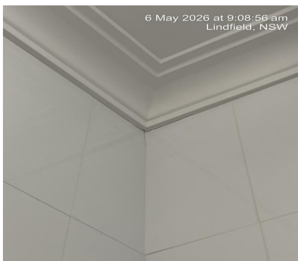
Photo 17 – Cracking observed to grout and coving
