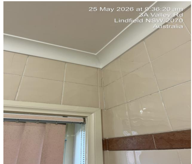
Photo 98 – Cracking observed to tiles
