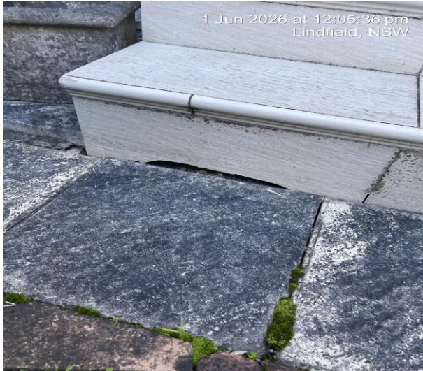
Photo 169 – Damage observed to tile
