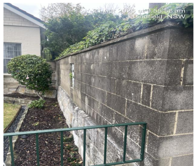
Photo 162 – Rear boundary block wall exhibiting outward bowing toward neighboring property
