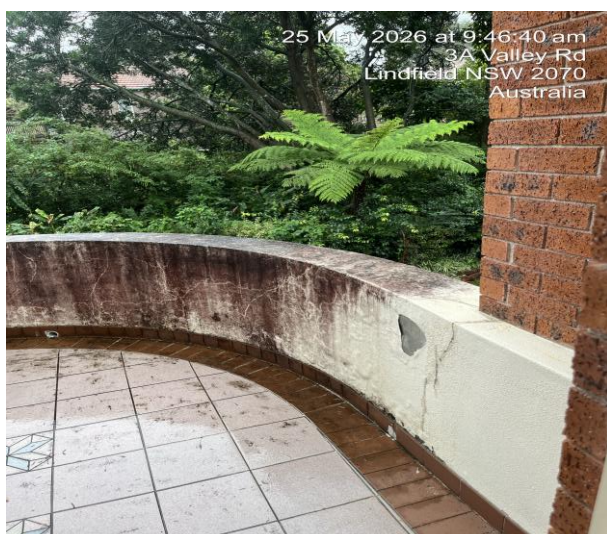
Photo 143 – Water ingress and delamination of paint observed
