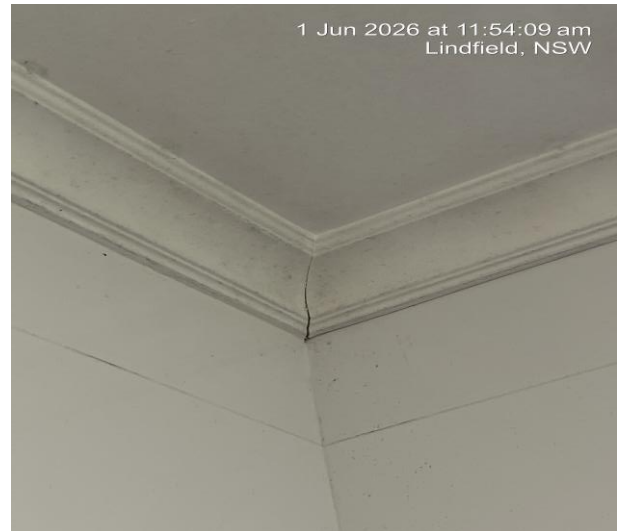
Photo 110 – Movement observed to coving
