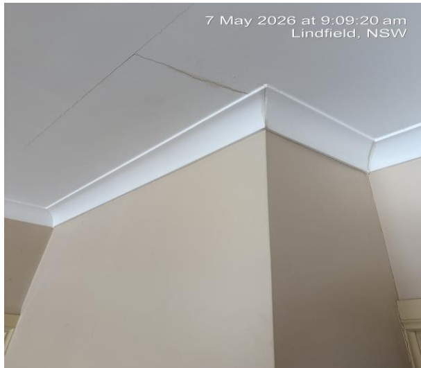
Photo 25 - Cracking observed to ceiling and coving
