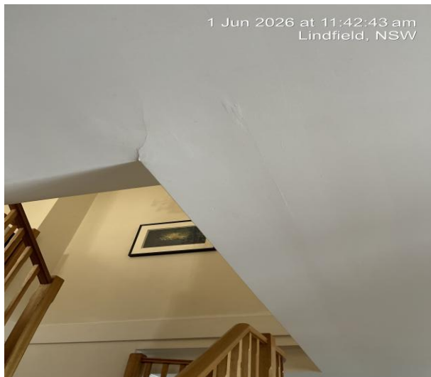
Photo 33 – Damage observed to ceiling
