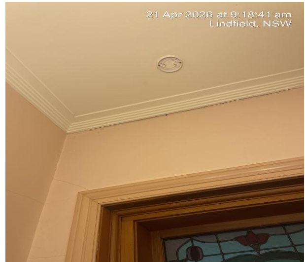
Photo 68 – Cracking observed to wall and movement observed to coving
