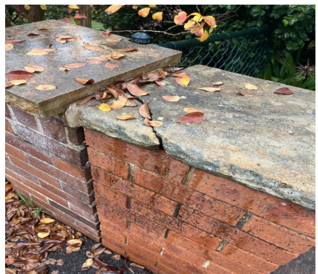
Photo 222 – Cracking observed to stone
