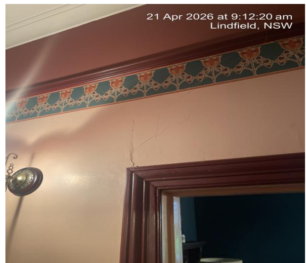
Photo 28 - Cracking observed to wall
