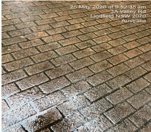
Photo 157 – Cracking observed to paver
