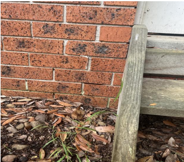
Photo 207 – Gaps observed to mortar
