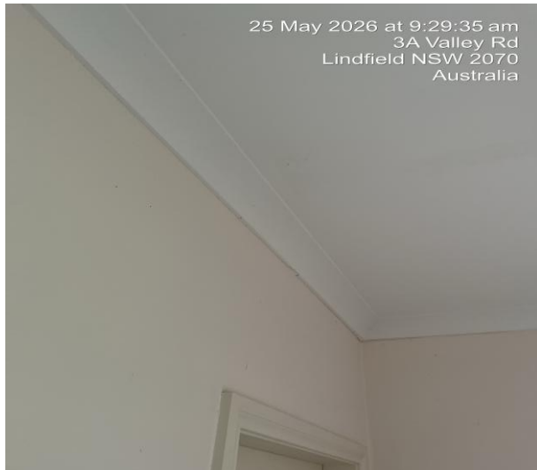
Photo 67 - Cracking observed to coving
