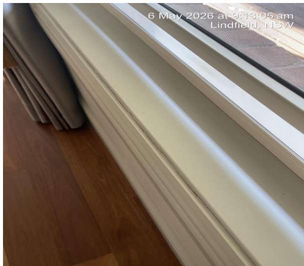
Photo 33 – Cracking observed to window frame
