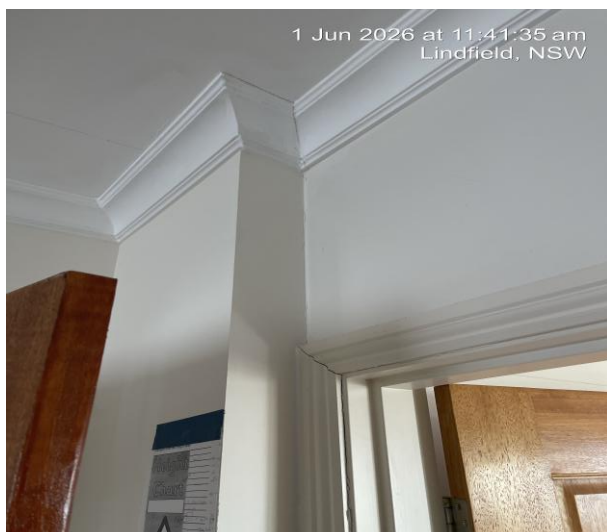
Photo 23 – Cracking observed to door frame and coving
