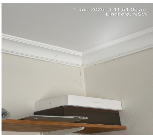
Photo 89 - Cracking observed to coving and render
