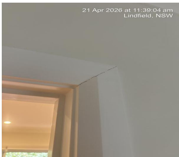
Photo 107 – Cracking observed to door frame
