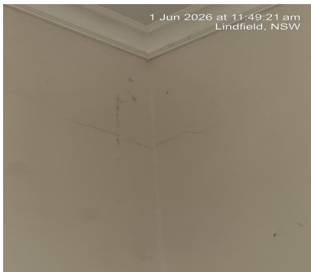
Photo 77 – Cracking observed to render
