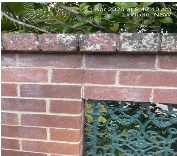
Photo 159 - Cracking observed to brick fence
