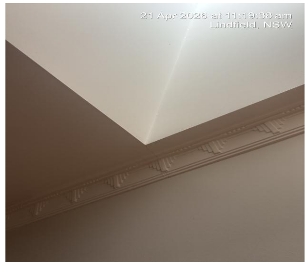
Photo 40 – Cracking observed to ceiling
