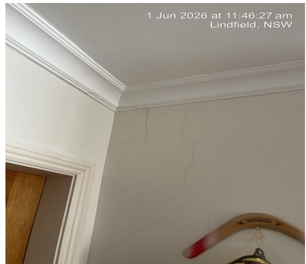
Photo 58 – Cracking observed to render
