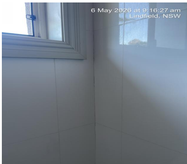
Photo 51 - Cracking observed to grout
