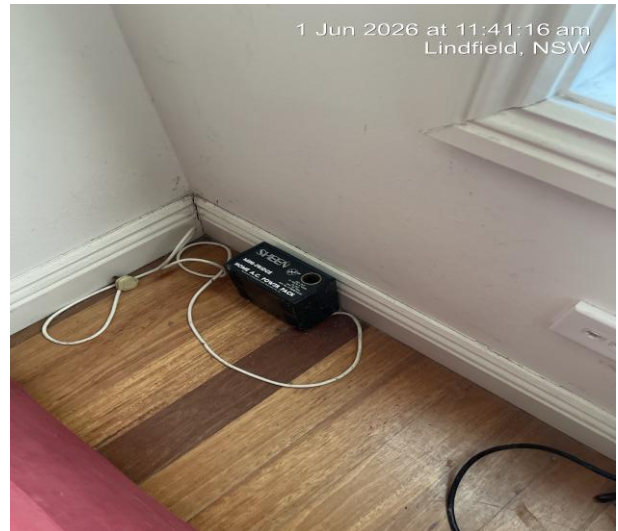
Photo 20 – Movement observed to skirting
