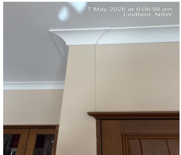
Photo 22 - Cracking observed to wall and coving
