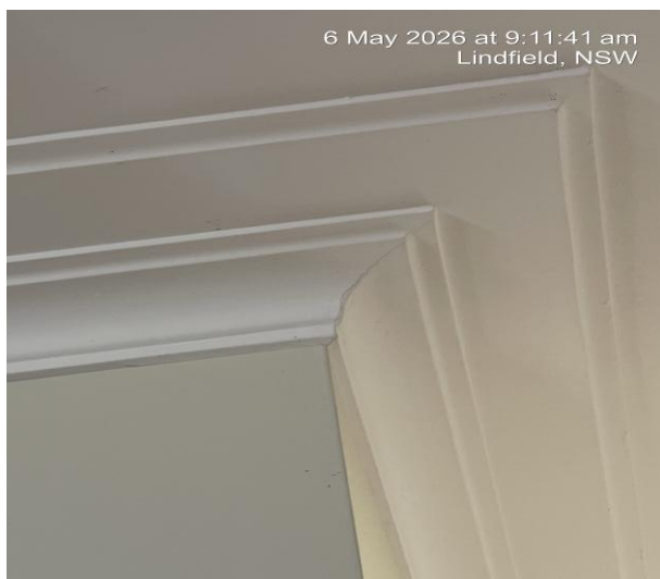
Photo 29 – Cracking observed to coving
