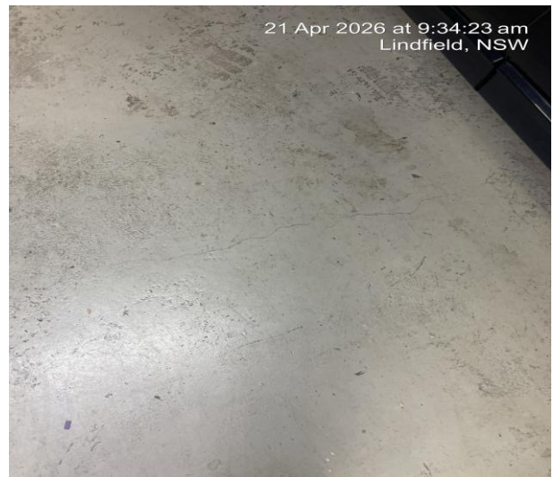
Photo 130 – Cracking observed to concrete
