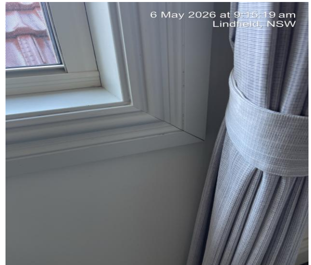
Photo 44 – Cracking observed to window frame
