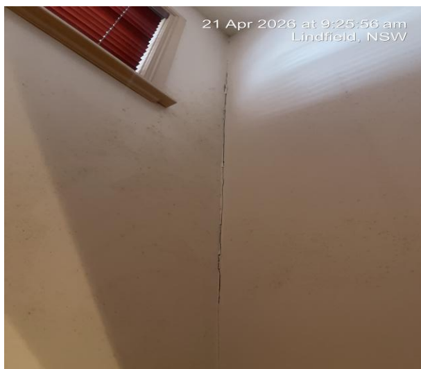
Photo 101 – Vertical crack observed to wall junction
