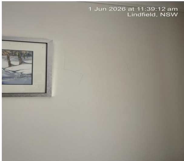
Photo 13 – Cracking observed to render
