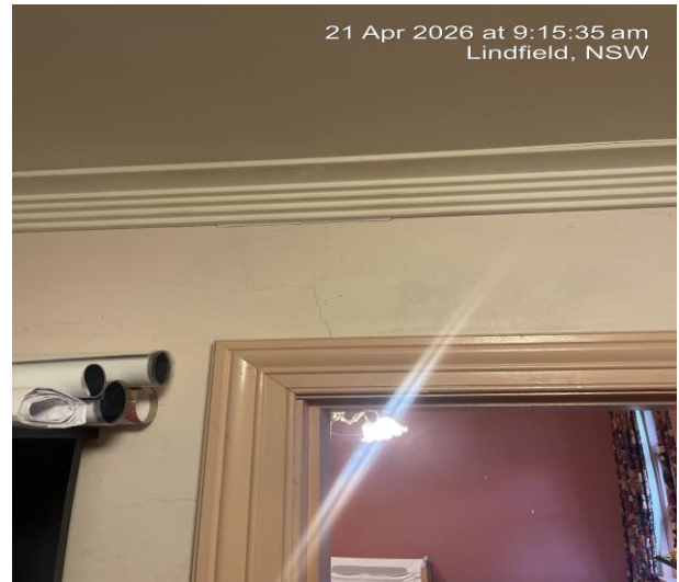
Photo 50 – Cracking observed to wall
