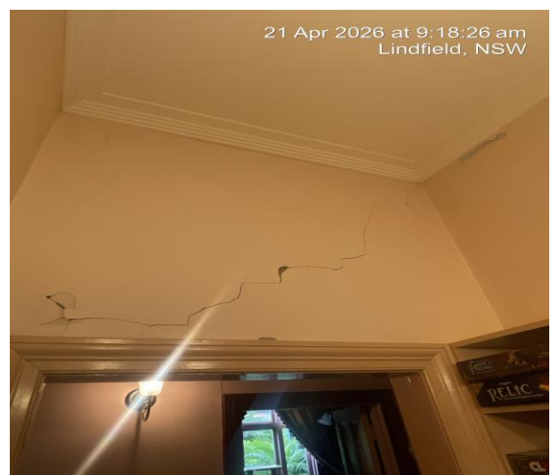
Photo 66 – 45° crack observed to wall
