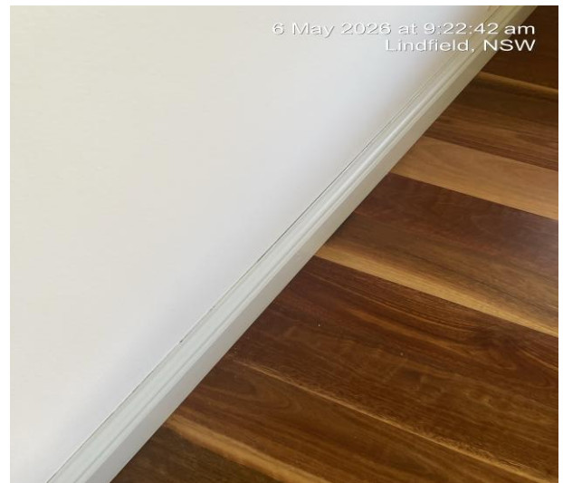
Photo 82 – Cracking observed to skirting
