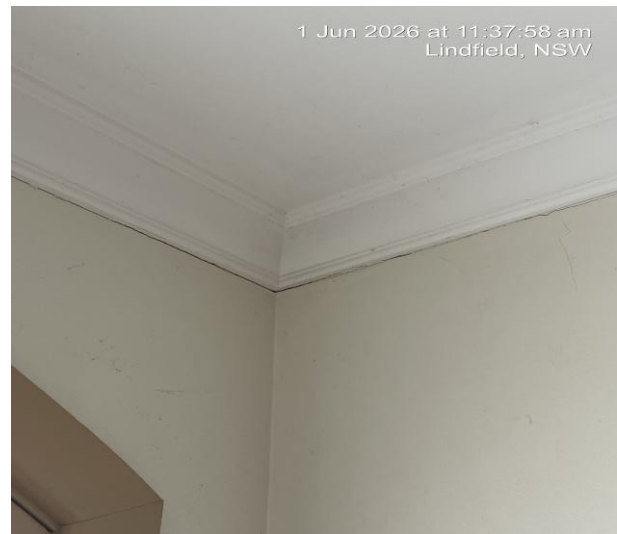
Photo 2 – Movement observed to coving
