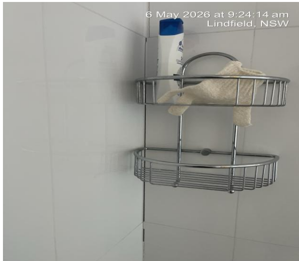
Photo 91 – Cracking observed to grout
