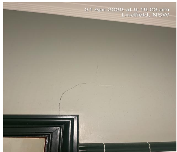
Photo 72 – Cracking observed to wall
