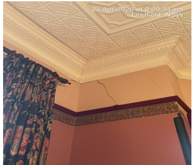
Photo 8 – Cracking observed to wall and coving
