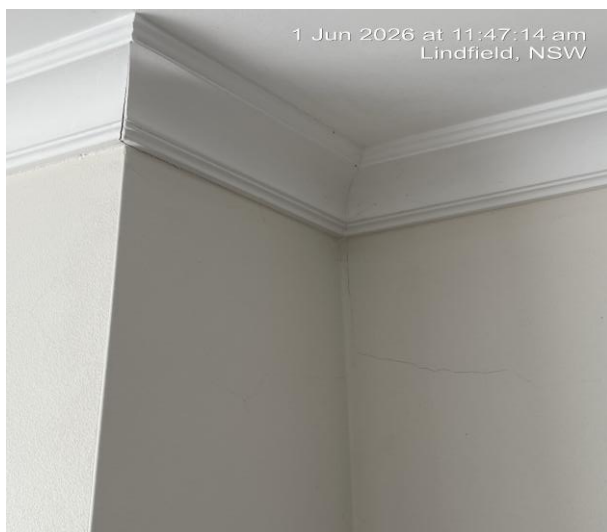
Photo 65 – Cracking observed to coving
