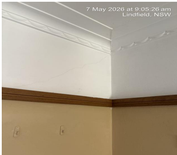
Photo 9 - Cracking observed to wall and coving
