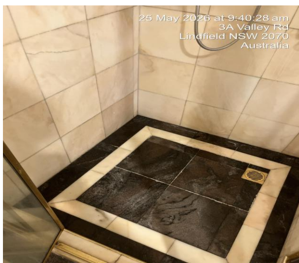
Photo 113 – Cracking observed to tiles
