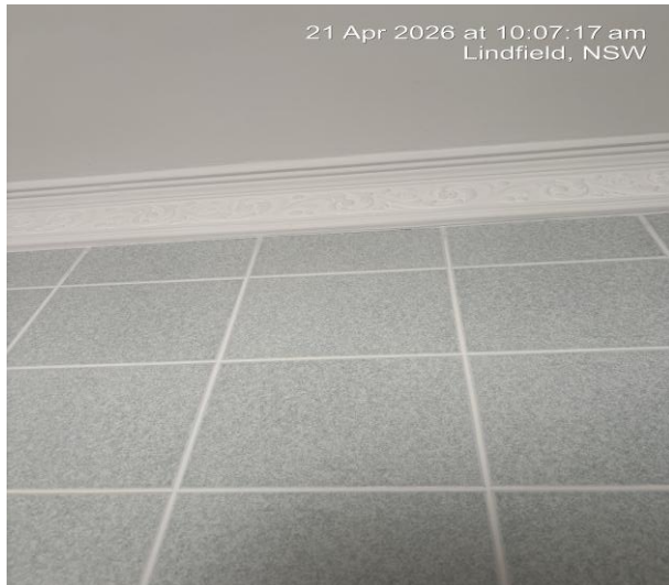
Photo 37 – Movement observed to tiles and coving
