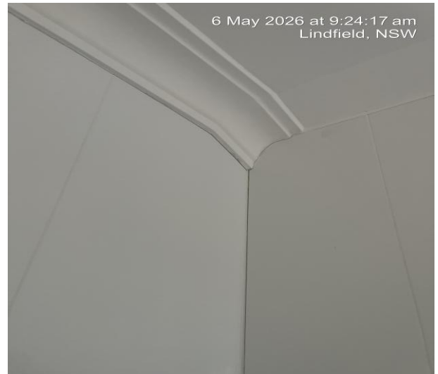
Photo 92 – Cracking observed to grout and coving
