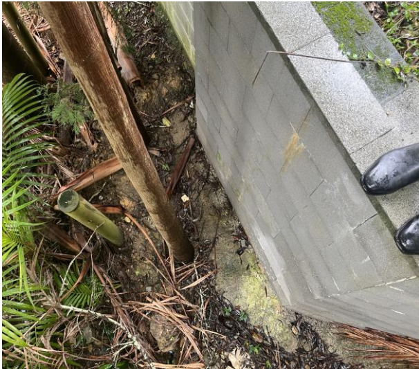
Photo 211 – Efflorescence observed to block retaining wall
