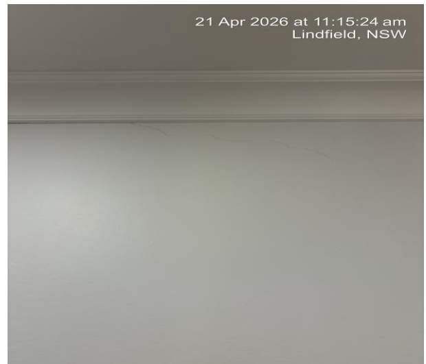
Photo 28 – Cracking observed to wall
