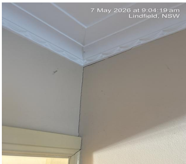
Photo 3 – Cracking observed to wall
