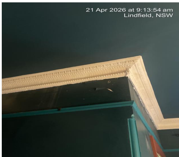
Photo 39 – Cracking observed to wall and coving
