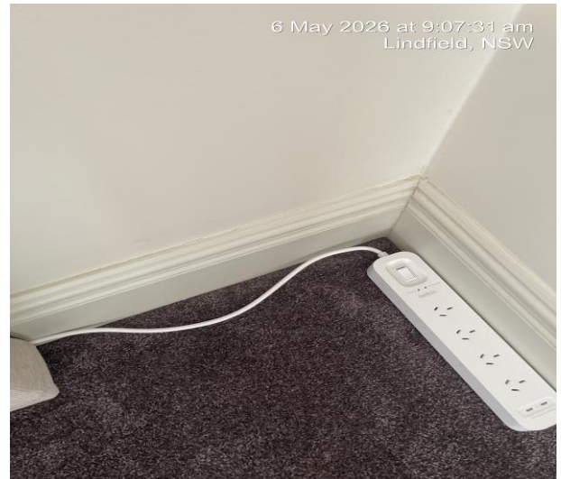
Photo 8 – Cracking observed to skirting
