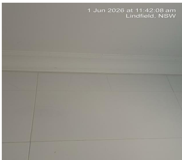
Photo 29 - Cracking observed to tiles
