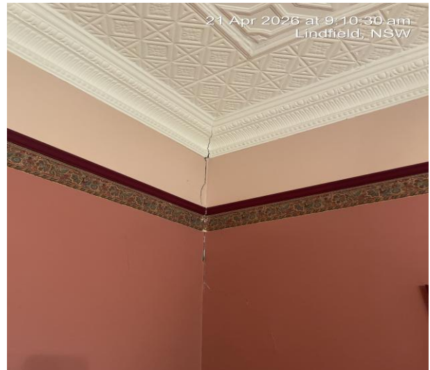
Photo 14 – Vertical cracking observed to wall and coving
