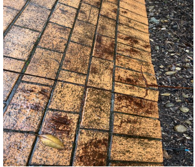
Photo 194 – Cracking observed to paver
