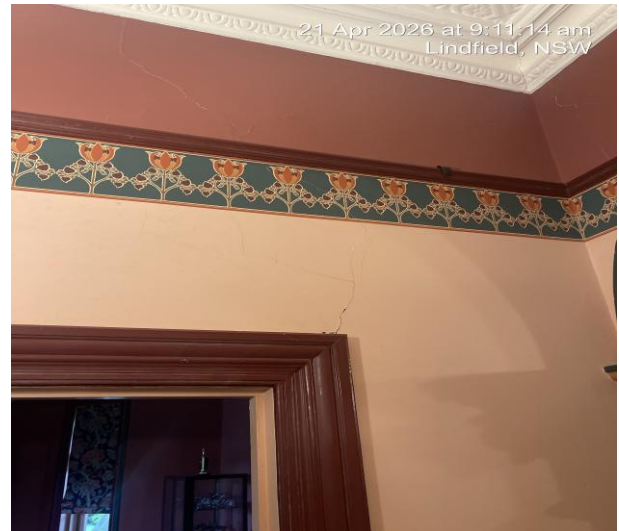
Photo 20 - Cracking observed to wall
