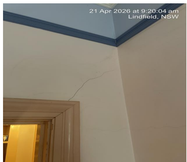
Photo 78 – 45° crack observed to wall
