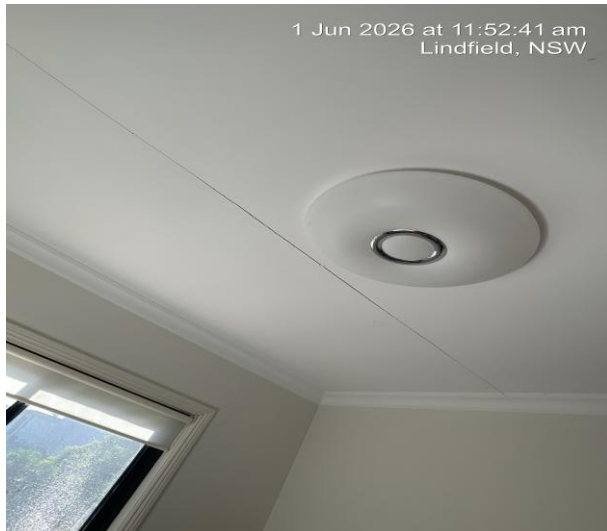
Photo 97 – Cracking observed to ceiling
