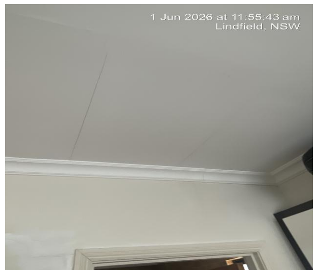
Photo 126 - Cracking observed to ceiling
