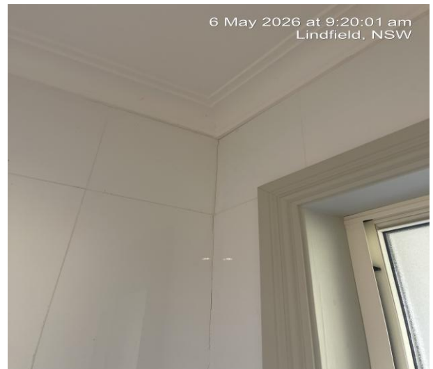
Photo 70 – Cracking observed to grout and coving
