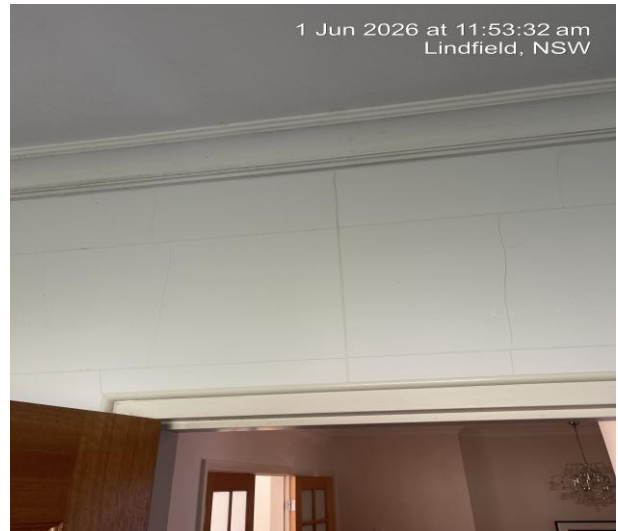
Photo 104 – Cracking observed to tiles
