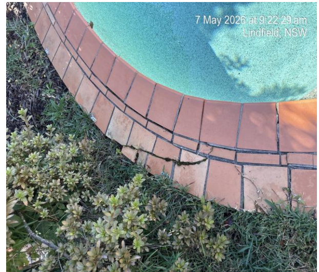
Photo 82 – Cracking observed to pavers
