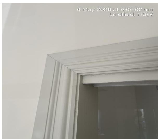
Photo 11 - Cracking observed to doorframe
