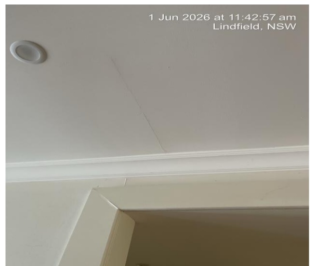
Photo 36 - Cracking observed to ceiling
