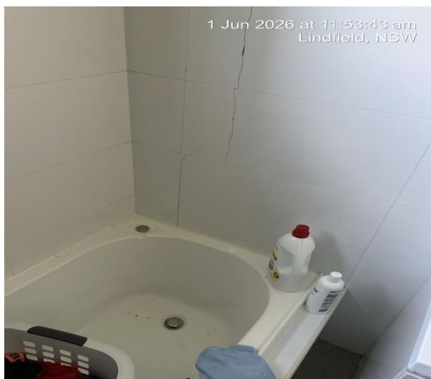
Photo 107 – Cracking observed to render
