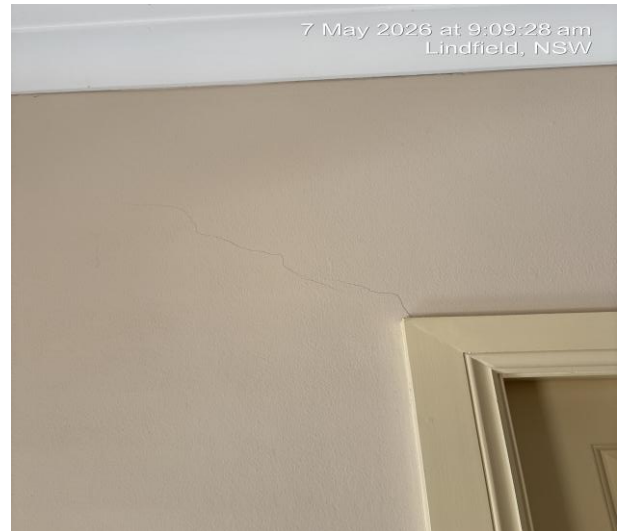
Photo 26 - Cracking observed to wall
