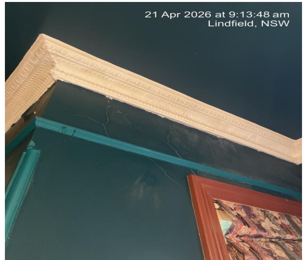
Photo 38 – Cracking observed to wall and coving
