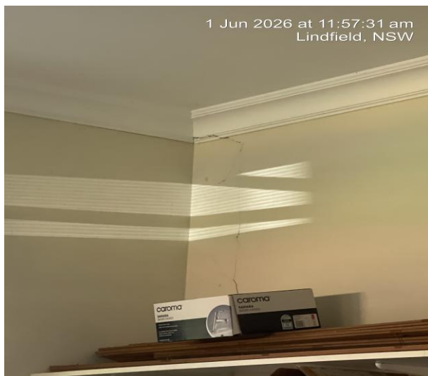
Photo 135 - Cracking observed to render
