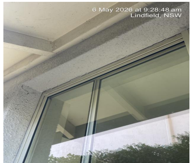
Photo 106 – Cracking observed to render
