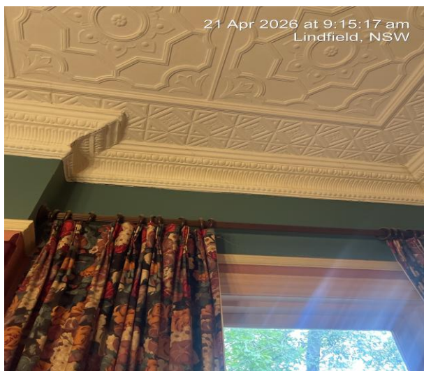
Photo 47 - Cracking observed to wall and coving
