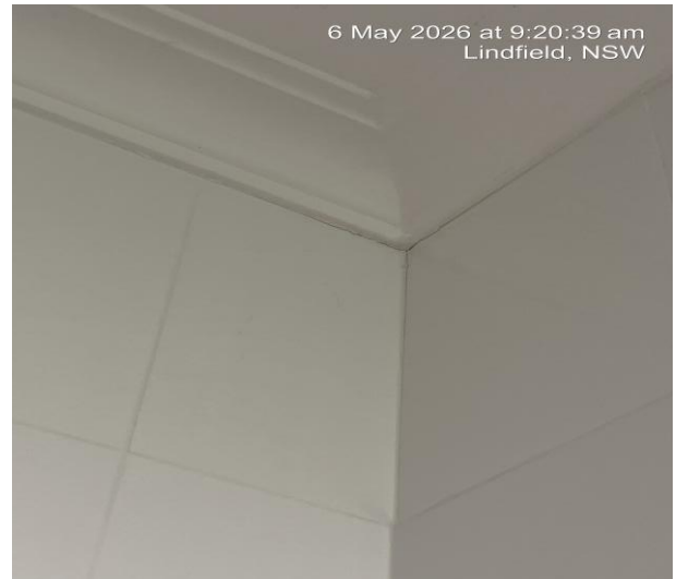
Photo 74 – Cracking observed to grout and coving
