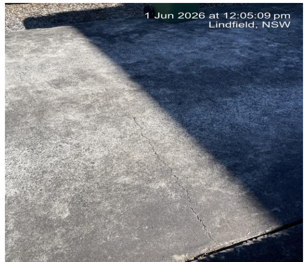
Photo 166 - Cracking observed to concrete
