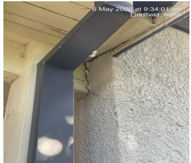
Photo 128 – Deterioration observed to ceiling and framing
