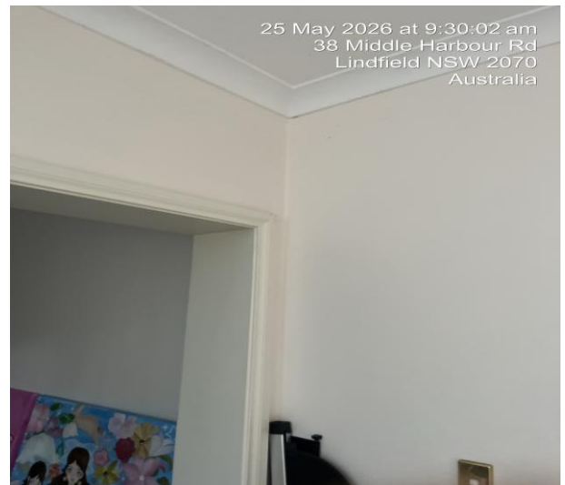
Photo 70 – Cracking observed to coving
