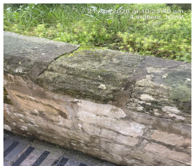
Photo 84 – Cracking observed to mortar
