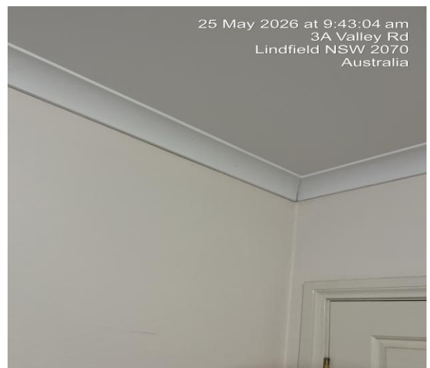
Photo 126 – Cracking observed to coving
