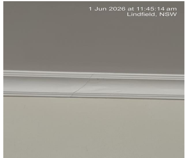
Photo 50 – Damage observed to coving
