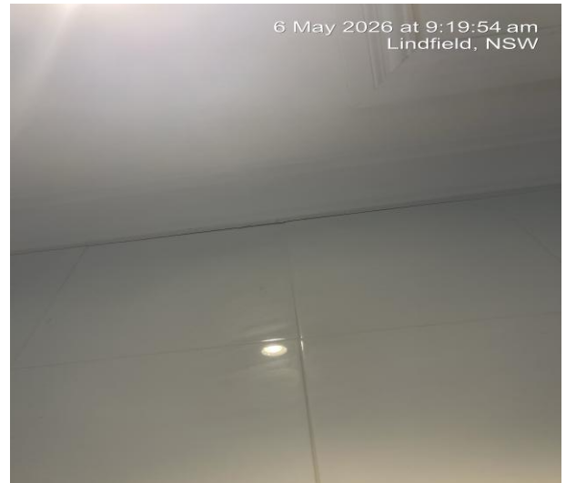
Photo 68 - Movement observed to coving
