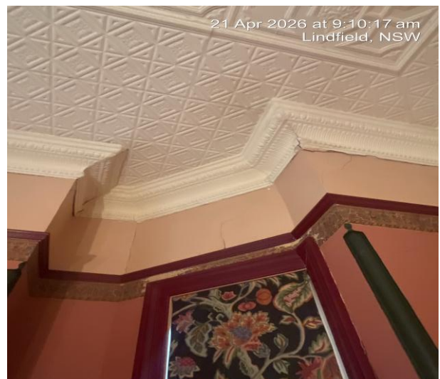
Photo 12 – Cracking observed to wall and coving
