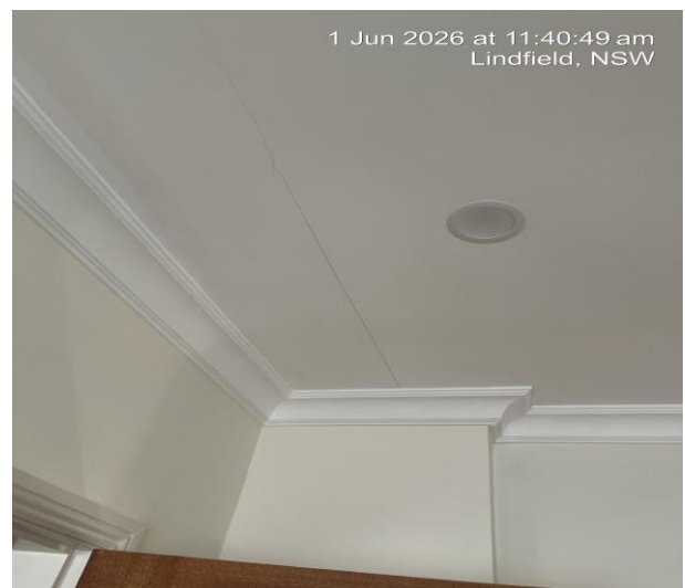
Photo 18 – Cracking observed to ceiling
