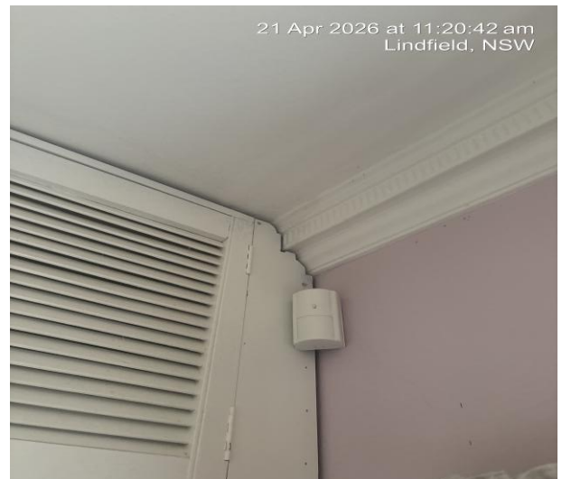
Photo 46 – Cracking observed to ceiling
