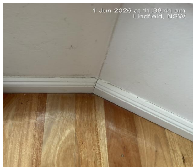
Photo 10 – Cracking observed to skirting
