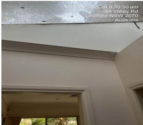
Photo 73 – Cracking observed to coving
