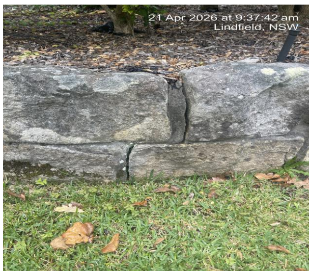
Photo 143 – Cracking observed to mortar
