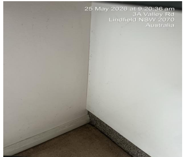
Photo 20 – Cracking observed to skirting
