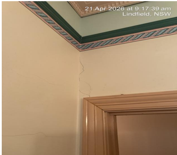
Photo 61 – Cracking observed to wall
