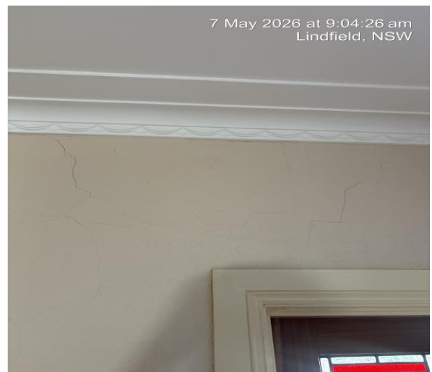
Photo 4 – Cracking observed to wall
