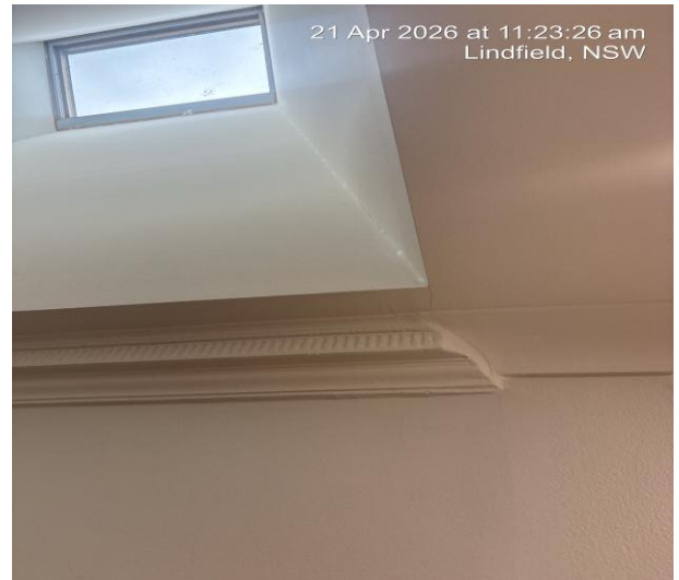
Photo 56 – Cracking observed to coving and ceiling
