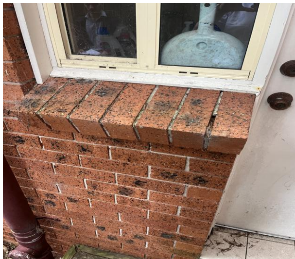
Photo 183 – Damage observed to mortar
