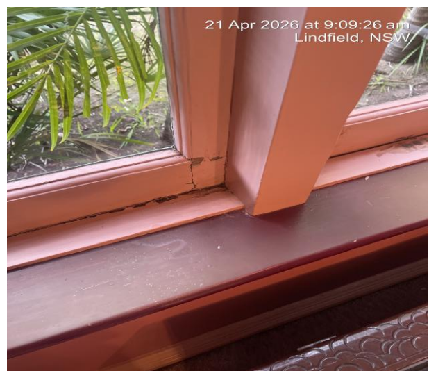
Photo 6 – Cracking observed to window frame
