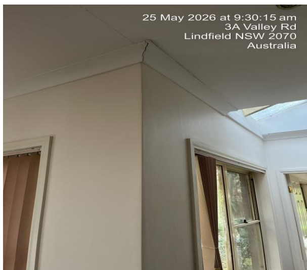
Photo 71 – Cracking observed to coving
