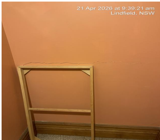
Photo 147 – Horizontal crack observed to wall
