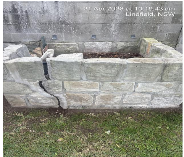
Photo 74 – Settlement observed to stone wall
