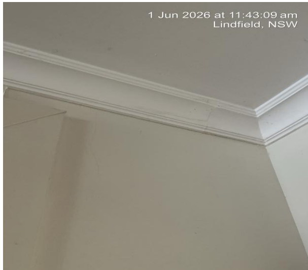
Photo 37 – Cracking observed to coving
