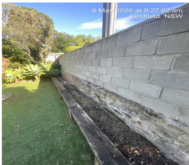
Photo 101 – Overturning observed to brick retaining wall
