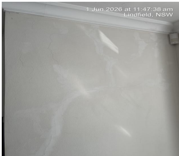
Photo 69 – Cracking observed to render with signs of attempts to repair
