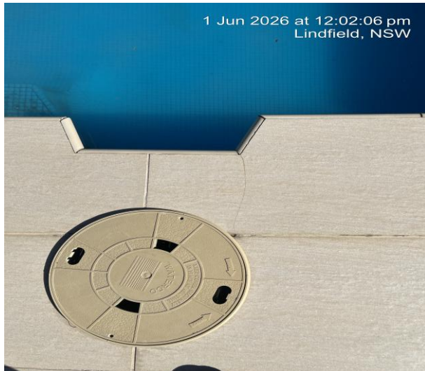
Photo 151 - Cracking observed to tiles
