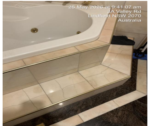
Photo 116 – Cracking observed to tiles
