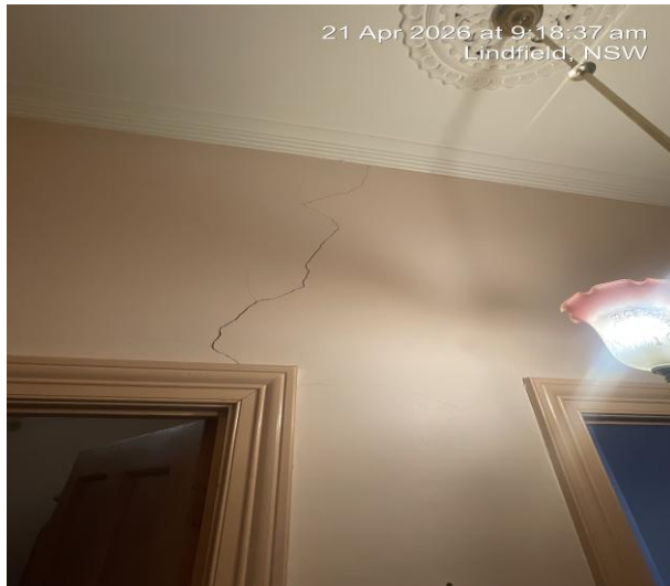
Photo 67 – Vertical crack observed to wall
