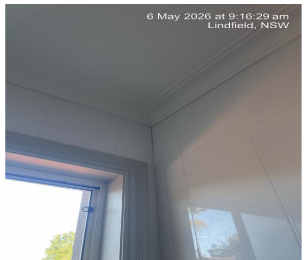
Photo 52 – Cracking observed to grout and coving
