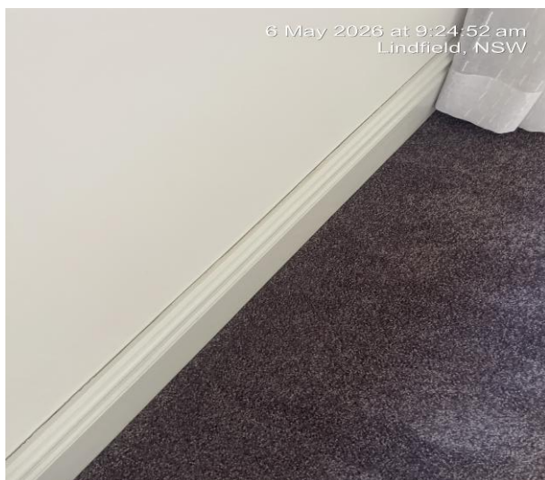
Photo 95 – Cracking observed to skirting
