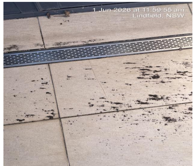
Photo 142 – Cracking observed to tiles
