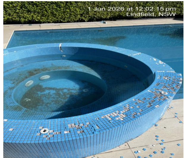
Photo 152 – Dislodgement of tiles observed
