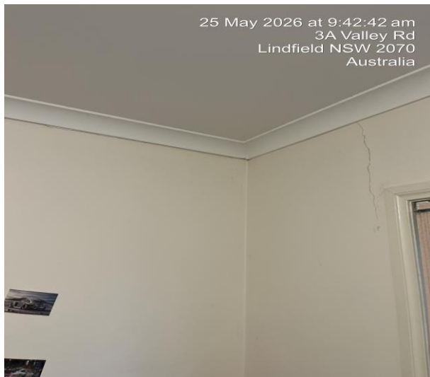
Photo 123 – Cracking observed to wall
