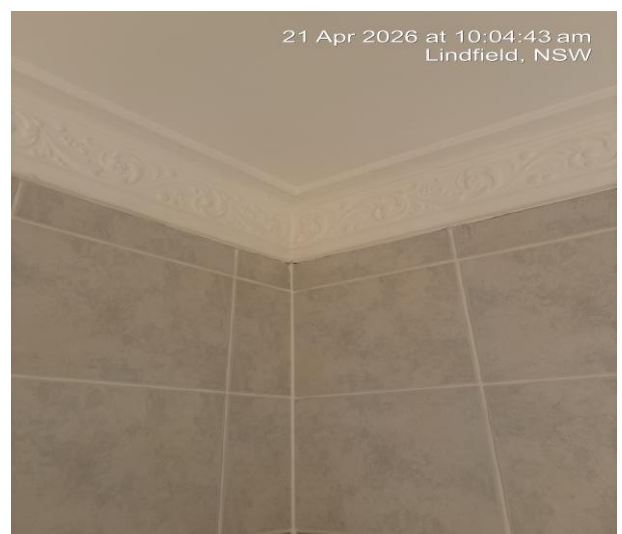
Photo 24 – Cracking observed to coving
