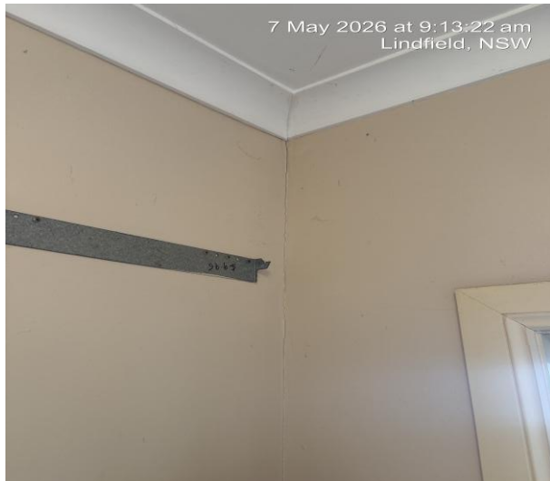
Photo 43 – Cracking observed to wall and coving
