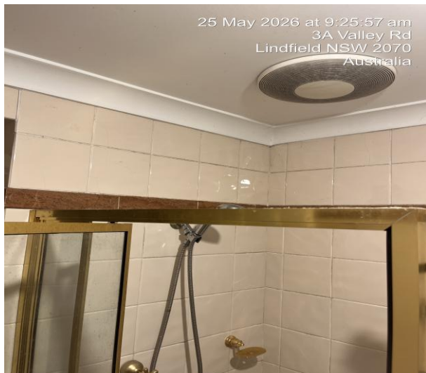
Photo 45 – Cracking observed to tiles
