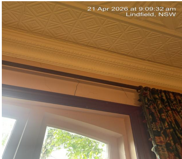
Photo 7 – Vertical cracking observed to wall
