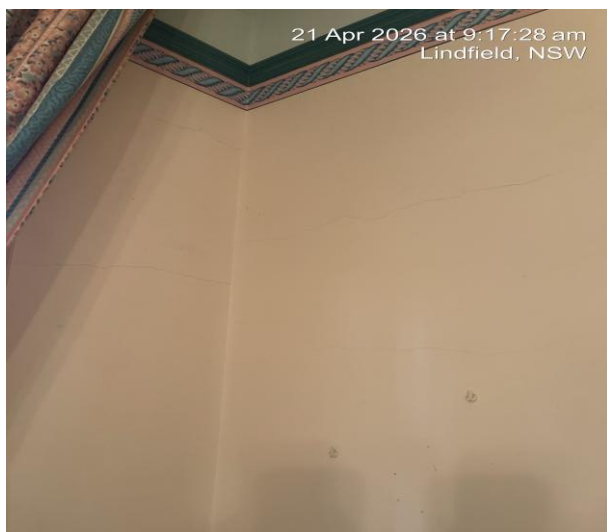
Photo 59 – Horizontal cracking observed to wall
