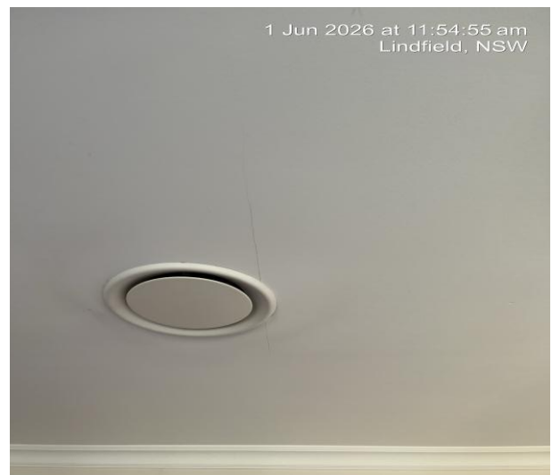
Photo 118 - Cracking observed to ceiling
