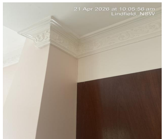
Photo 30 - Cracking observed to wall and coving
