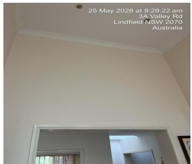
Photo 66 - Cracking observed to coving
