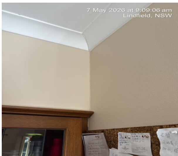
Photo 23 - Cracking observed to wall and coving
