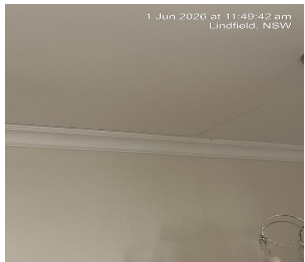
Photo 78 – Cracking observed to ceiling
