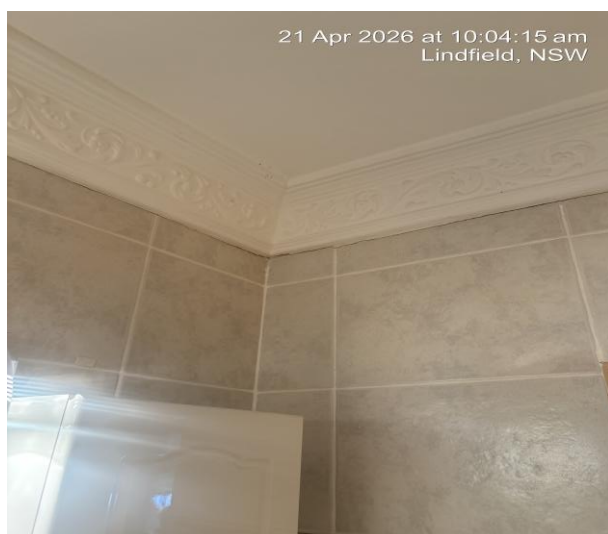
Photo 23 – Cracking observed to coving
