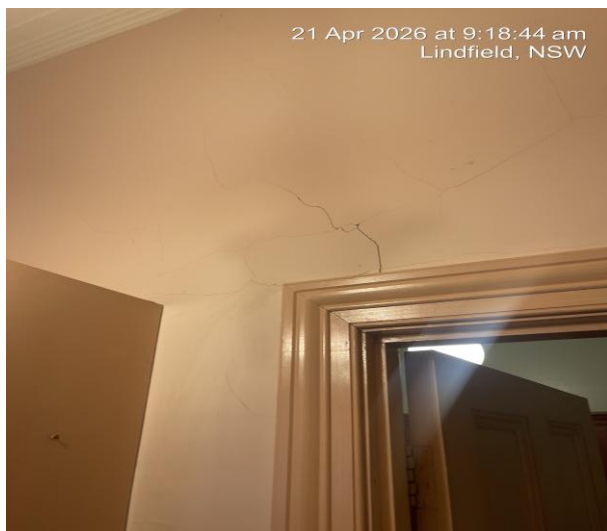
Photo 69 – Cracking observed to wall
