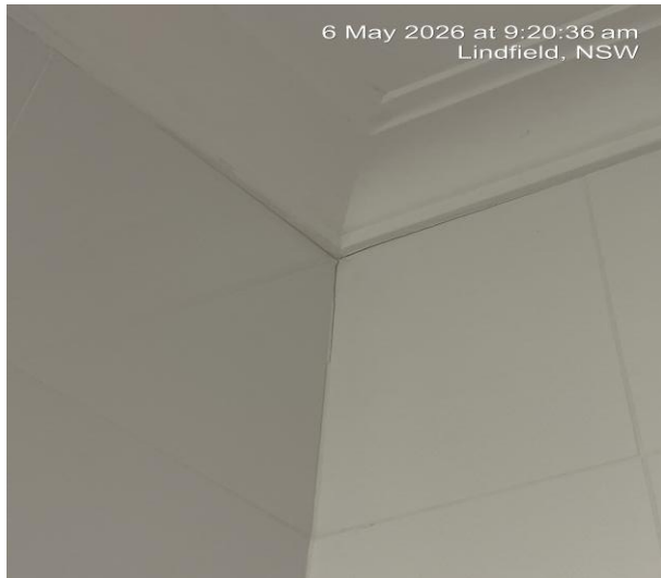
Photo 73 – Cracking observed to grout and coving
