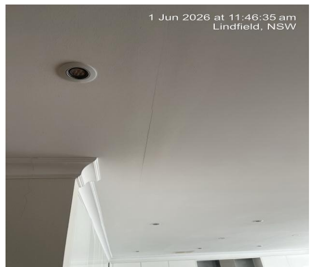
Photo 60 – Cracking observed to ceiling
