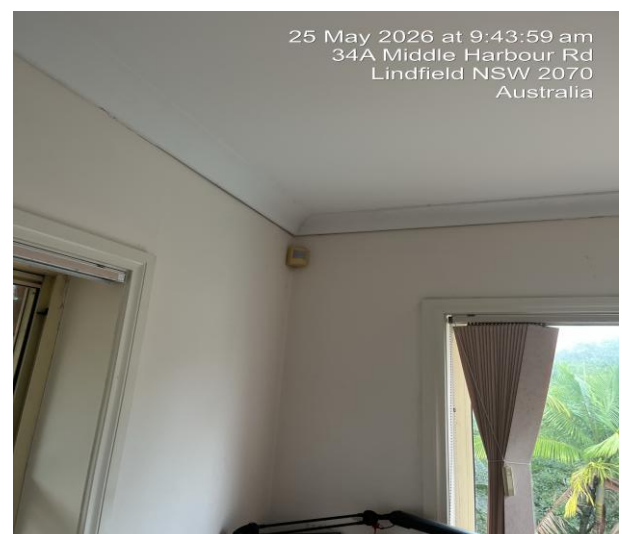
Photo 132 – Movement observed to coving
