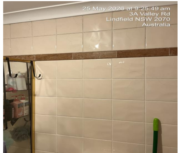
Photo 44 – Cracking observed to tiles
