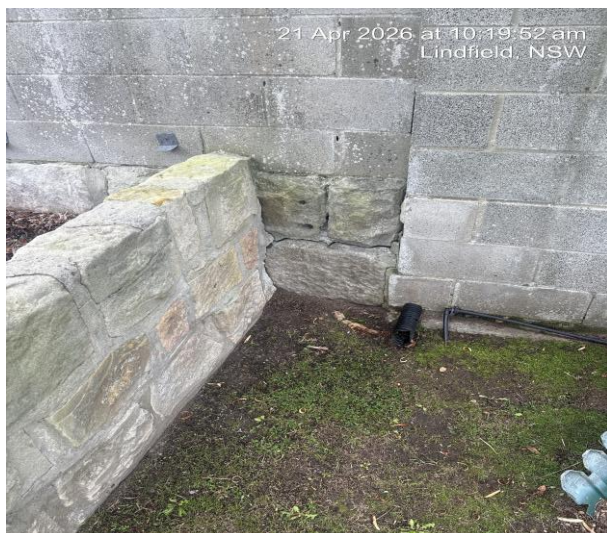
Photo 75 – Cracking observed to mortar
