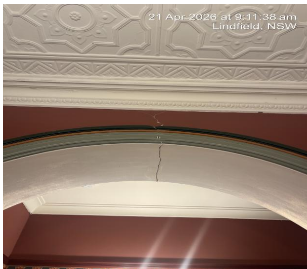
Photo 21 - Cracking observed to archway
