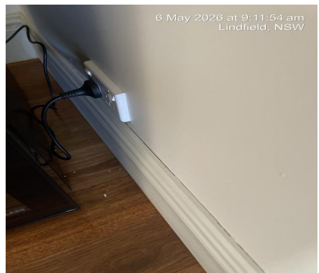
Photo 30 – Movement observed to skirting
