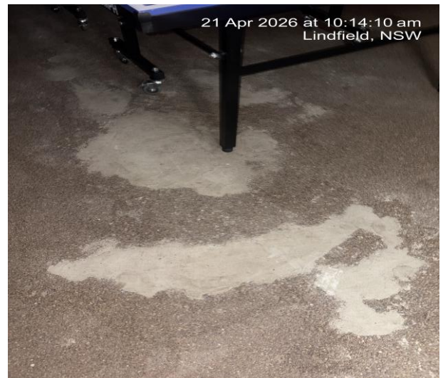
Photo 52 – Repair patching observed to epoxy pebble flooring
