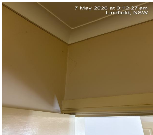
Photo 39 – Cracking observed to wall
