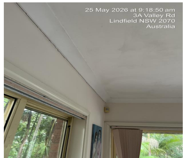
Photo 4 – Cracking observed to coving
