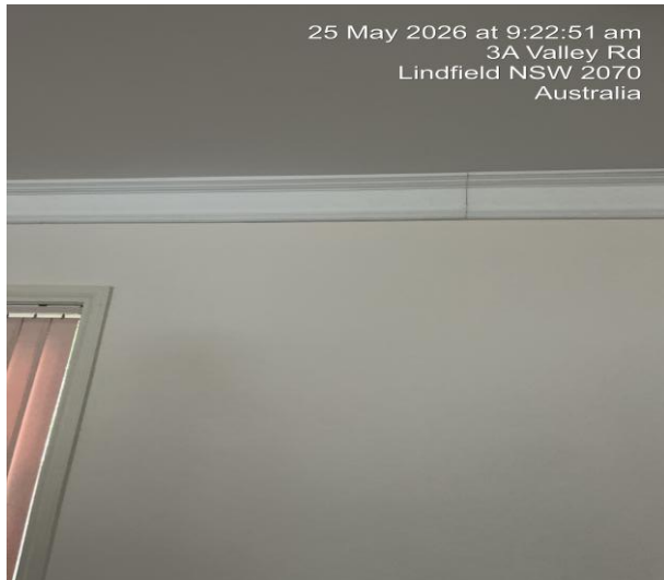
Photo 31 – Cracking observed to coving
