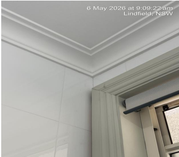
Photo 19 – Cracking observed to grout and coving
