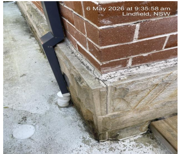
Photo 140 – Cracking observed to mortar
