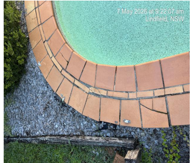
Photo 80 - Cracking observed to pavers
