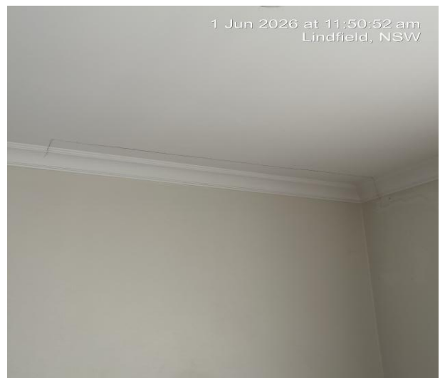
Photo 88 - Cracking observed to ceiling and render with signs of attempts to repair
