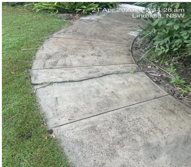
Photo 153 – Cracking observed to footpath
