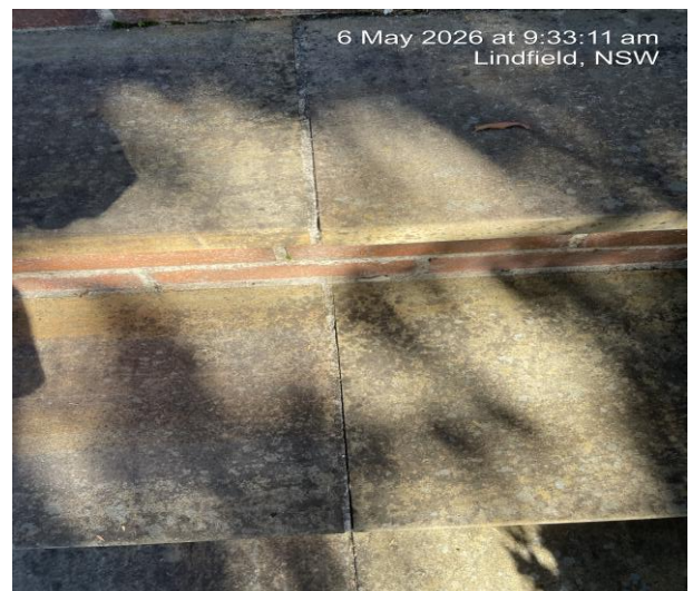
Photo 120 – Cracking observed to grout
