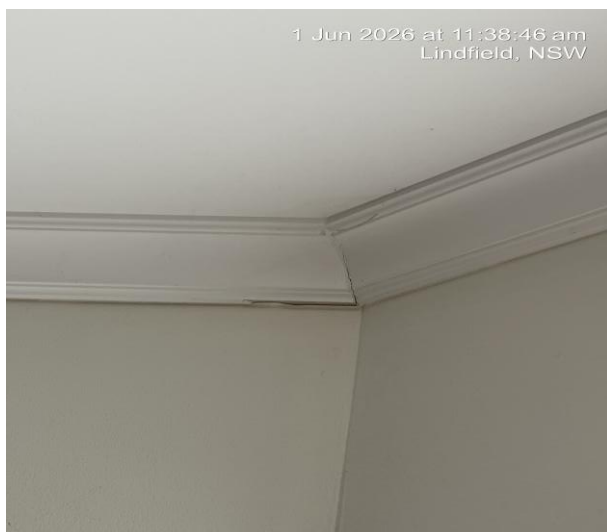
Photo 11 – Cracking and delamination of paint observed to coving
