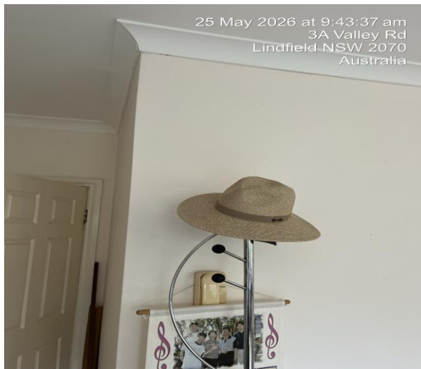
Photo 129 – Cracking observed to coving
