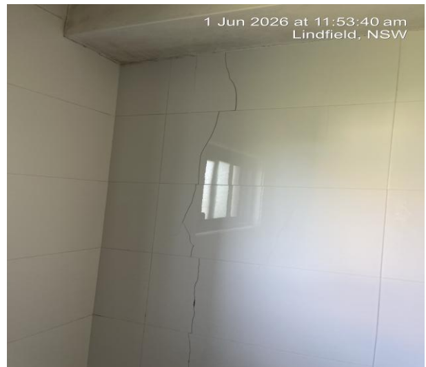
Photo 106 - Cracking observed to render
