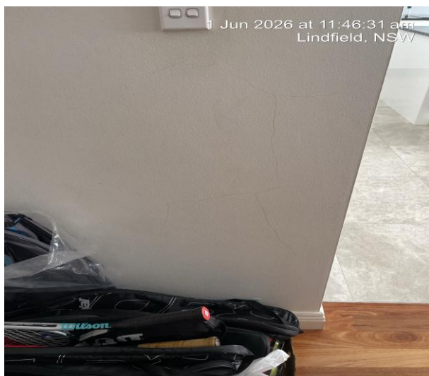
Photo 59 – Cracking observed to render
