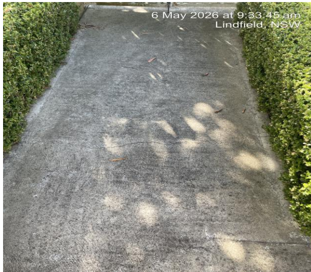
Photo 127 – Cracking observed to concrete
