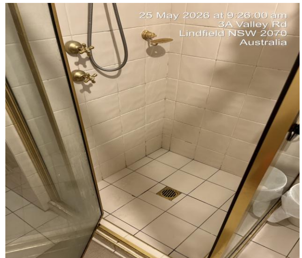
Photo 46 – Cracking observed to tiles
