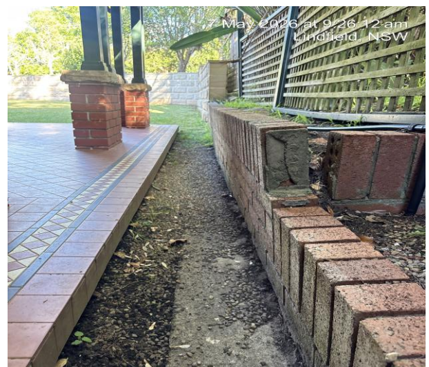
Photo 90 – Cracking and bowing observed to brick wall
