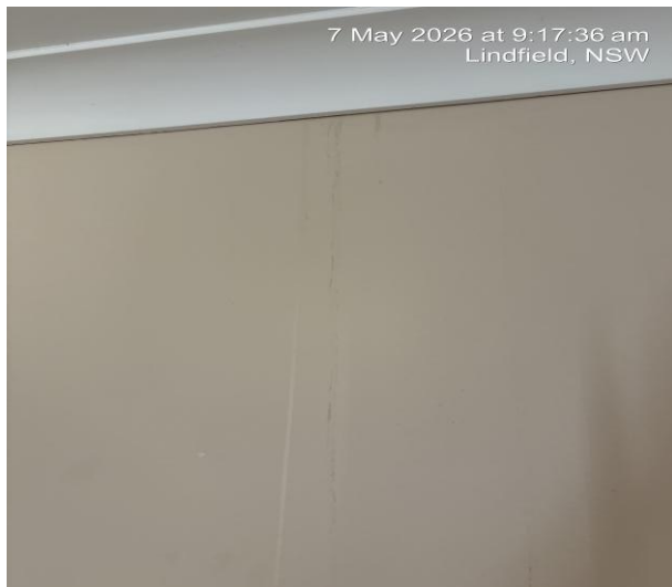
Photo 63 – Water damage observed to wall
