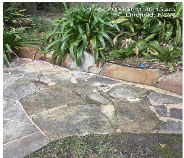
Photo 94 – Cracking observed to mortar
