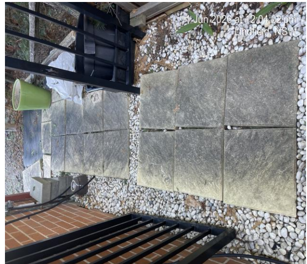
Photo 160 – Settlement observed to pavers
