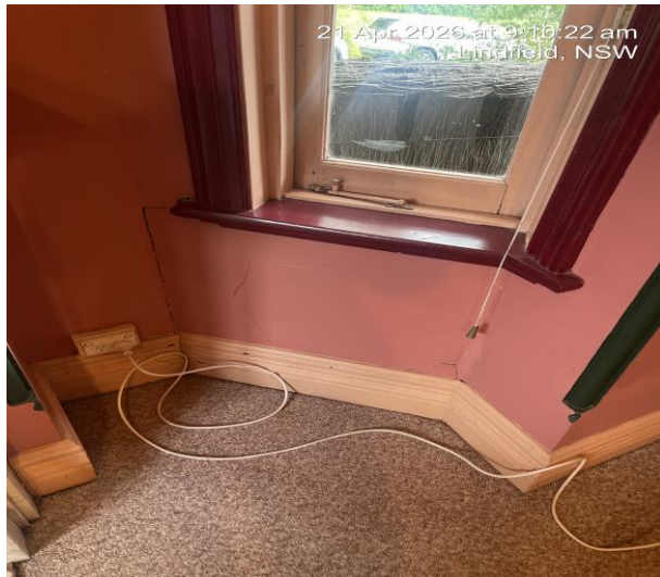
Photo 13 – Vertical cracking observed to wall
