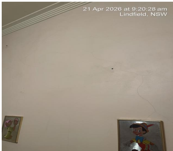
Photo 81 - Cracking observed to wall
