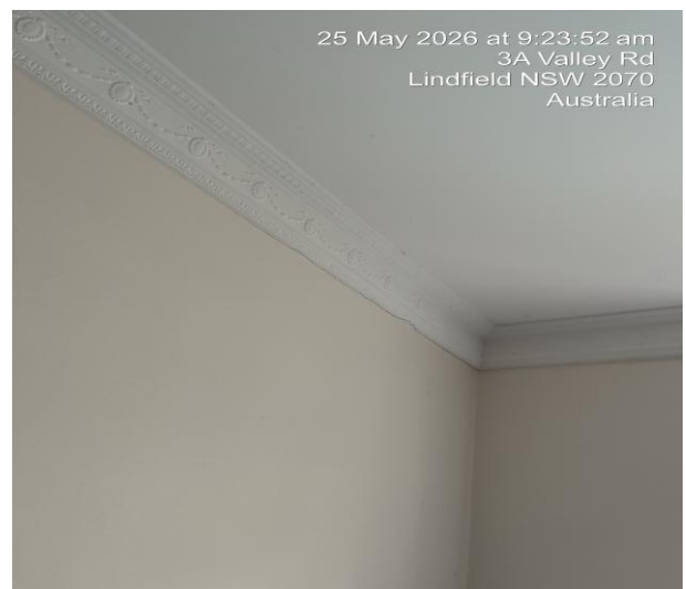
Photo 36 – Cracking observed to coving
