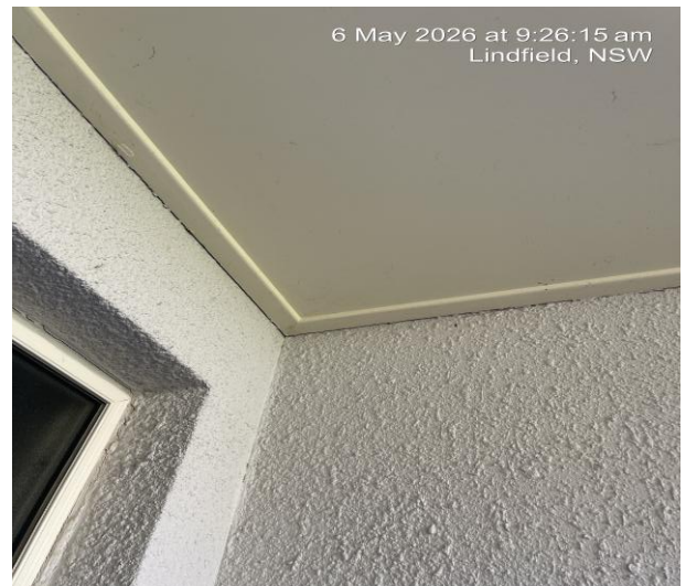
Photo 100 – Movement observed to wall/ceiling junction
