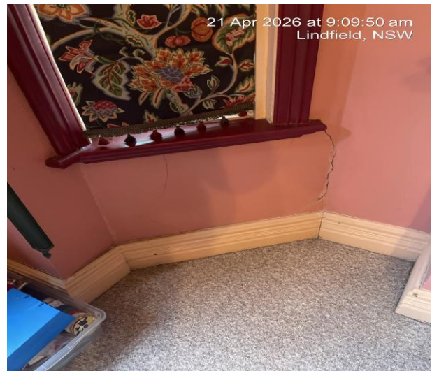
Photo 10 – Vertical cracking observed to wall
