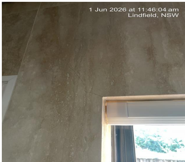
Photo 57 – Cracking observed to tiles
