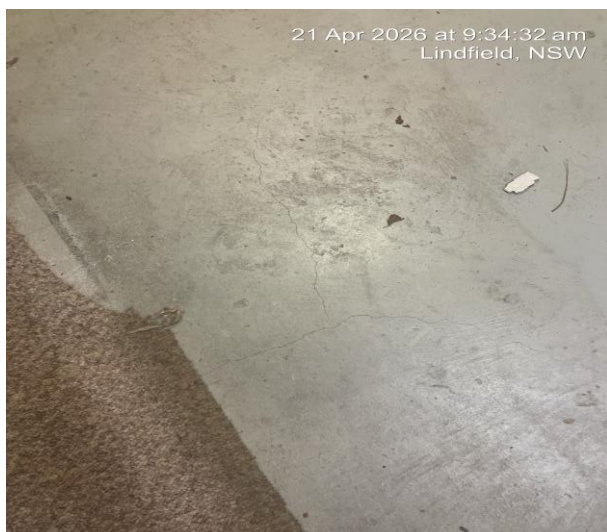
Photo 131 - Cracking observed to concrete
