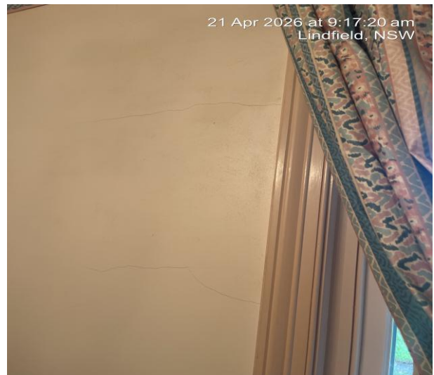
Photo 58 – Horizontal cracking observed to wall
