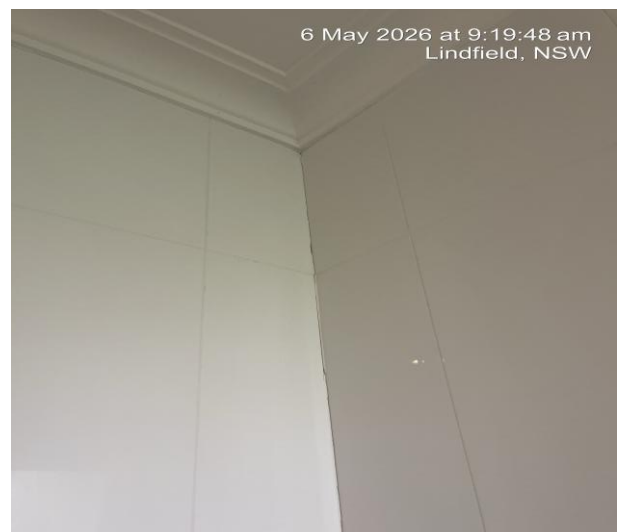
Photo 66 - Cracking observed to grout and coving
