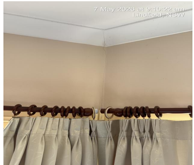
Photo 32 – Cracking observed to wall and coving
