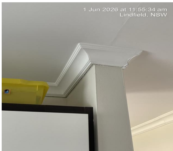
Photo 125 – Movement observed to coving
