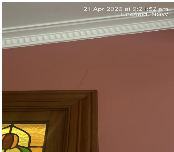
Photo 87 - Cracking observed to wall
