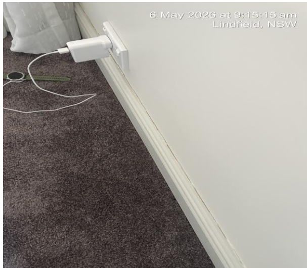
Photo 43 – Cracking observed to skirting
