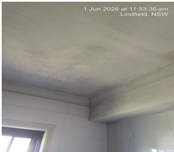
Photo 105 – Mould growth observed to ceiling
