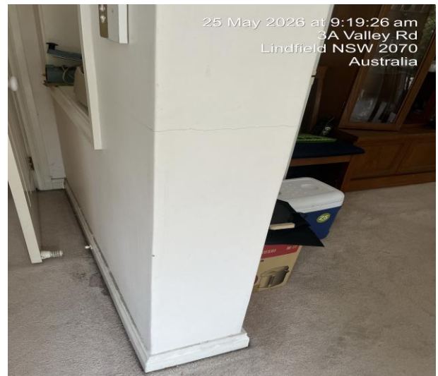
Photo 10 – Cracking observed to wall
