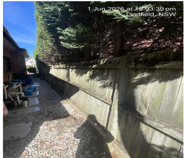
Photo 158 – Overturning of fence observed
