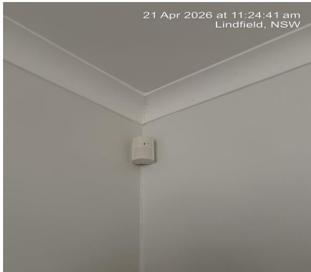
Photo 61 – Vertical cracking observed to wall and coving
