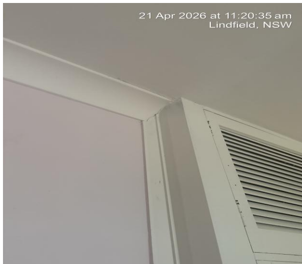
Photo 45 – Cracking observed to coving
