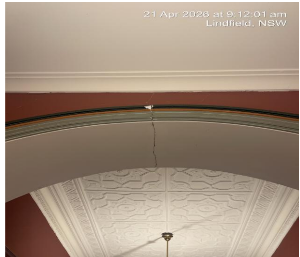
Photo 26 - Cracking observed to archway
