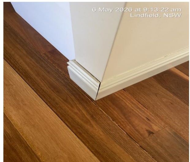
Photo 34 – Movement observed to skirting
