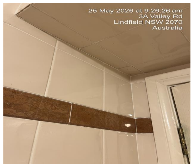
Photo 48 – Cracking observed to grout
