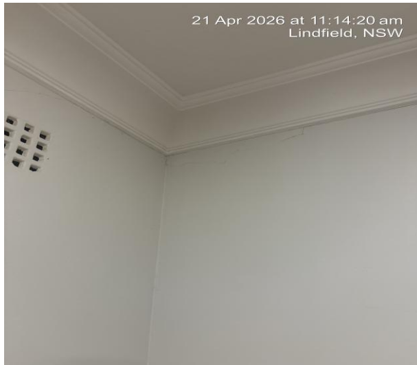
Photo 25 – Cracking observed to wall
