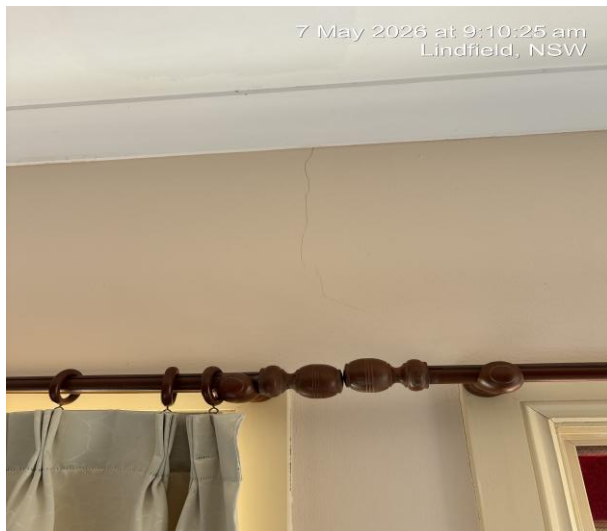
Photo 33 – Cracking observed to wall
