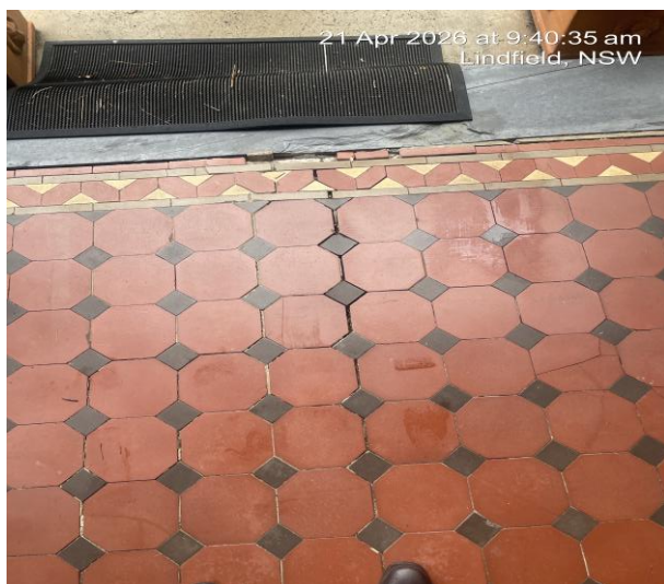
Photo 149 – Cracking observed to tiles
