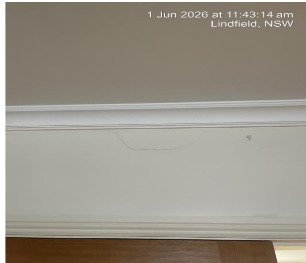
Photo 38 – Cracking observed to render
