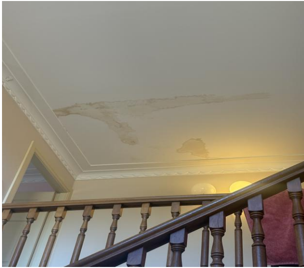
Photo 97 – Water damage observed to ceiling
