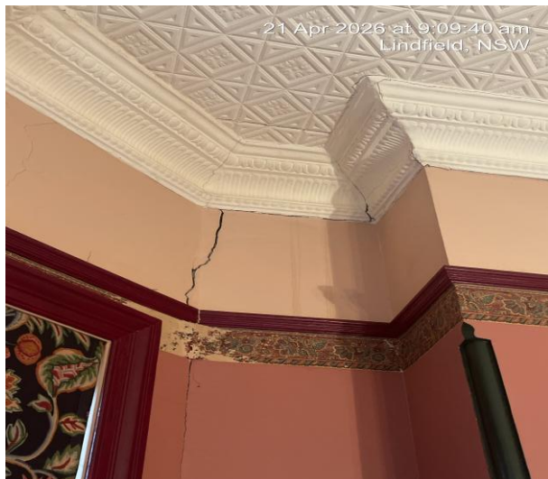
Photo 9 – Vertical cracking observed to wall and coving
