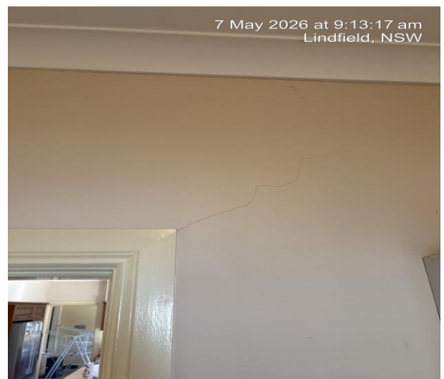
Photo 42 – Cracking observed to wall
