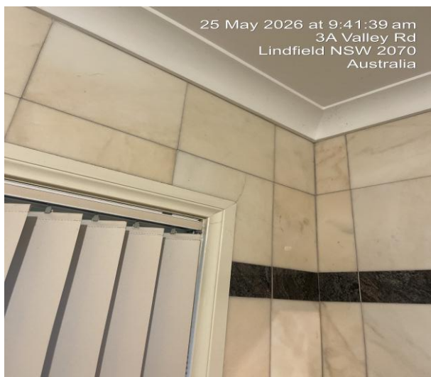
Photo 119 – Cracking observed to tiles and frame
