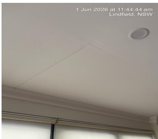
Photo 47 - Cracking observed to ceiling
