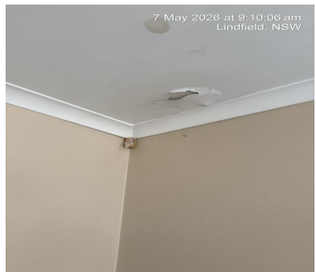
Photo 30 – Water damage observed to ceiling
