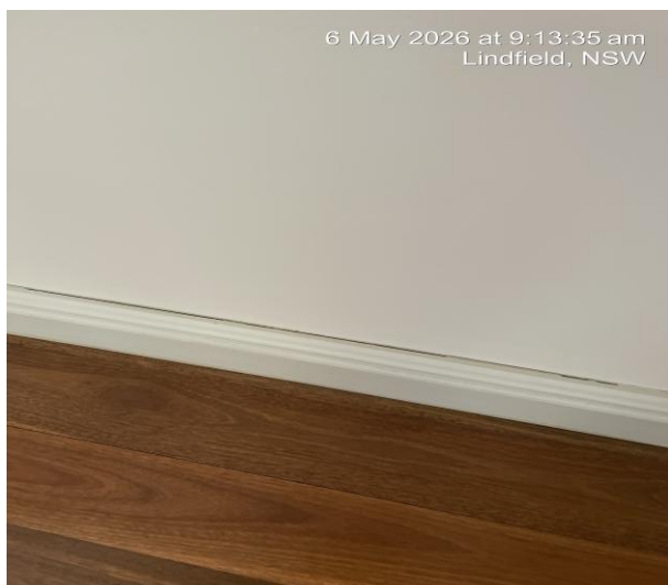
Photo 35 - Movement observed to skirting
