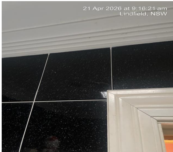
Photo 55 - Cracking observed to tile
