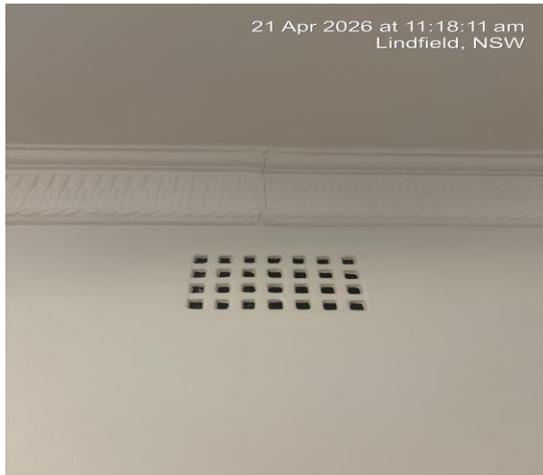
Photo 37 – Cracking observed to coving
