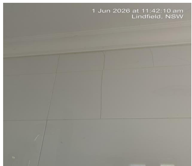
Photo 30 – Cracking observed to tiles
