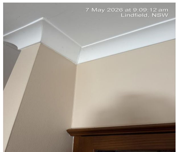
Photo 24 – Cracking observed to wall and coving
