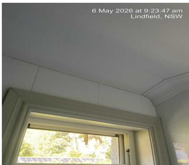
Photo 89 – Movement observed to wall/ceiling junction
