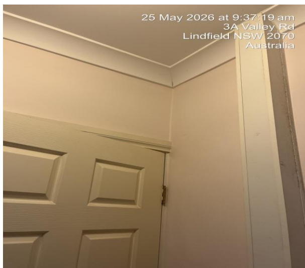
Photo 101 – Cracking observed to coving
