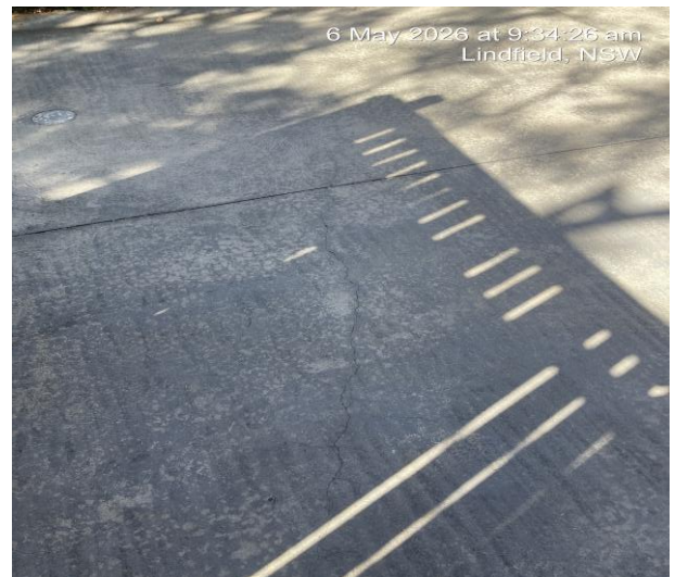
Photo 130 – Cracking observed to concrete
