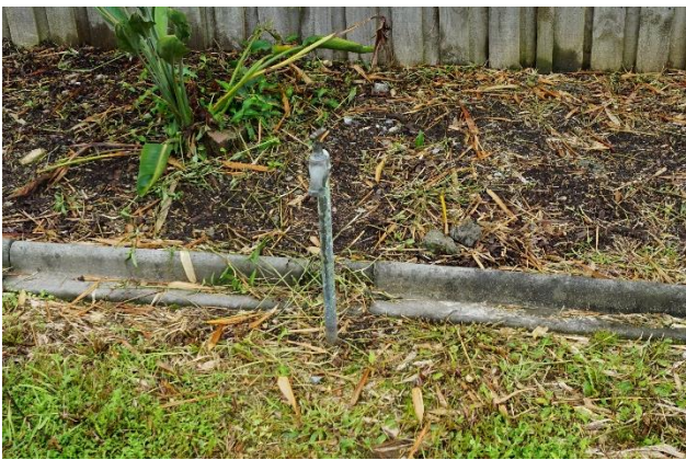
Figure 26 – Tap located in front yard at No. 4 Woodside Avenue.
