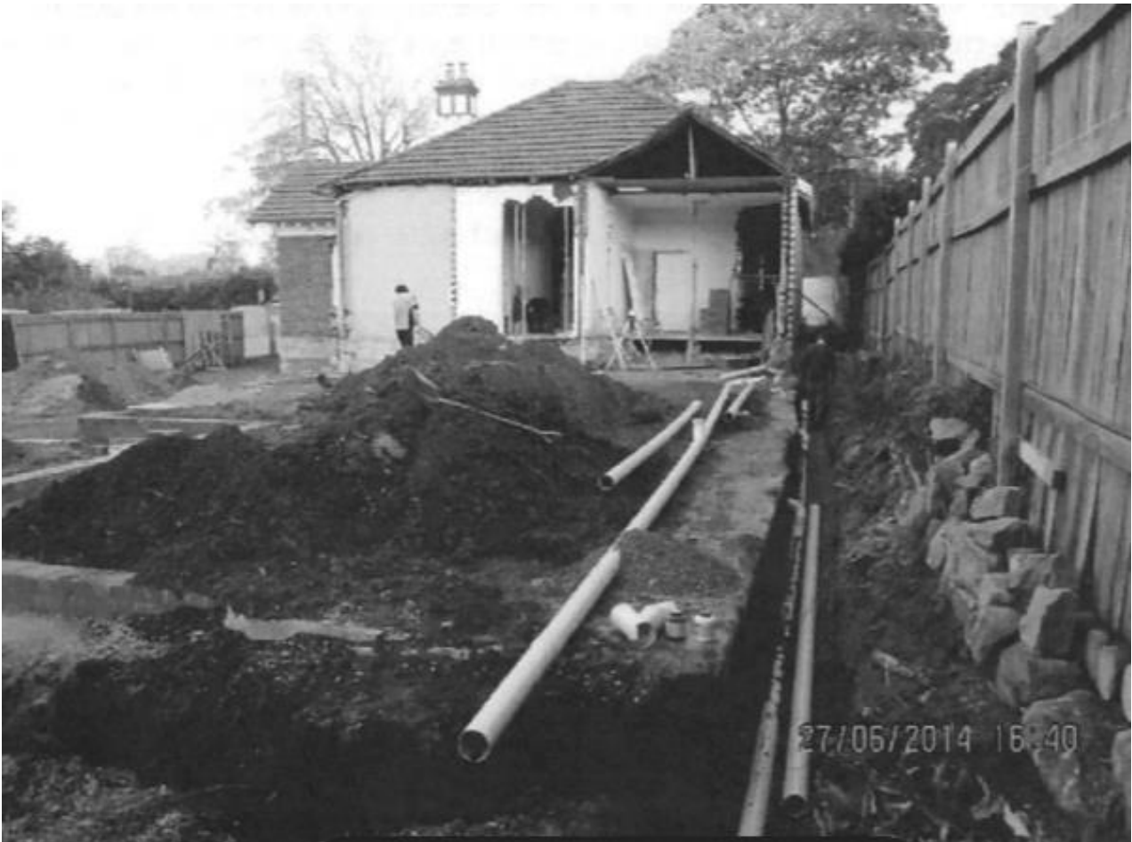
Figure 93 Photograph of dwelling during construction prior to completion of 2014 alterations and additions
