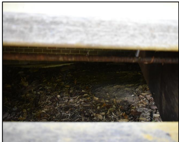
Figure 32: 20 Lord St, underneath the house.
