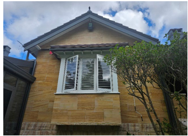
Figure 11 Front façade, showing alterations, with contemporary tiling as a decorative feature of the façade.
