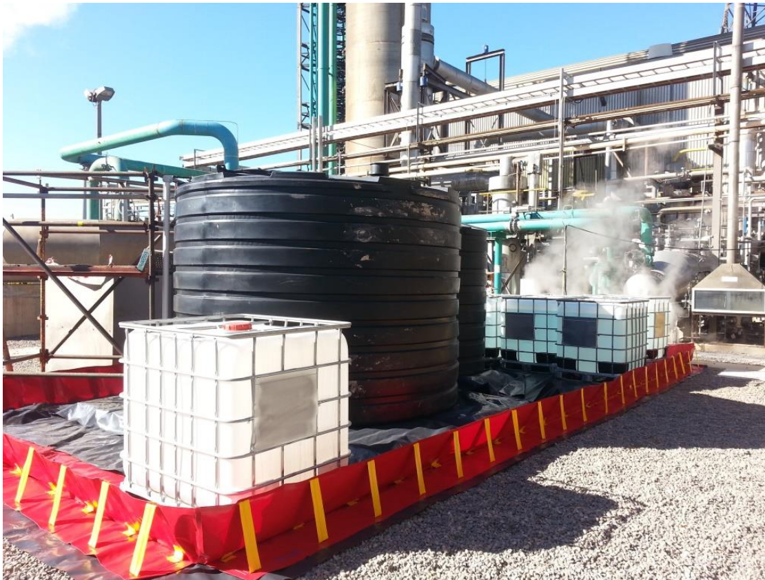
Figure 14 Temporary chemical bunding
