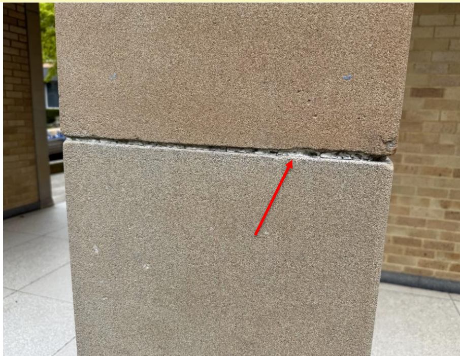
Photo 7: Asbestos containing mastic around pillars at Centenary Hall's exterior
