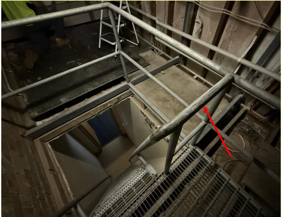
Photo 9: Grey lead containing paint on handrail, L02-L03 Ladder to plantroom
