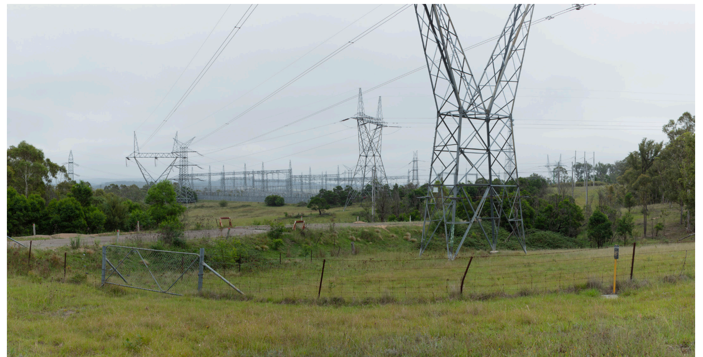
Image 08 View of Marulan Substation from Canyonleigh Road
