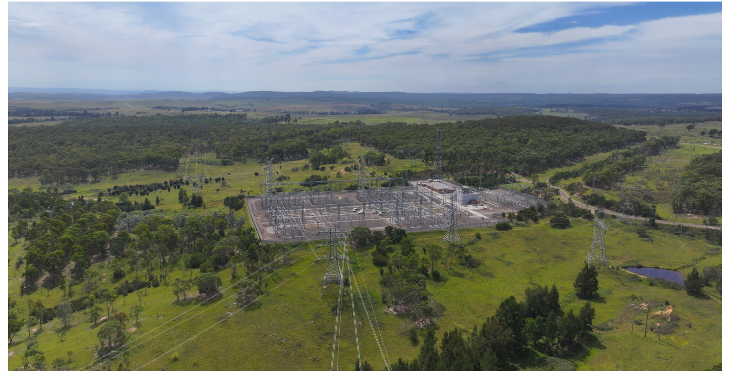
Image 03 Marulan Substation to the north of the Project
