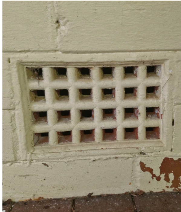
Photo 8 Inspection showing the air vents with very small openings
