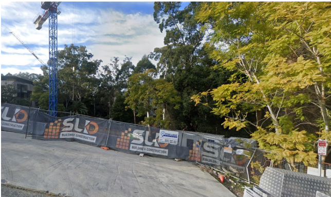
Figure 6: Sites to the south at 4A-10 Maclaurin Parade, Roseville under construction Source: Google maps
