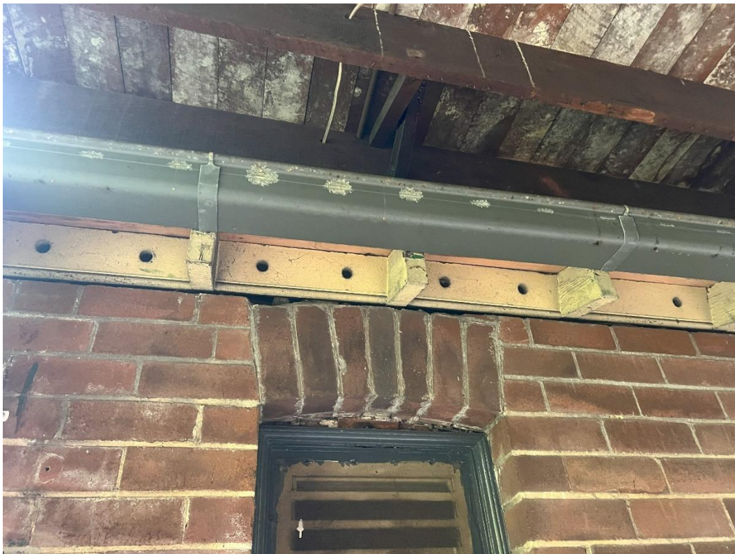
Figure 15 – possible microbat entry point (rotted timber)
