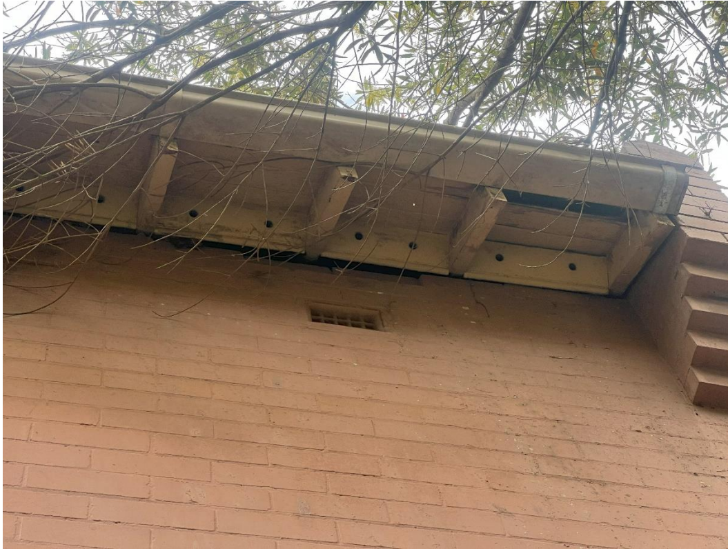
Figure 14 – possible microbat entry point (rotted eve)
