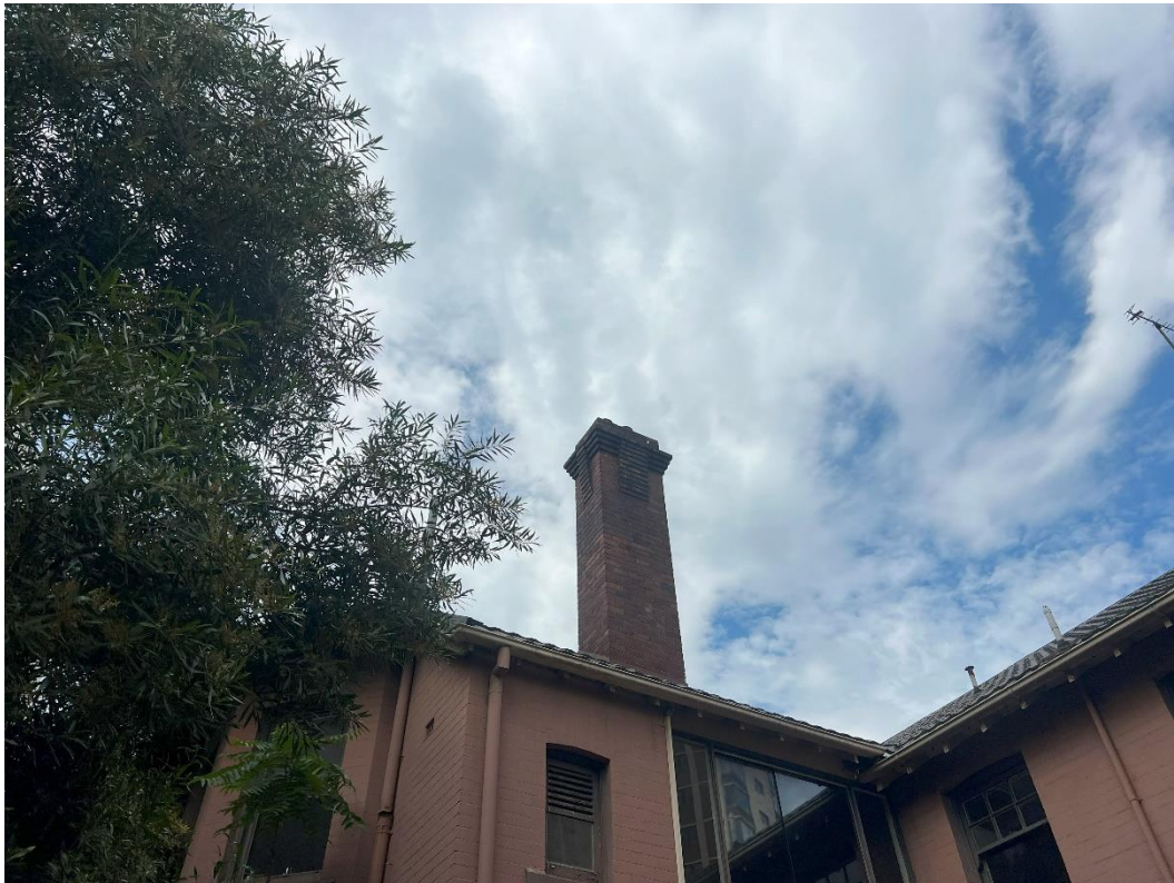
Figure 13 – possible microbat entry point (chimney)
