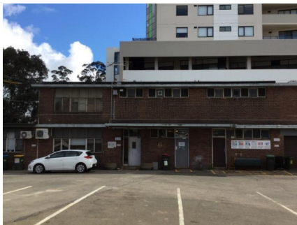
PHOTO NO.: J155653-001-PHOTO017 RESULT: ASBESTOS - PRESUMED POSITIVE BUILDING/LEVEL: MAIN BUILDING - GROUND LEVEL ROOM/LOCATION: ROOF - THROUGHOUT FEATURE/MATERIAL: ROOF COVERING - BITUMINOUS MATERIAL SAMPLE NO.: NOT SAMPLED HEIGHT RESTRICTED
