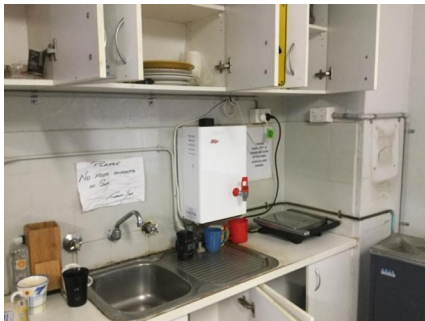
PHOTO NO.: J155653-001-PHOTO007 RESULT: SMF - PRESUMED POSITIVE BUILDING/LEVEL: MAIN BUILDING - LEVEL ONE ROOM/LOCATION: LUNCH ROOM FEATURE/MATERIAL: HOT WATER HEATER - INSULATION MATERIAL SAMPLE NO.: -
