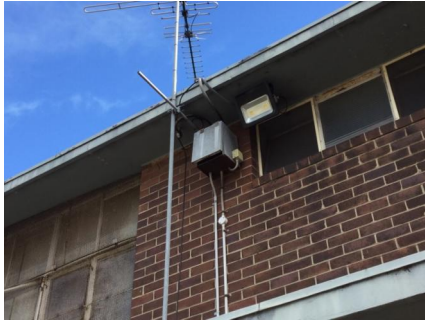
PHOTO NO.: J155653-001-PHOTO018 RESULT: ASBESTOS - PRESUMED POSITIVE BUILDING/LEVEL: MAIN BUILDING - GROUND LEVEL ROOM/LOCATION: ELECTRICAL BOX - ON UPPER WALL FEATURE/MATERIAL: ELECTRICAL - FUSE BOARD - COMPRESSED BITUMINOUS ELECTRICAL PANEL SAMPLE NO.: NOT SAMPLED HEIGHT RESTRICTED
