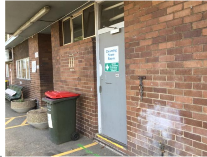
PHOTO NO.: J155653-001-PHOTO021 RESULT: LEAD (PAINT) - POSITIVE, 3.9% W/W BUILDING/LEVEL: MAIN BUILDING - GROUND LEVEL ROOM/LOCATION: EXTERNAL WINDOW FRAMES - MAIN ELEVATIONS FEATURE/MATERIAL: DOOR & FRAME - UPPER & LOWER PAINT SYSTEM/S SAMPLE NO.: J155653-001-LP-005
