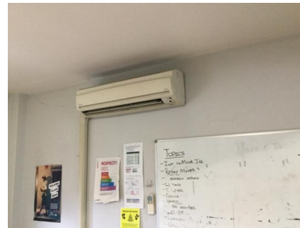
PHOTO NO.: J155653-001-PHOTO008 RESULT: ODS - PRESUMED POSITIVE BUILDING/LEVEL: MAIN BUILDING - LEVEL ONE ROOM/LOCATION: LUNCH ROOM - REAR WALL FEATURE/MATERIAL: SPLIT SYSTEM AIR CON UNIT - R401A - HCFC BLEND SAMPLE NO.: -
