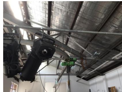
PHOTO NO.: J155653-001-PHOTO026 RESULT: SMF - PRESUMED POSITIVE BUILDING/LEVEL: MOWERS SHED - GROUND LEVEL ROOM/LOCATION: MAIN SHED - ROOF LINING FEATURE/MATERIAL: INSULATION - SARKING INSULATION SAMPLE NO.: -
