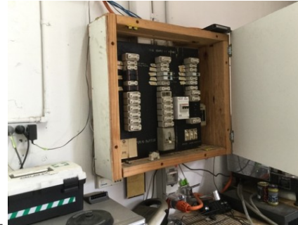
PHOTO NO.: J155653-001-PHOTO038 RESULT: ASBESTOS - PRESUMED POSITIVE BUILDING/LEVEL: MOWERS SHED - GROUND LEVEL ROOM/LOCATION: MAIN SHED - AT GIBBONS ST END FEATURE/MATERIAL: ELECTRICAL DISTRIBUTION BOARD - COMPRESSED BITUMINOUS ELECTRICAL PANEL SAMPLE NO.: SIMILAR TO: J155653-001-004
