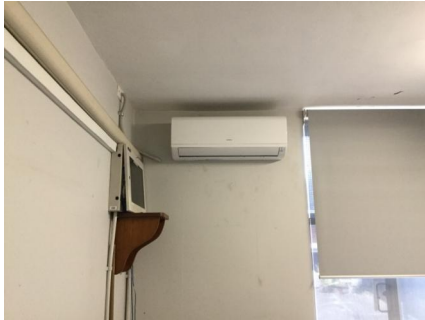
PHOTO NO.: J155653-001-PHOTO019 RESULT: ODS - PRESUMED POSITIVE BUILDING/LEVEL: MAIN BUILDING - GROUND LEVEL ROOM/LOCATION: OFFICE - FRONT WALL FEATURE/MATERIAL: SPLIT SYSTEM AIR CON UNIT - R401A - HCFC BLEND SAMPLE NO.: -
