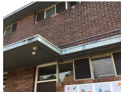
PHOTO NO.: J155653-001-PHOTO022 RESULT: LEAD (PAINT) - PRESUMED POSITIVE BUILDING/LEVEL: MAIN BUILDING - GROUND LEVEL ROOM/LOCATION: SOFFIT - MAIN ELEVATIONS FEATURE/MATERIAL: BULKHEAD - UPPER & LOWER PAINT SYSTEM/S SAMPLE NO.: NOT SAMPLED HEIGHT RESTRICTED
