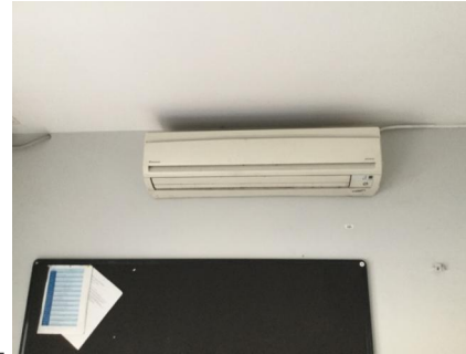
PHOTO NO.: J155653-001-PHOTO015 RESULT: ODS - PRESUMED POSITIVE BUILDING/LEVEL: MAIN BUILDING - GROUND LEVEL ROOM/LOCATION: TEAM LEADERS OFFICE - REAR WALL FEATURE/MATERIAL: SPLIT SYSTEM AIR CON UNIT - R401A - HCFC BLEND SAMPLE NO.: -
