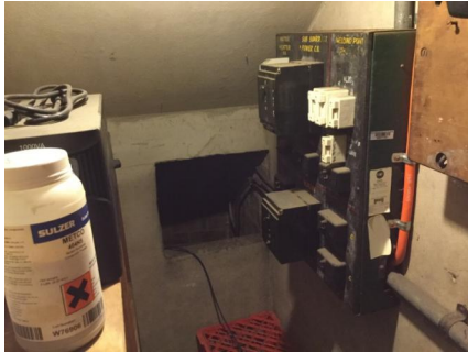
PHOTO NO.: J155653-001-PHOTO036 RESULT: ASBESTOS - POSITIVE BUILDING/LEVEL: MOWERS SHED - GROUND LEVEL ROOM/LOCATION: BELOW STAIRS - ADJACENT OUTSIDE WALL FEATURE/MATERIAL: ELECTRICAL - FUSE BOARD - BITUMINOUS MATERIAL SAMPLE NO.: J155653-001-004
