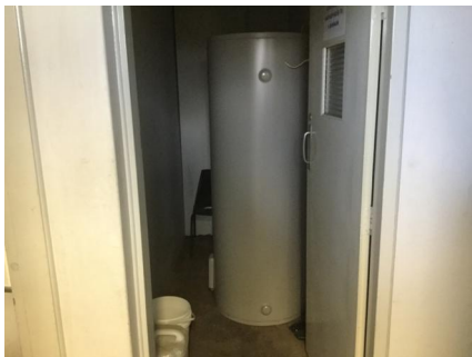
PHOTO NO.: J155653-001-PHOTO003 RESULT: SMF - PRESUMED POSITIVE BUILDING/LEVEL: MAIN BUILDING - LEVEL ONE ROOM/LOCATION: UTILITY ROOM - THROUGHOUT FEATURE/MATERIAL: HOT WATER HEATER - INSULATION MATERIAL SAMPLE NO.: -
