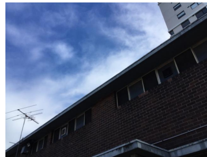
PHOTO NO.: J155653-001-PHOTO023 RESULT: LEAD (PAINT) - PRESUMED POSITIVE BUILDING/LEVEL: MAIN BUILDING - ROOF ROOM/LOCATION: ROOF - MAIN ELEVATIONS FEATURE/MATERIAL: FASCIA - UPPER & LOWER PAINT SYSTEM/S SAMPLE NO.: NOT SAMPLED HEIGHT RESTRICTED
