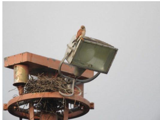
Figure 12. Poorly designed lighting is often used by raptors to establish nests.
